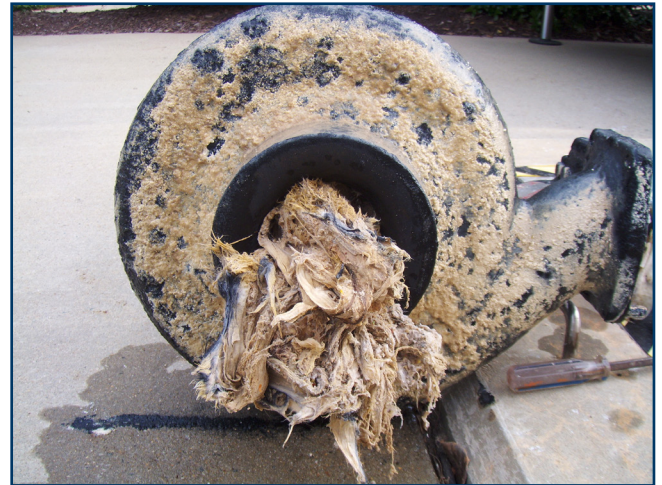
Sewer pump clogged with “flushable” wipes.
