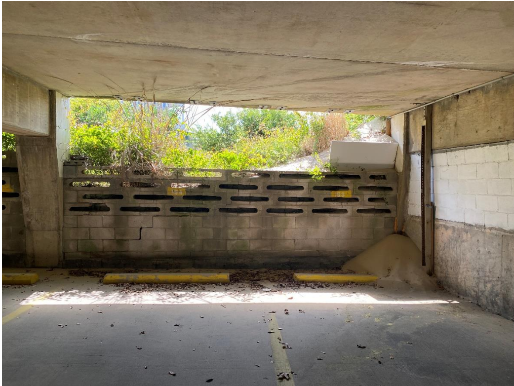
Photo 1: Coastal sand dune encroaching into northwestern corner of parking garage at Chesapeake House on the Bay
