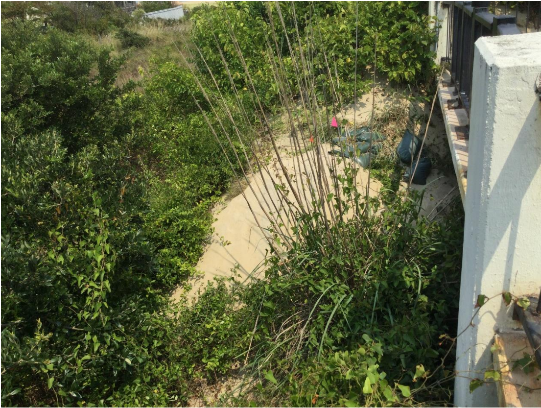
Photo 5: View of sand dune encroachment into first level of parking garage taken from second level of parking garage at Chesapeake House on the Bay
