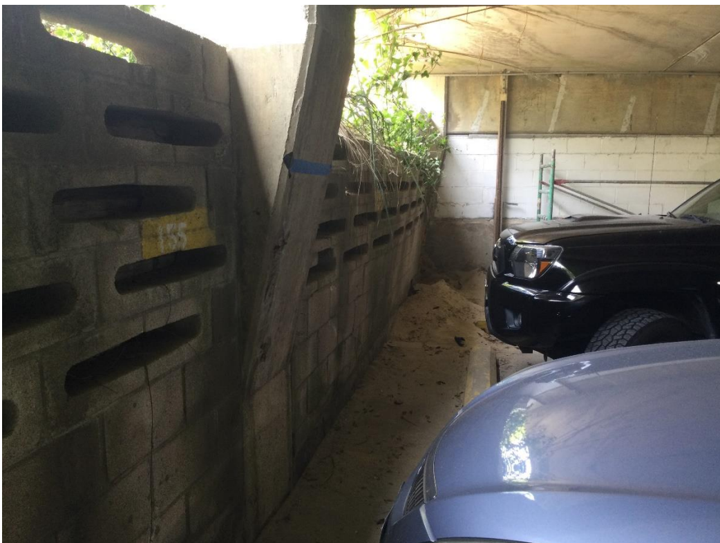
Photo 2: Damage to parking garage wall cause by coastal sand dune at Chesapeake House on the Bay
