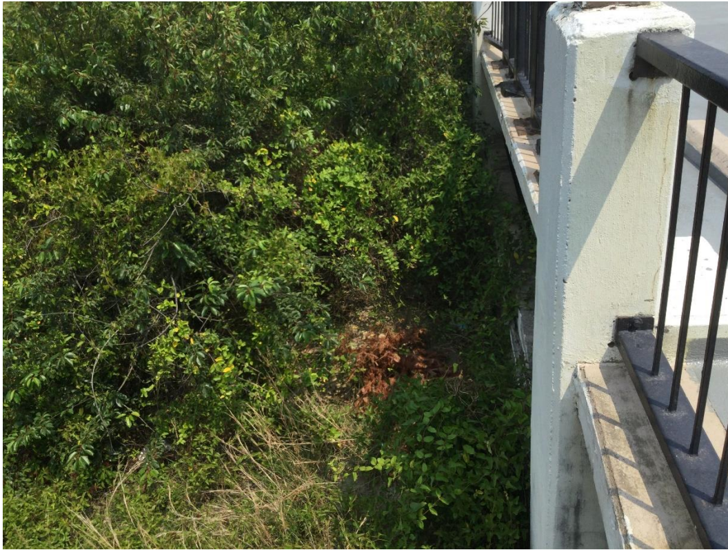
Photo 3: View of sand dune encroachment into first level of parking garage taken from second level of parking garage at Chesapeake House on the Bay
