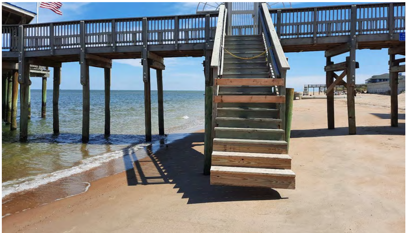
Photo 1. View of the stair case at low tide on May 5, 2021.
