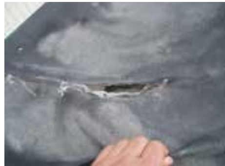
LEFT: A PUNCTURE IN THE ROOF.
