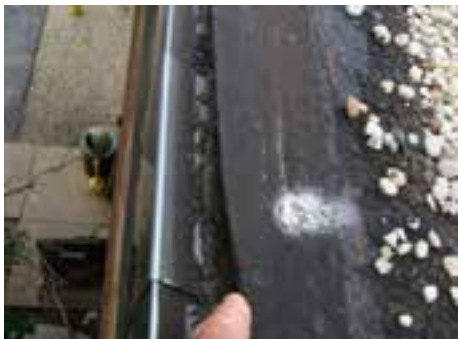
ROOF HAS PULLED FROM THE STRUCTURE.
