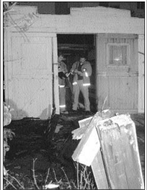
Andrew H. Fixmer/Daily Press Santa Monica Fire Department firefighters survey damage in the garage next to a home that caught on fire Tuesday. Contents of the garage lie charred in the front.
