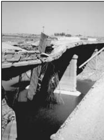
Kelly Hayes-Raitt/Special to the Daily Press A truck has fallen through a collapsed bridge on the only highway between Baghdad and Basra. The bombed bridge remains unrepaired for four months after the war.
