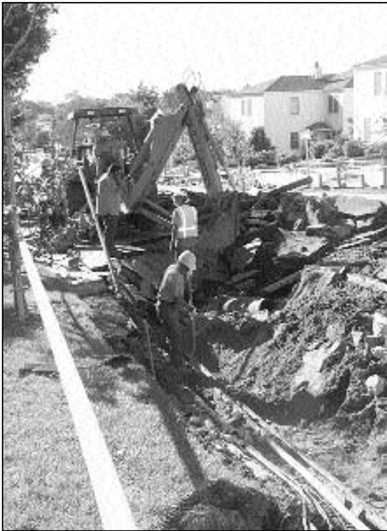
Crews remove the debris from the giant sinkhole that collapsed on Ocean Park Boulevard.
