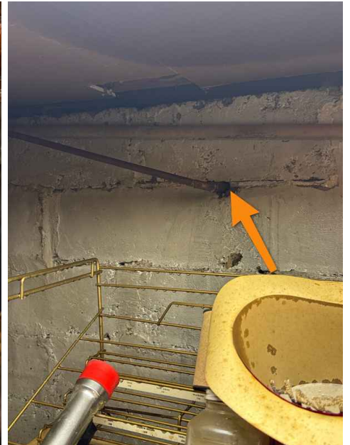
Northwest Basement hosebib
