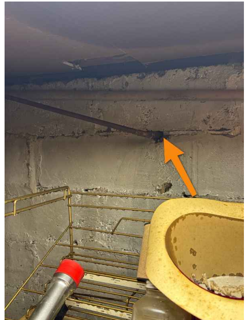
Northwest Basement hosebib
