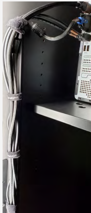
Vertical cable management detail.
