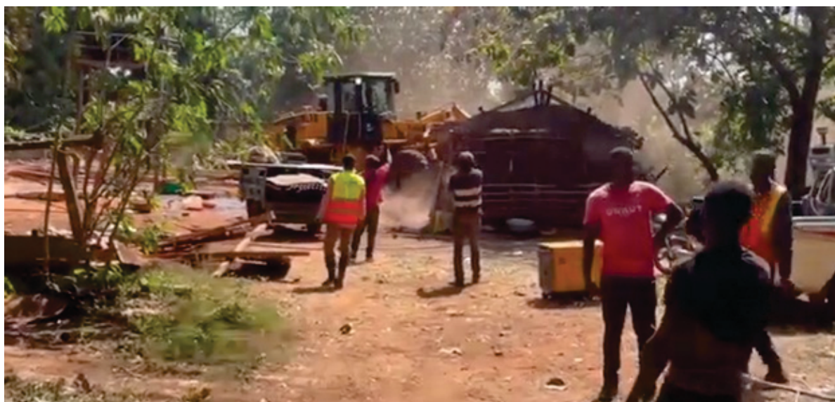
Fig. 7: Destruction of properties on affected respondents' properties.
