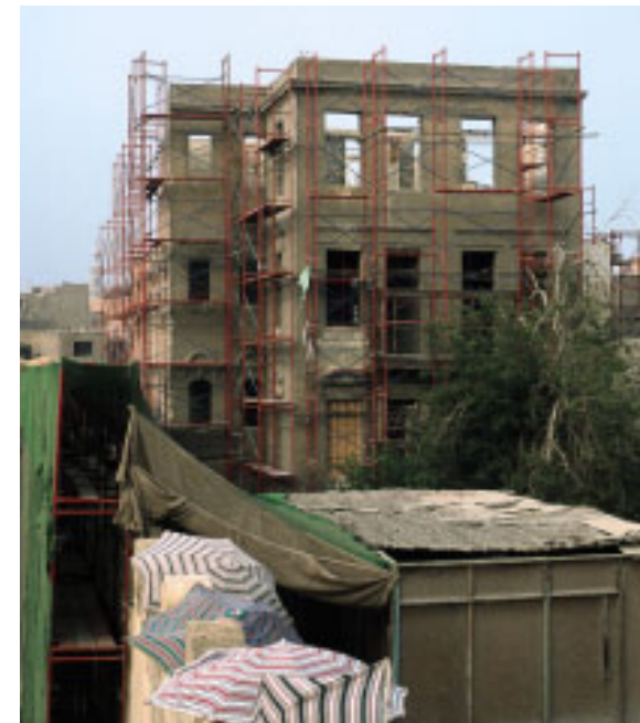
Rehabilitation of the former Darb Shouglan School, seen here in its early stages, offered an opportunity to introduce a community centre into a context that sorely lacked public facilities.
