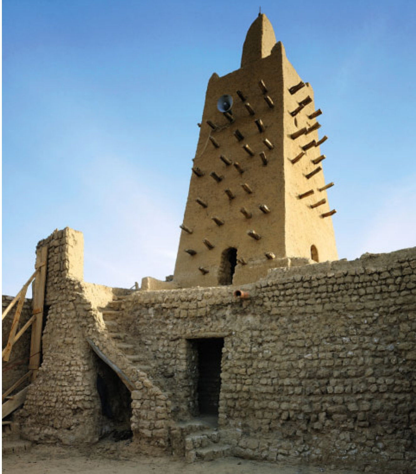
A minaret of Djingareyber Mosque after restoration. The Mosque was built in mud and tuff stone, evident in the foreground of the shot.
