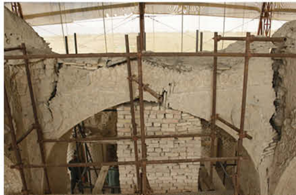
A temporary masonry wall built beneath the damaged arch to prevent collapse, AKTC, 2009
