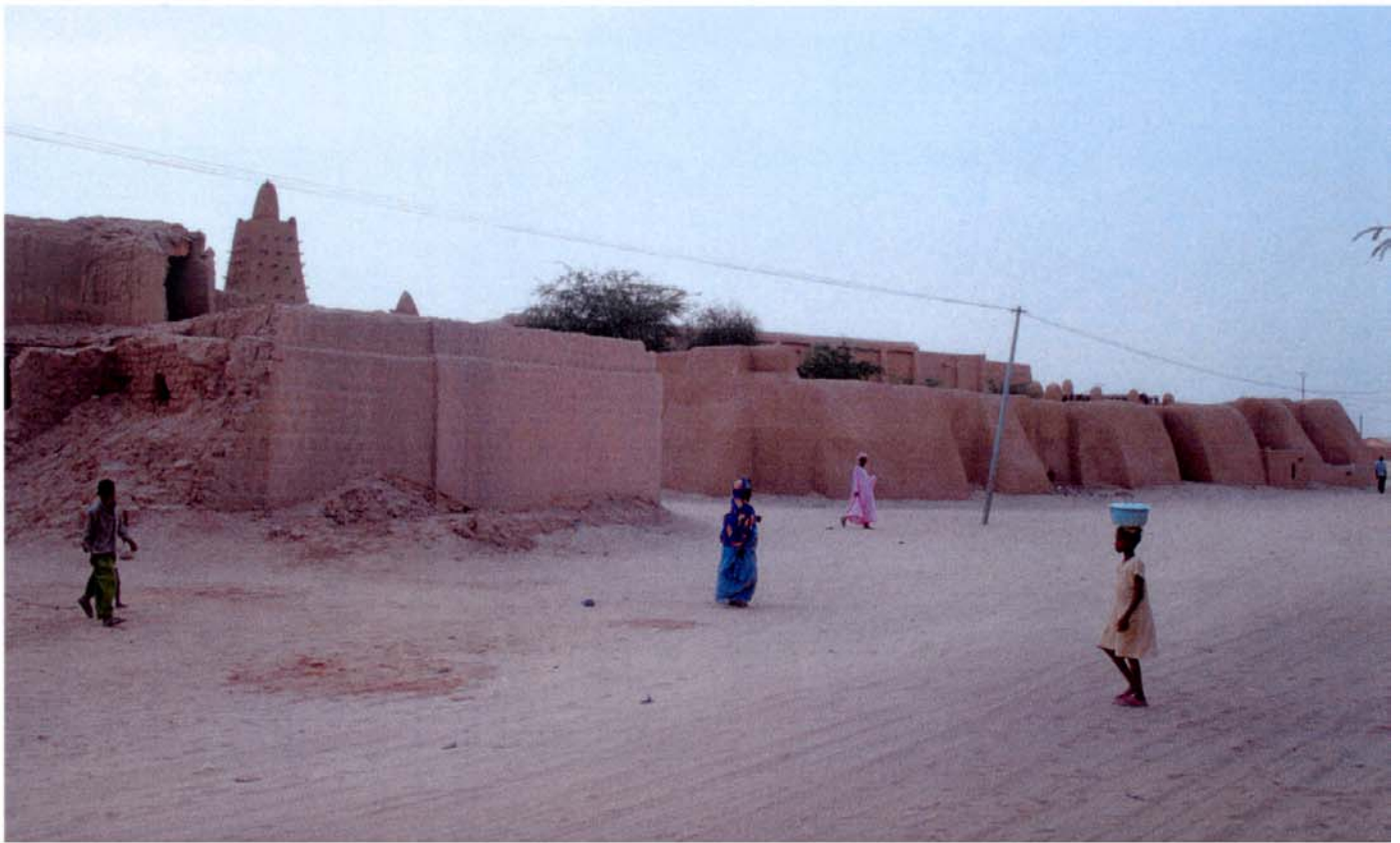
Above: Deteriorating mud constructions near the mosque.
