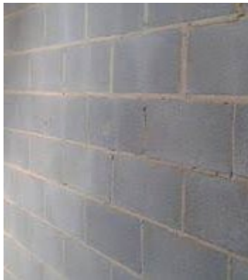
Figure 2 Unfinished block is not acceptable.
