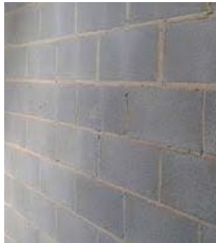
Figure 3 Unfinished block is not acceptable.
