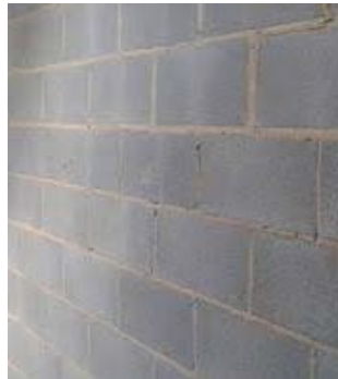
Figure 3. Unfinished block is not acceptable.
