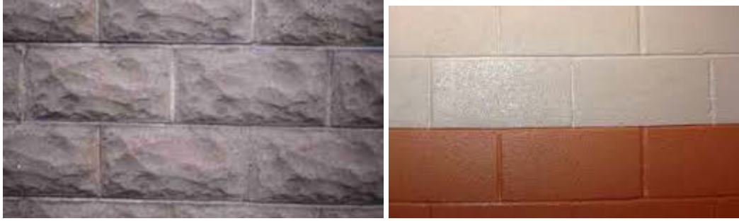
Figure 2. Finished concrete block is acceptable.
