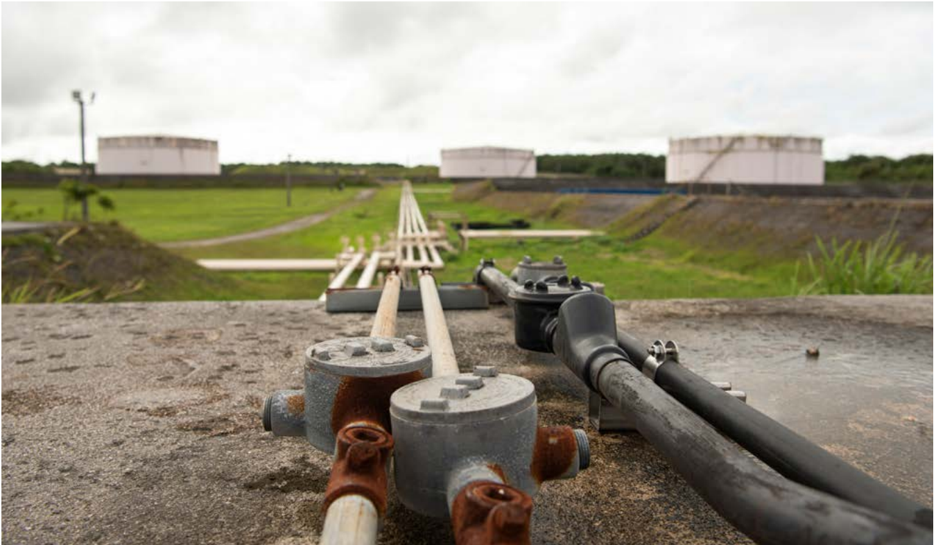
This electrical conduit powers fuel tanks on Guam holding almost 30 million gallons of fuel. It represents the type of infrastructure that should be hardened or made more resilient by building in redundancy. (Aubree Owens/U.S. Air Force)
