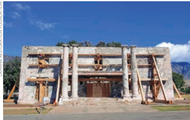
The Old Lahaina Courthouse, built in the 1850s by the Kingdom of Hawaii, is one of nine historic buildings owned or managed by the Lahaina Restoration Foundation that were severely damaged or destroyed during the 2023 Lahaina wildfire disaster.
