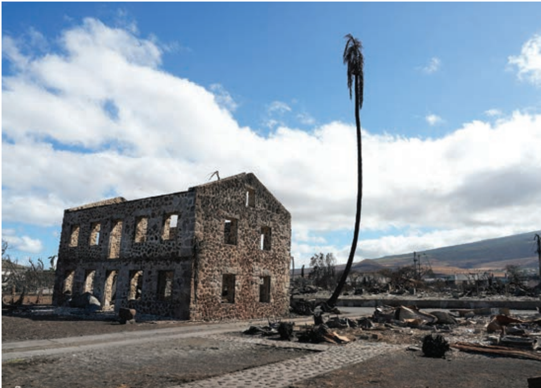
Fire-damaged remains of the U.S. Seamen's Hospital (U.S. Marine Hospital) in Lahaina Historic District.
