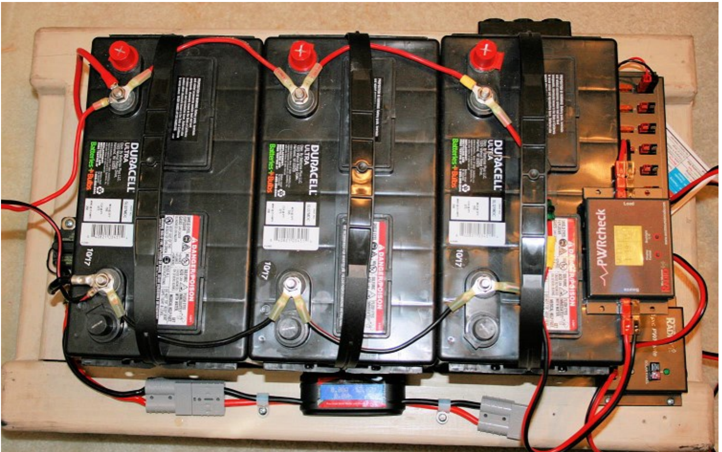
Figure 17: Top View of Battery Pack
