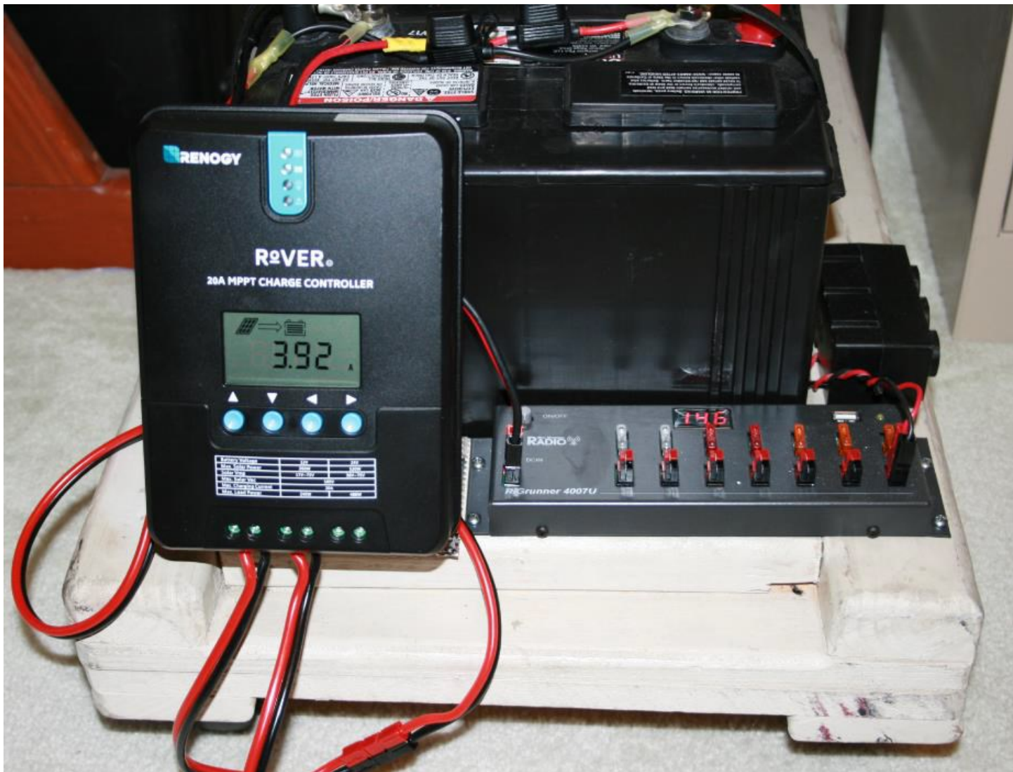
Figure 20: Renogy Rover 20A Battery Pack Instrumentation
