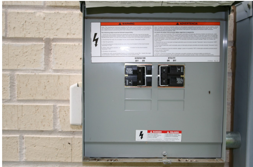
Figure 3: DPDT Manual Transfer Switch with Cover Open A schematic diagram, Figure 4, shows the connection of this manual residential transfer switch to my house wiring.
