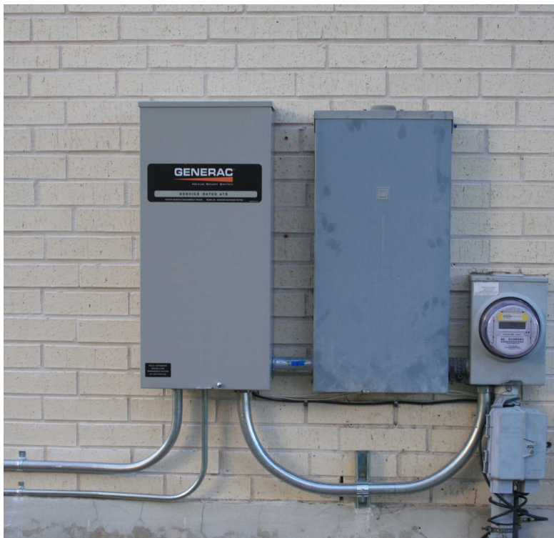
Figure 5:200A Automatic Transfer Switch
