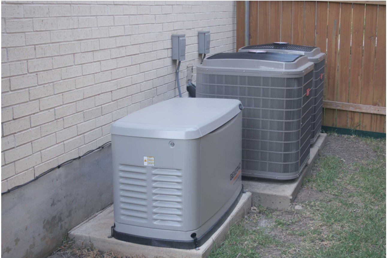
Figure 7: Residential 20KW Natural Gas/Propane Generator
