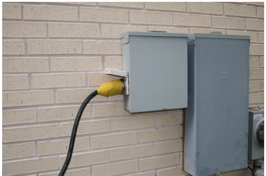
Figure 2: 10 KW Manual Transfer Switch
