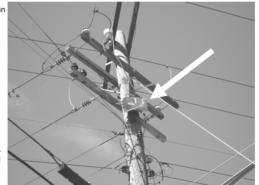
A TYPICAL CORINEX BPL INSTALLATION IN THE AUSTIN BPL TEST.
