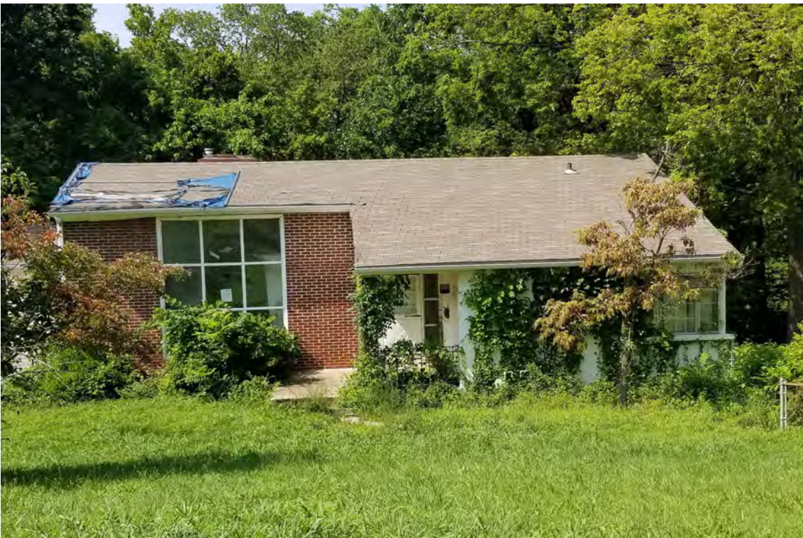
Dilapidation (Fox Woods)
