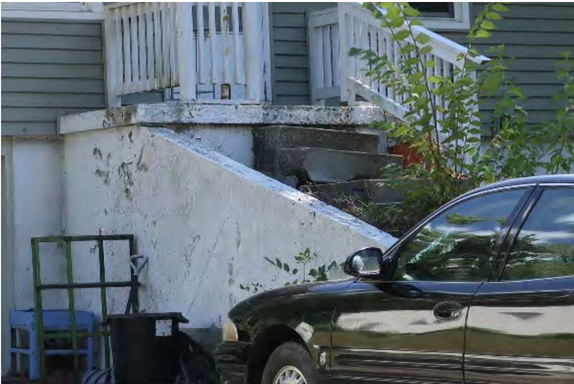
Deteriorating Steps / Porch / Retaining Wall (Edgewood Acres)
