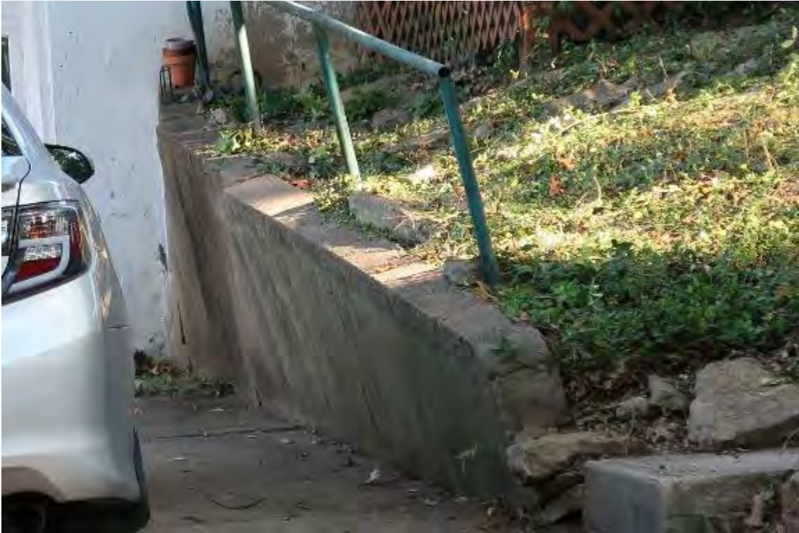
Failing Retaining Wall
