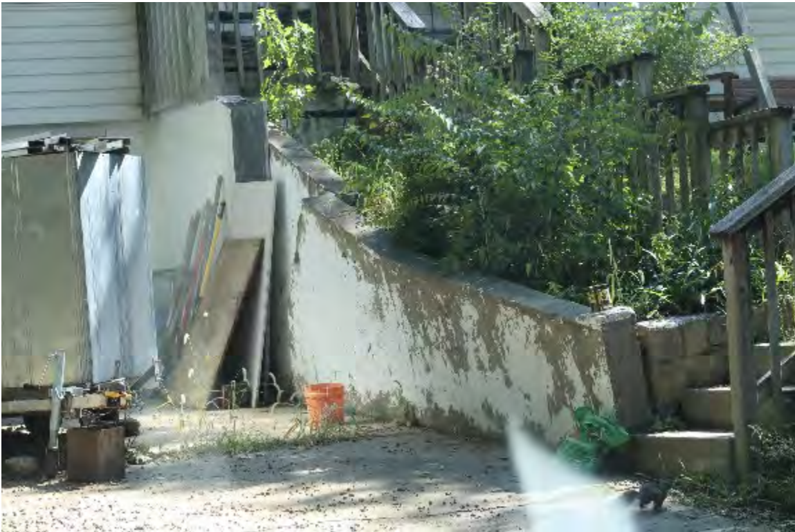
Failing / Leaning Retaining Walls & Deteriorated Driveway (Edgewood Acres)
