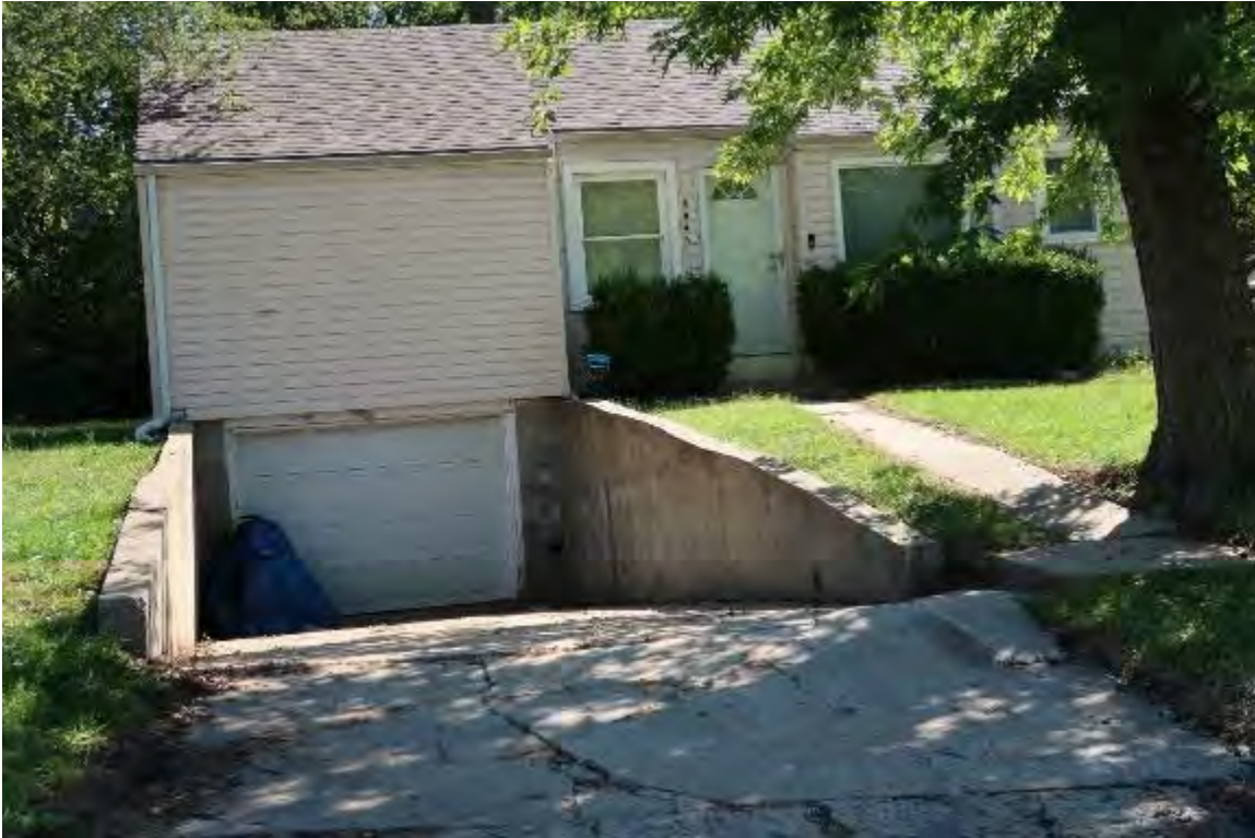
Unsecured Retaining Wall
