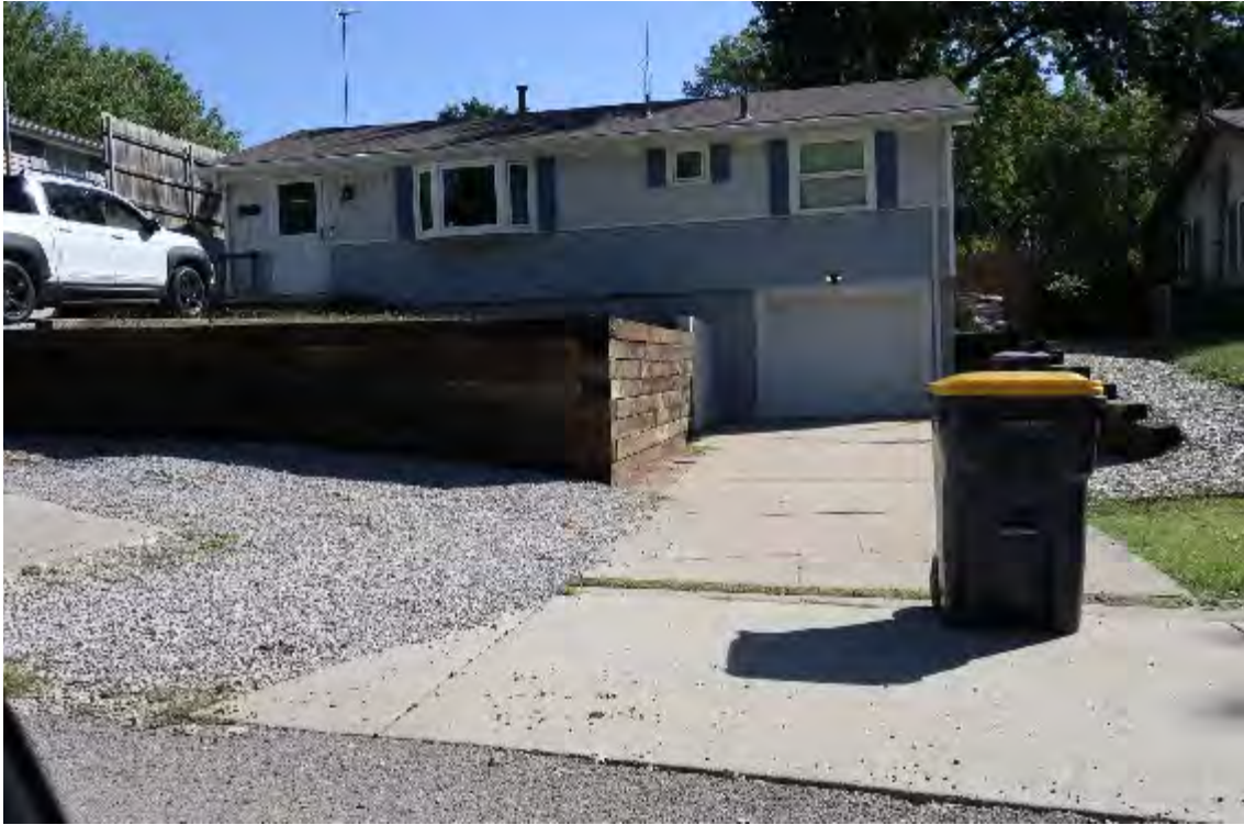
Unsecured Retaining Wall
