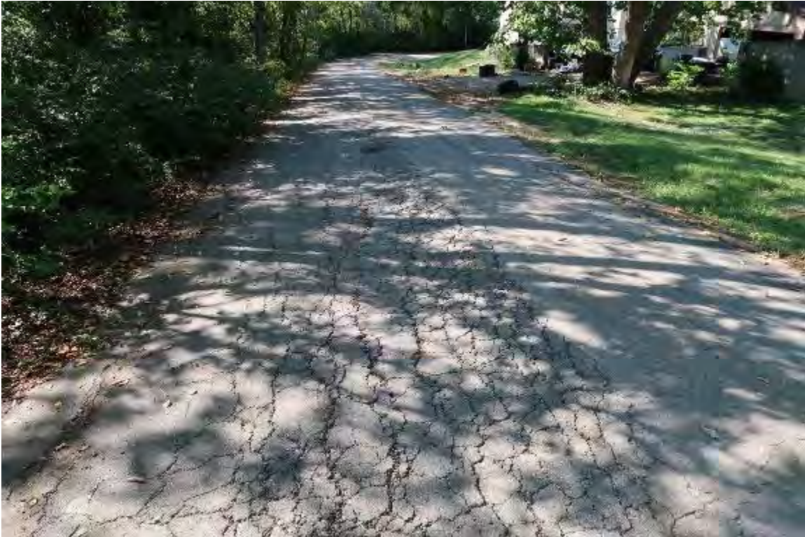
Narrow & Damaged Roadway Lacking Curbs, Gutters, & Pedestrian Sidewalks (Golden Oaks)
