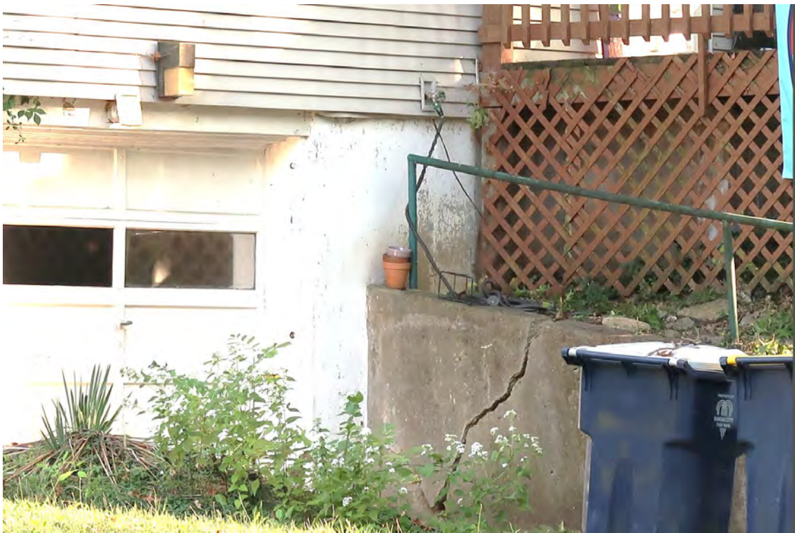
Failing Retaining Wall
