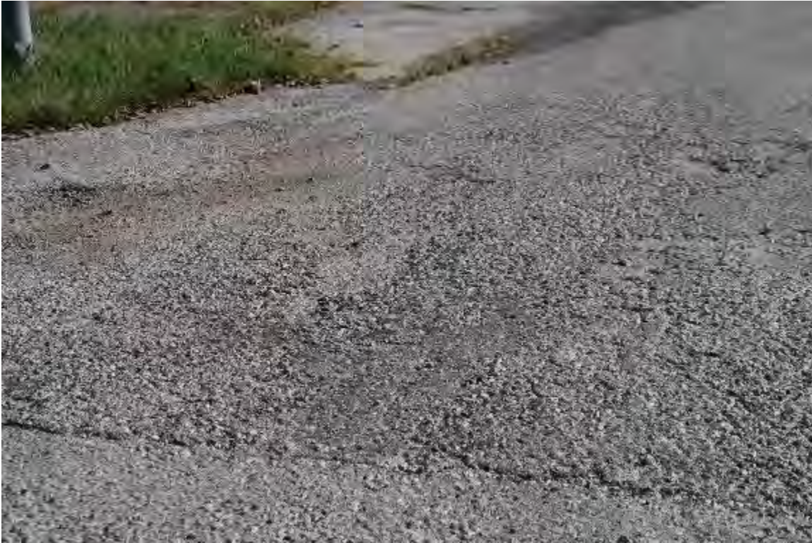
Damaged Roadway (Fox Woods)
