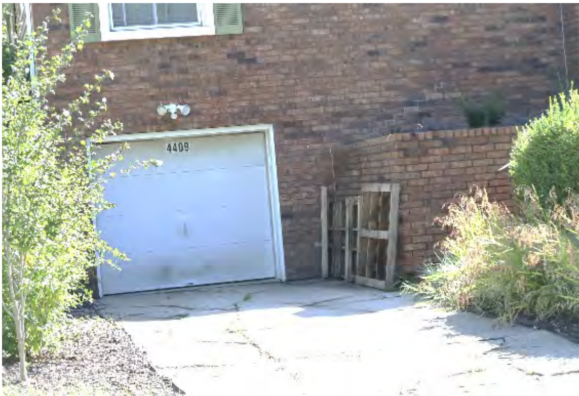
Unsecured Retaining Wall
