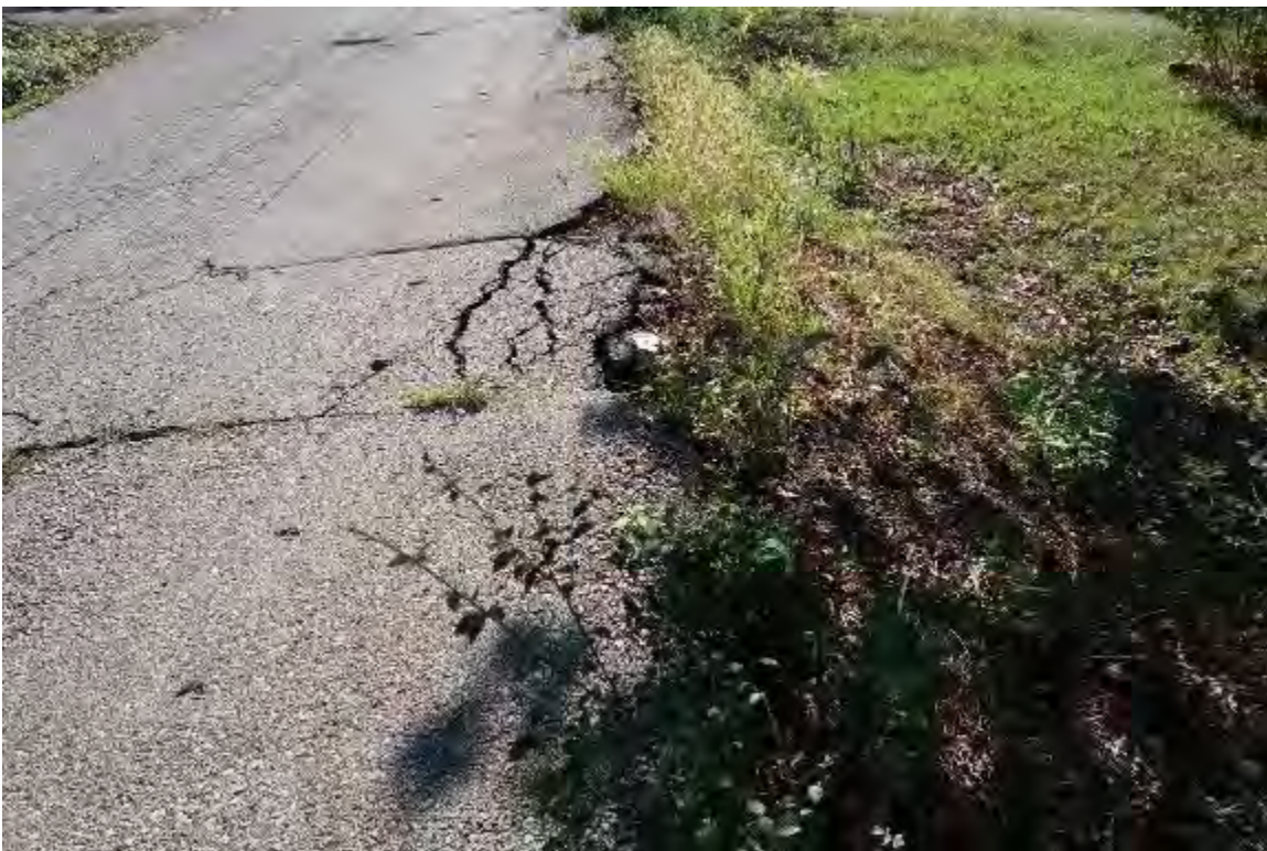
Damaged Roadway (Fox Woods)
