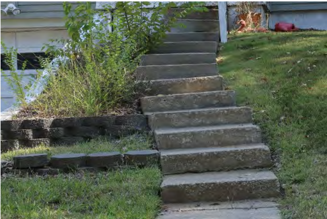
Deteriorating Steps (Edgewood Acres)
