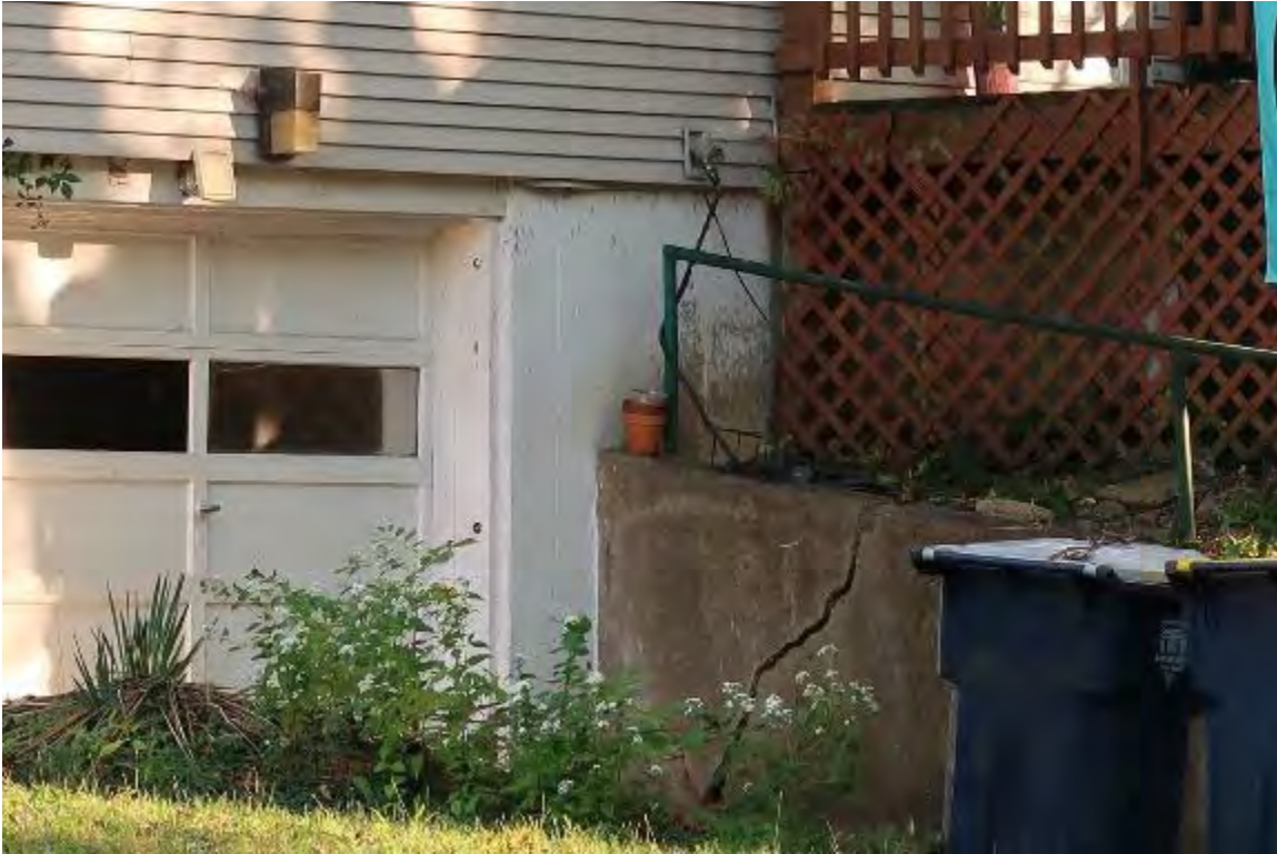
Failing Retaining Wall
