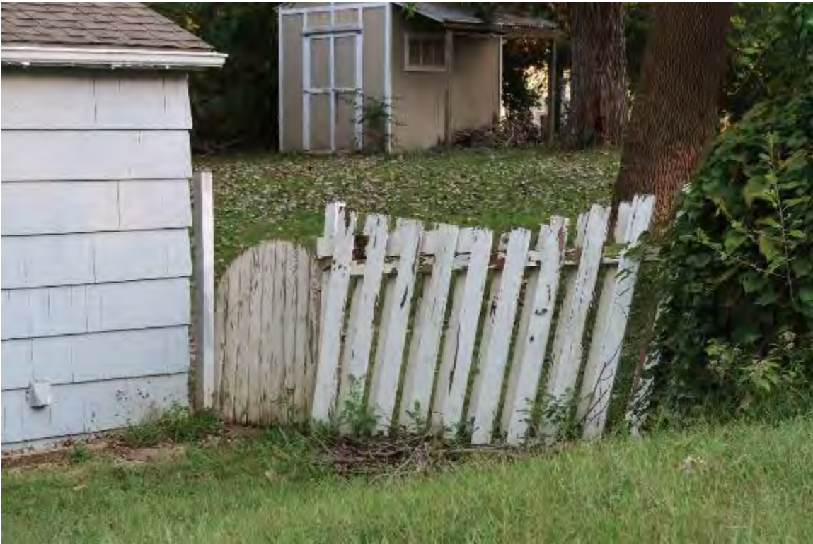
Deteriorating Fencing (Kelsey Park)
