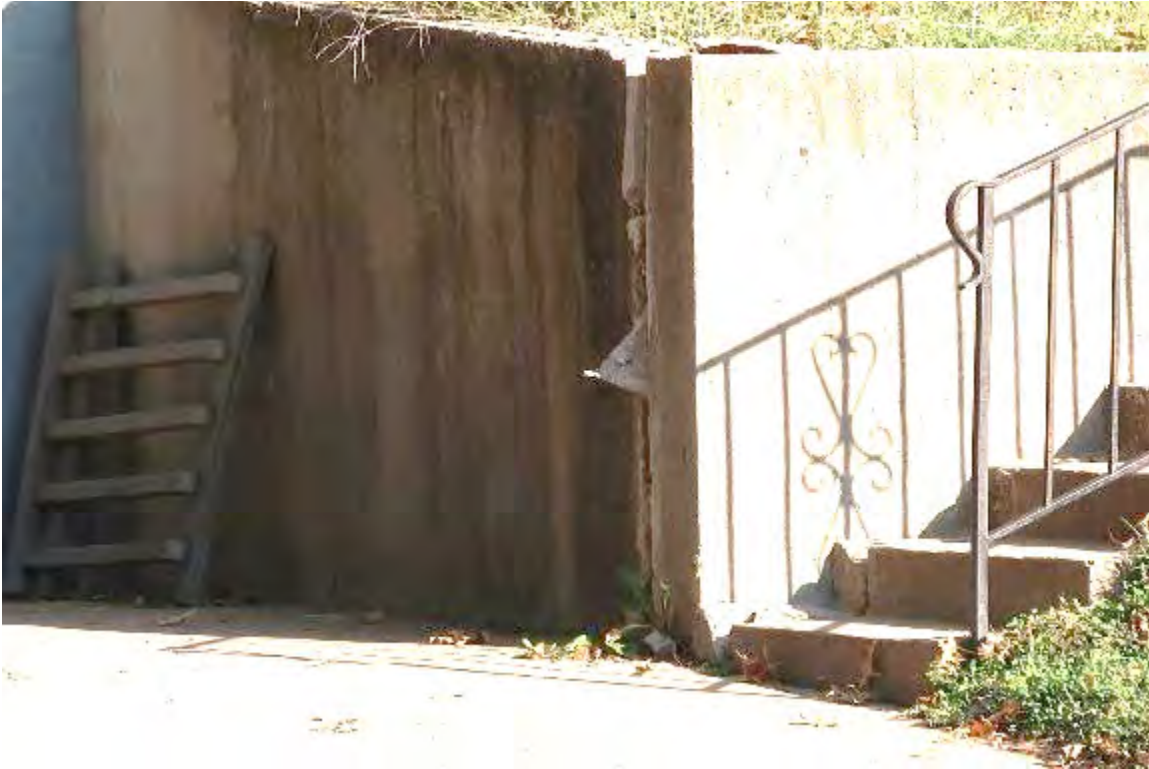
Failing / Unsecured Retaining Wall
