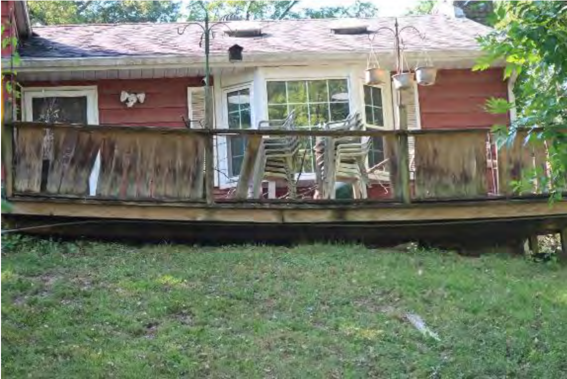
Deteriorating & Unsafe Decking (Golden Oaks)
