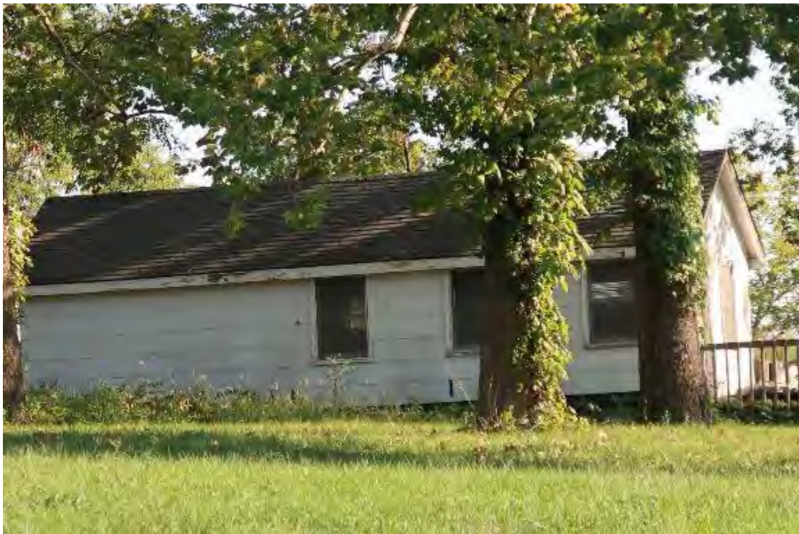
Dilapidation (Brookwood Heights)
