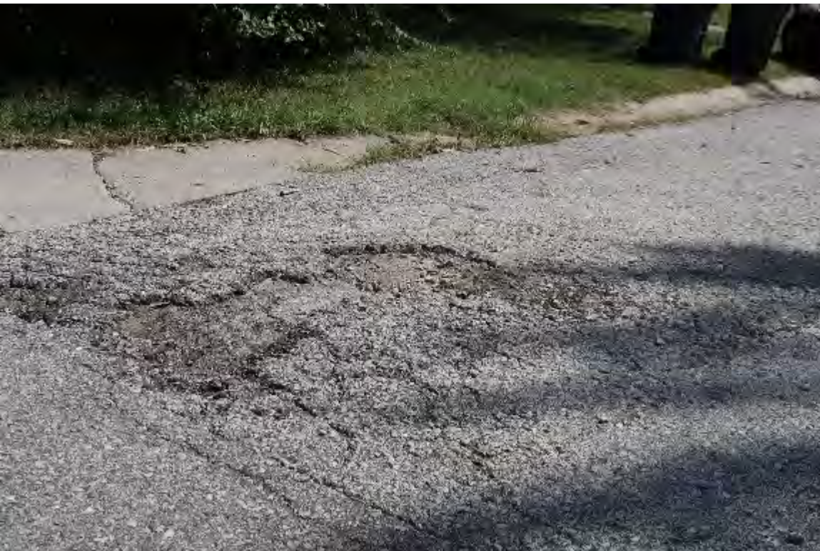
Damaged Roadway (Edgewood Acres)
