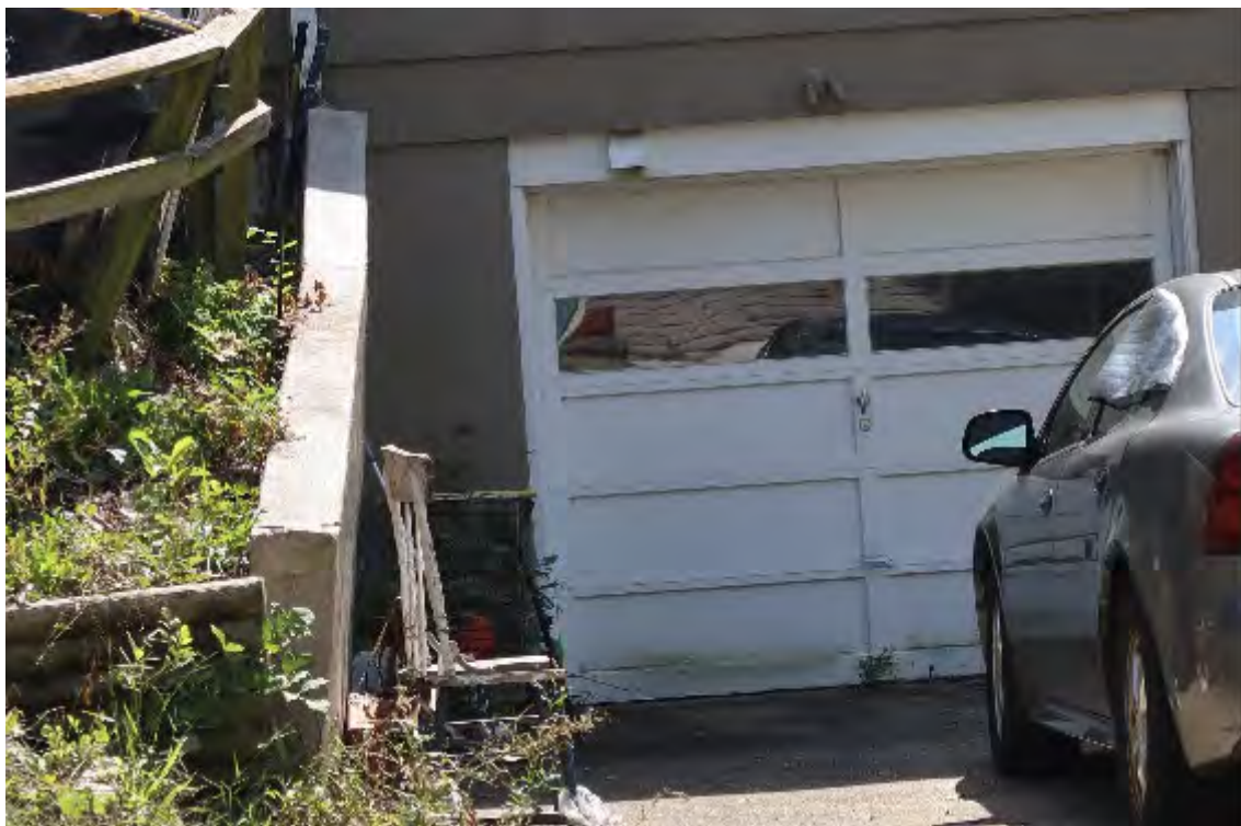
Failing Retaining Wall
