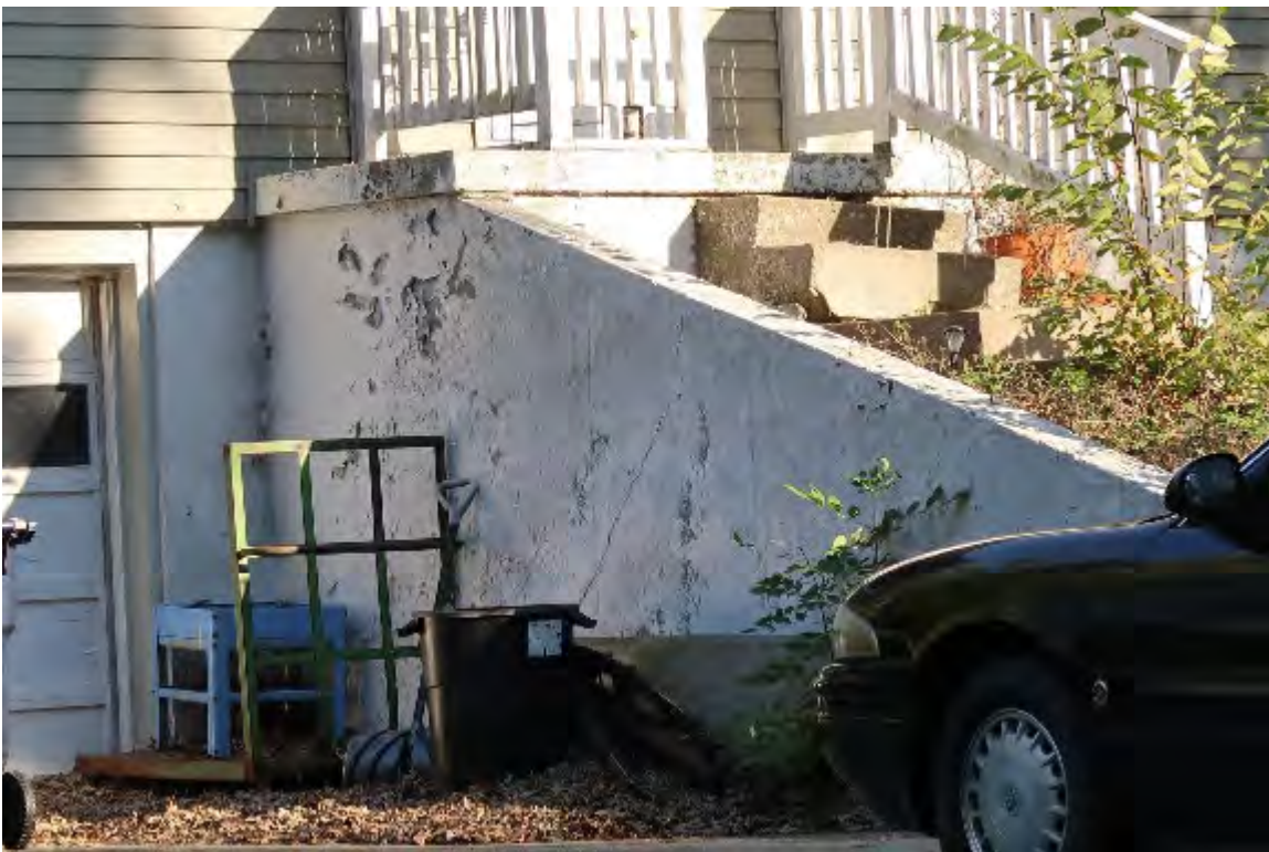
Failing / Unsecured Retaining Wall
