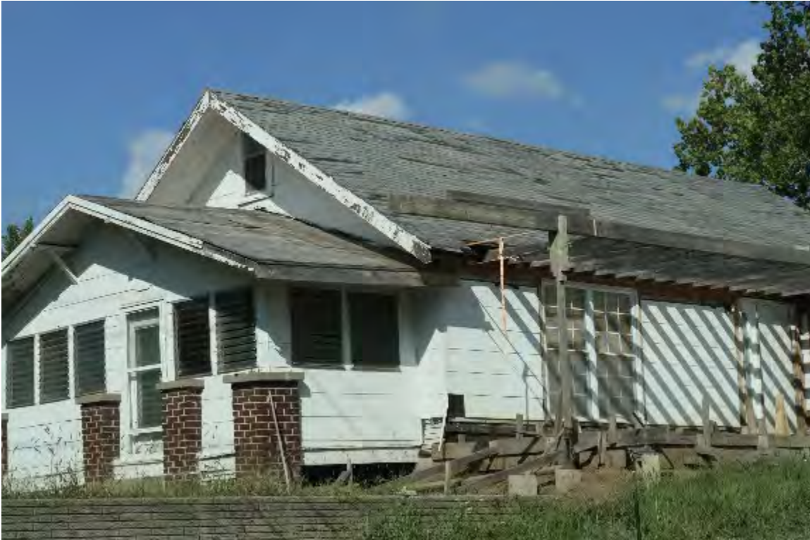
Deterioration (Brookwood Heights)
