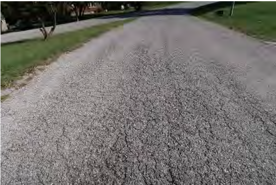
Narrow & Damaged Roadway Lacking Curbs, Gutters, & Pedestrian Sidewalks (Fox Woods)
