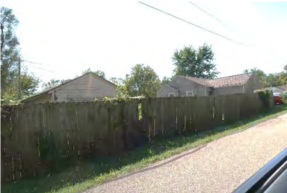
Deteriorating Fencing (Golden Oaks)
