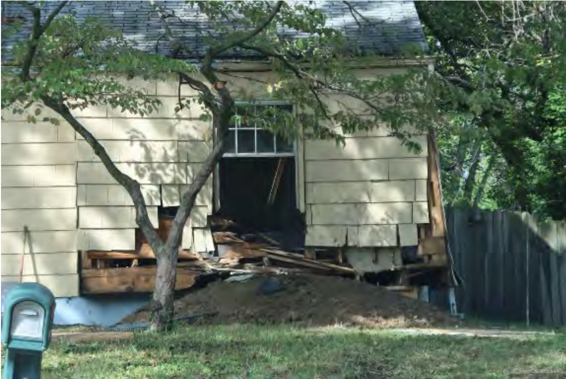
Dilapidation (Antioch Acres)
