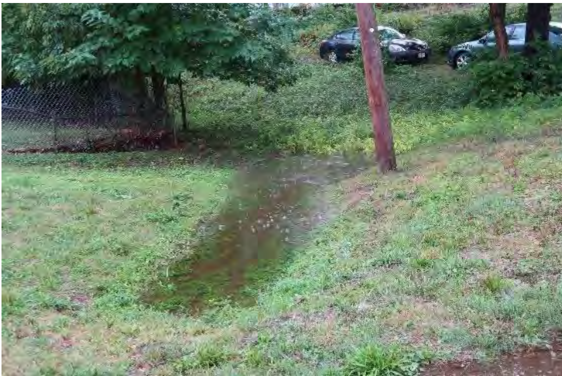
Standing Water In Drainage Ditches (Fox Woods)
