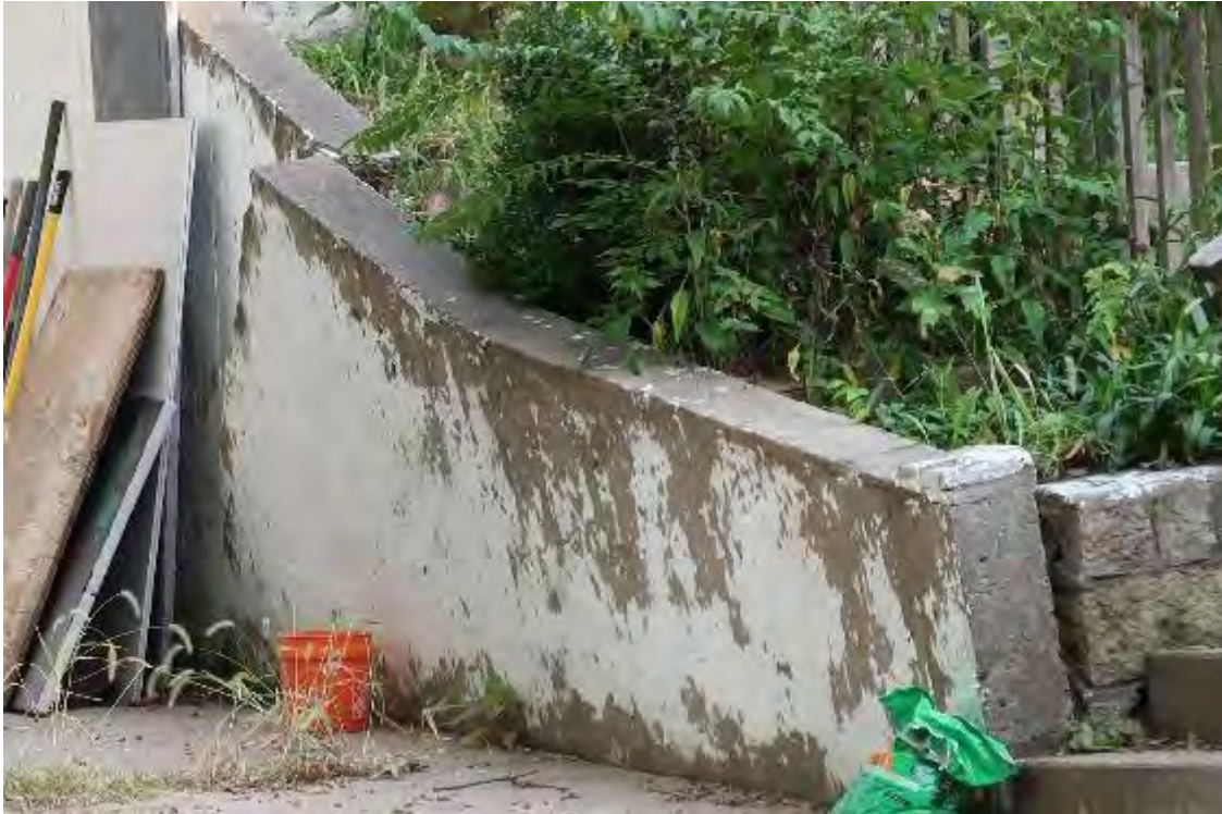
Failing / Unsecured Retaining Wall
