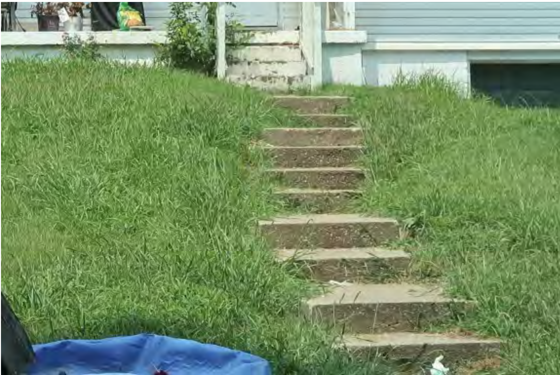
Deteriorating Steps / Porch / Retaining Wall (Edgewood Acres)
