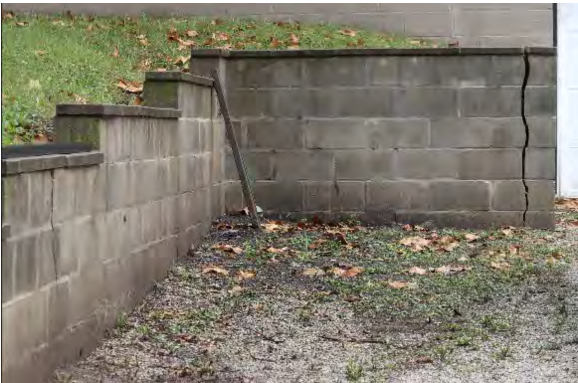
Failing / Unsecured Retaining Wall
