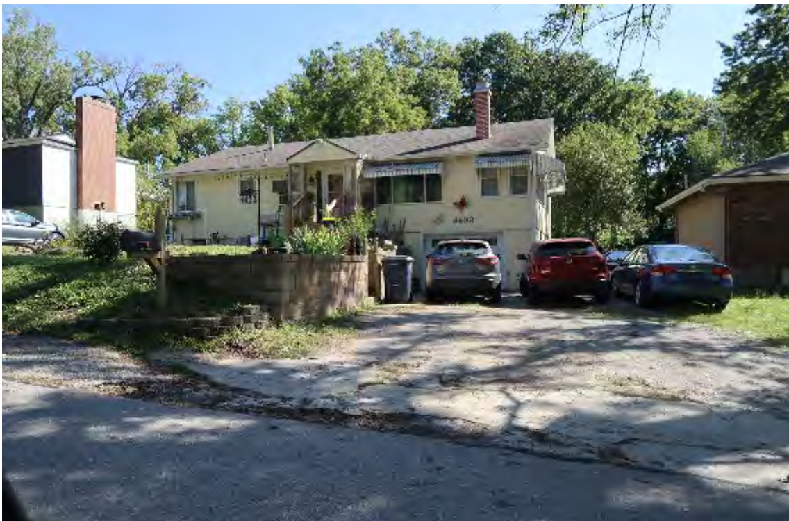
Unsecured Retaining Wall
