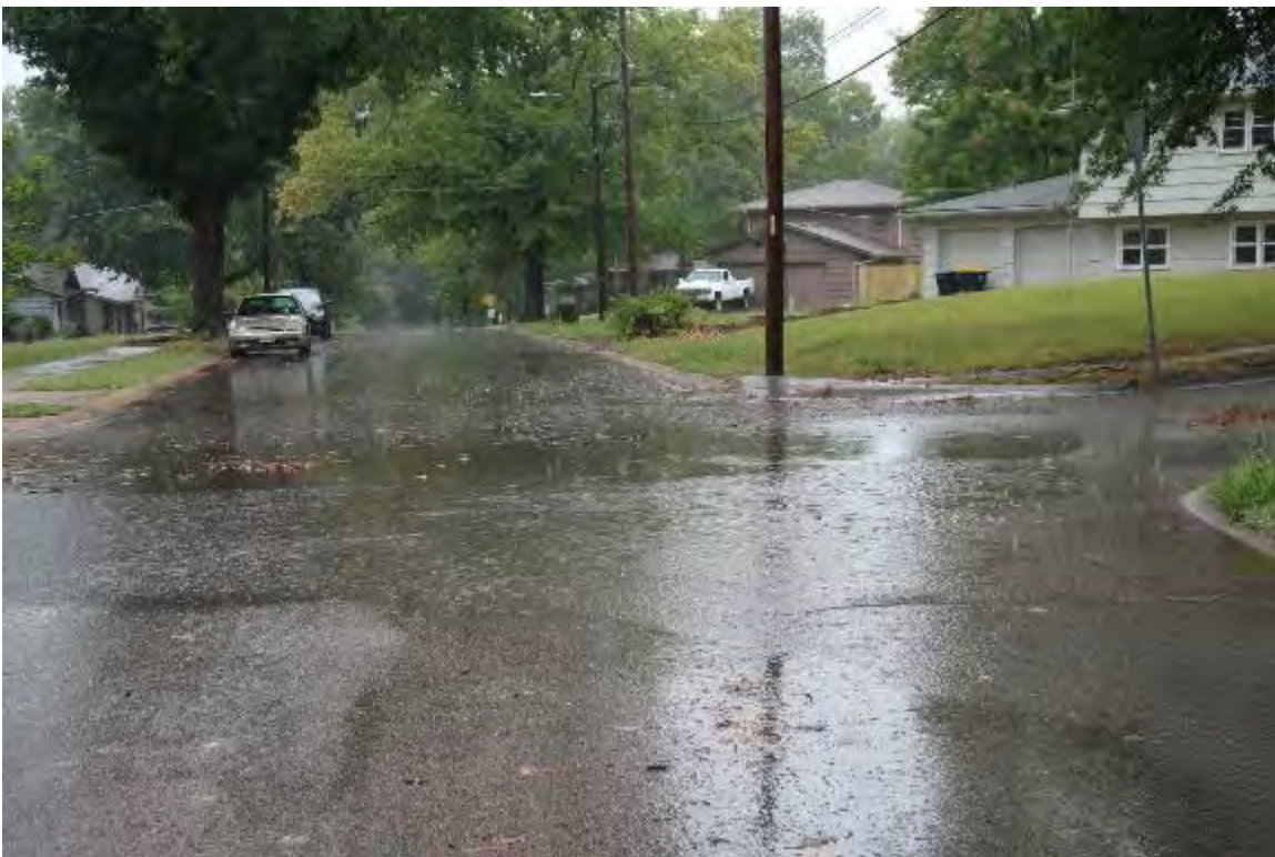
Standing Water In Roadway During Rain Event
