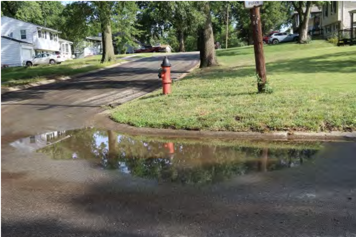
Poor Drainage – Glenhaven Subdivision
