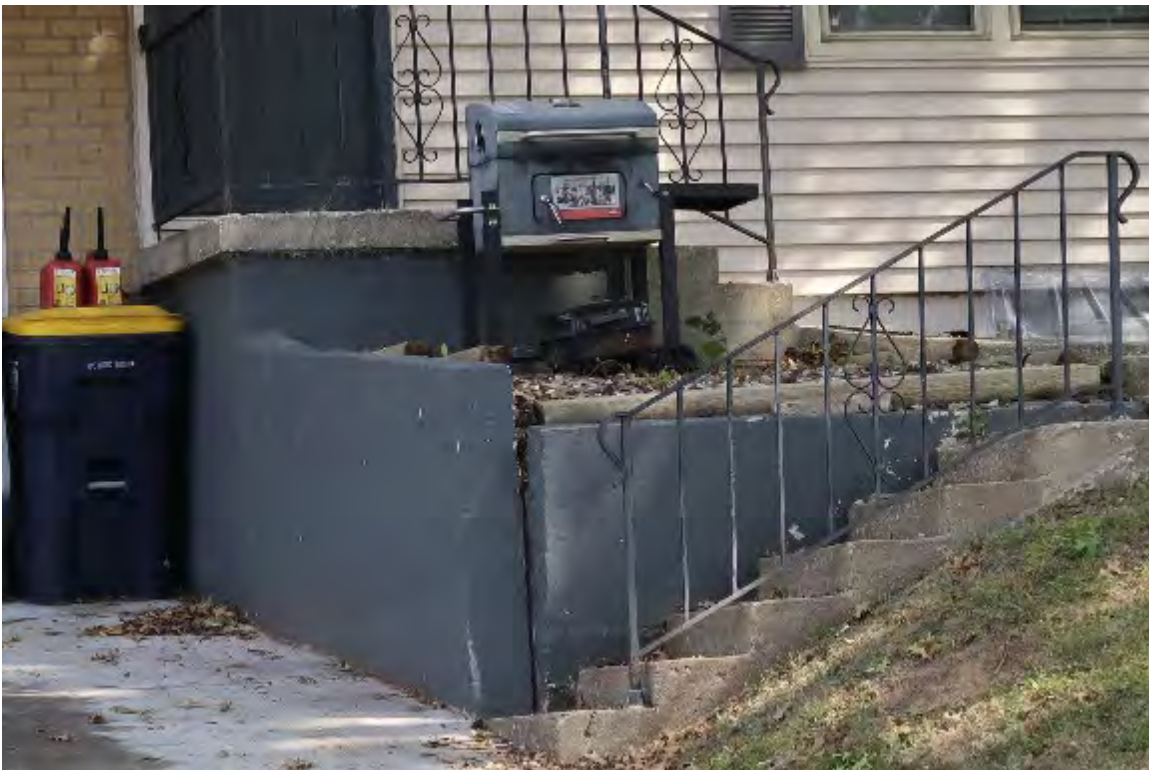
Deteriorating Retaining Wall & Steps (Edgewood Acres)
