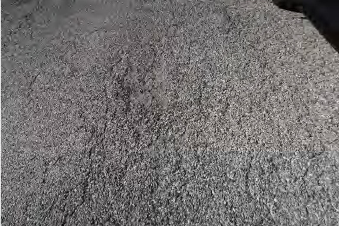
Damaged Roadway (Fox Wood)
