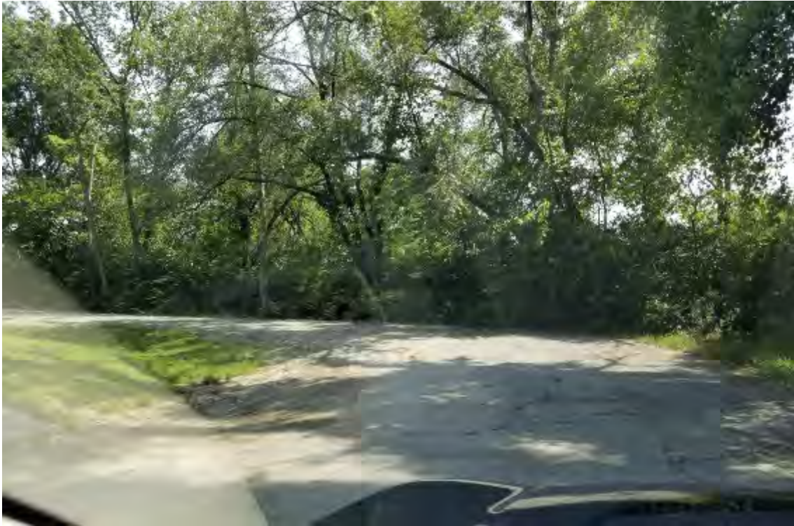
Erosion Adjoining Roadway In Golden Oaks Due To Lack Of Curbs & Gutters
