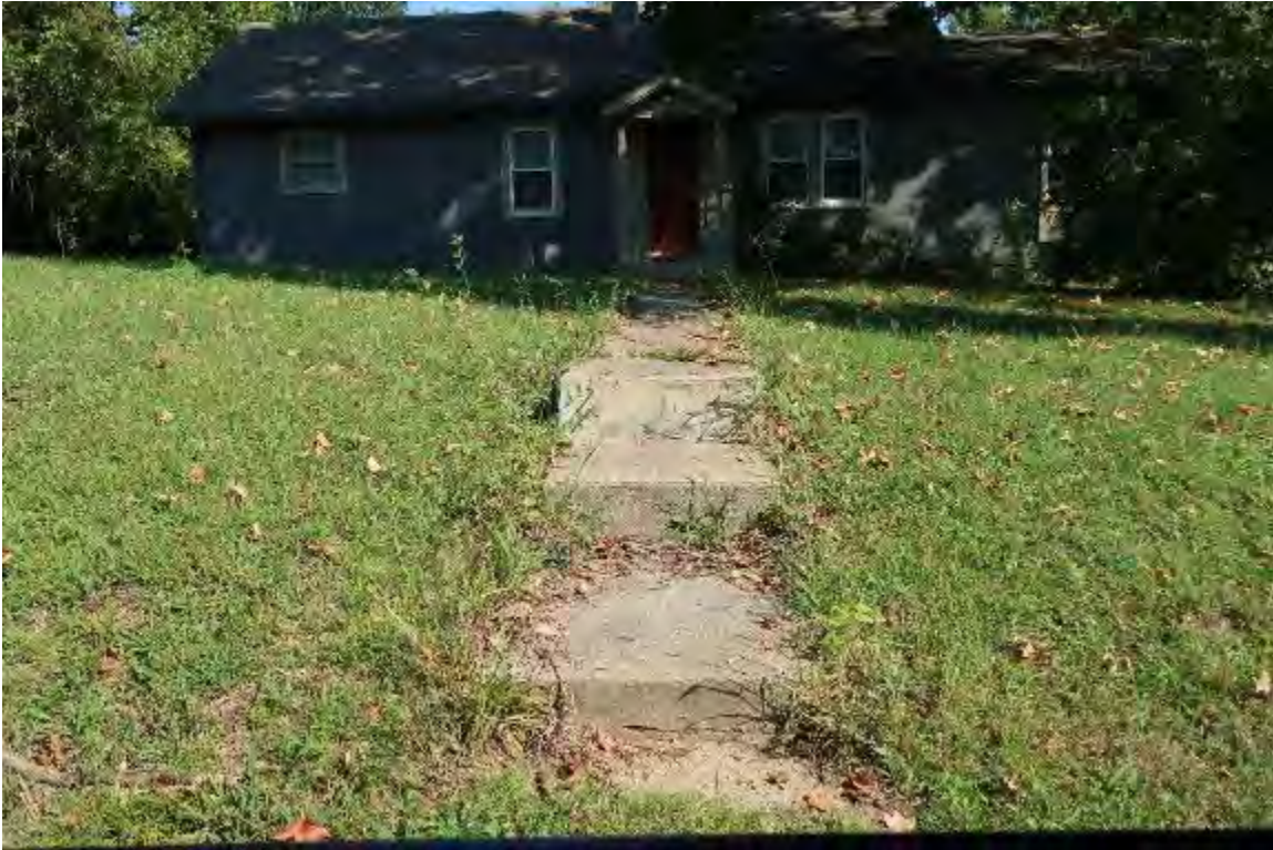
Deteriorating Sidewalk (Golden Oaks)
