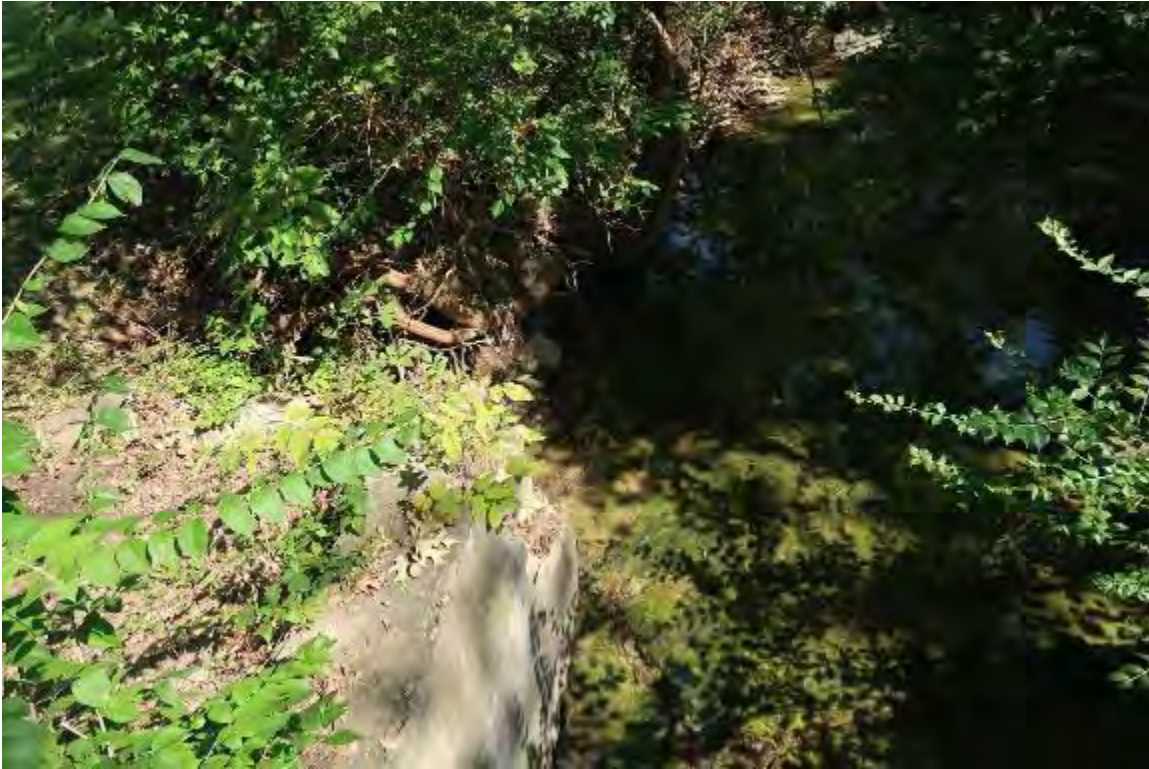
Unsecured Drop Off In Drainage Culvert On NE 45 th Street
