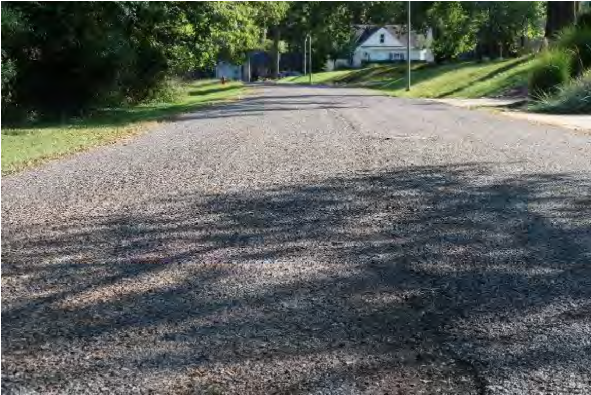
Damaged Roadway (Fox Woods)
