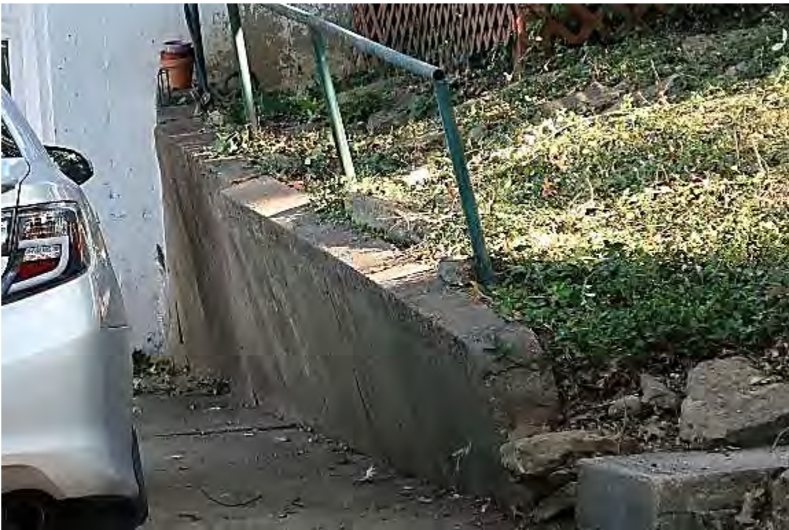
Failing Retaining Wall
