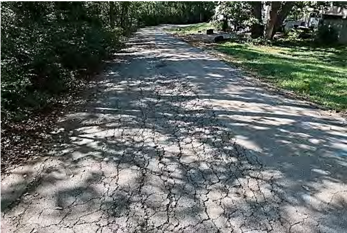
Damaged Roadway (Wood Hills)
