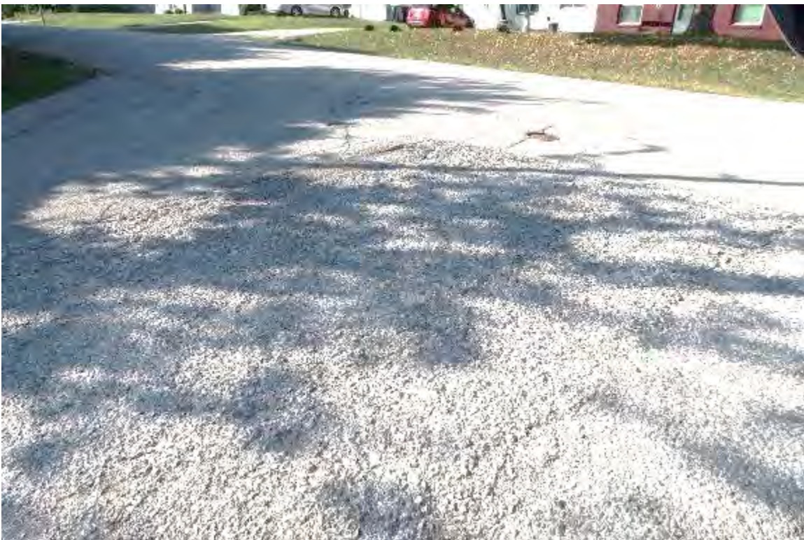
Damaged Roadway (Fox Woods)
