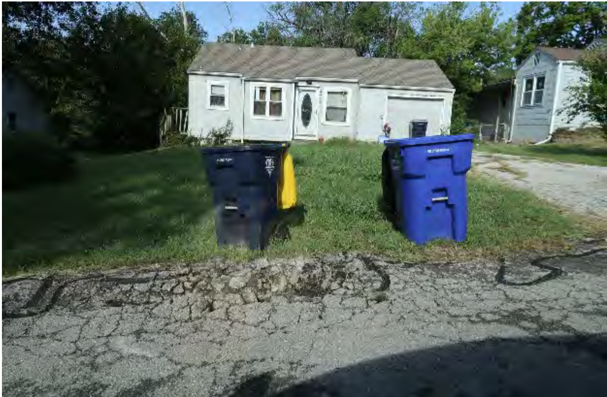
Damaged Roadway (Golden Oaks)
