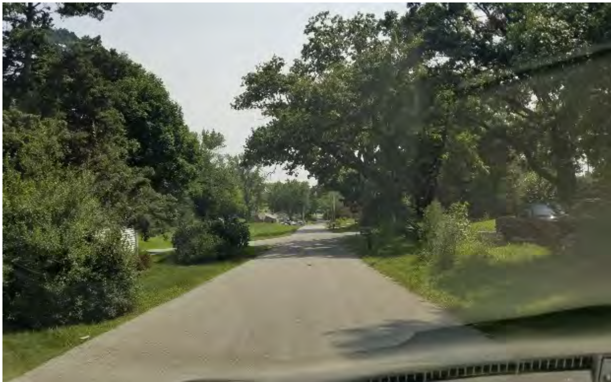
Narrow Roadway Lacking Curbs, Gutters, & Pedestrian Sidewalks (Kelsey Park)
