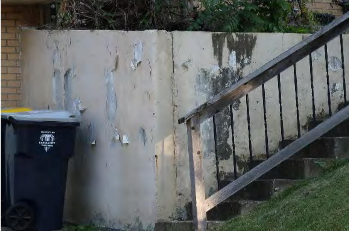
Failing / Unsecured Retaining Wall
