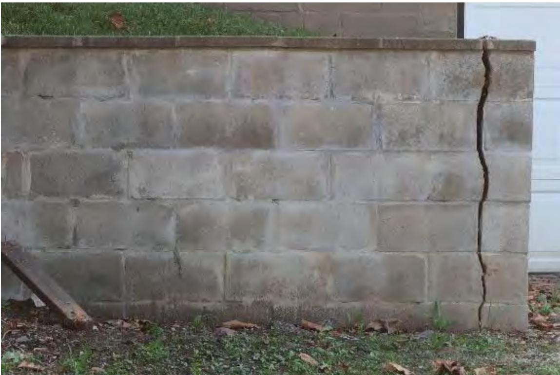
Failing / Unsecured Retaining Wall
