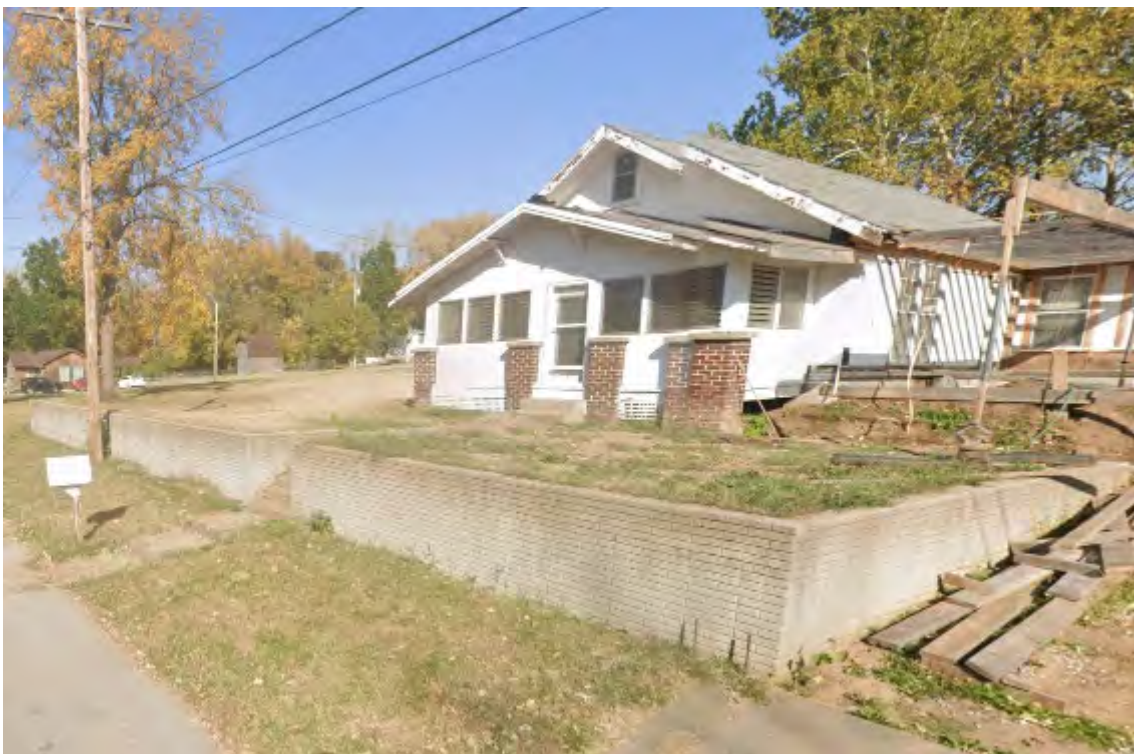
Unsecured Retaining Wall / Lack Of Roof Drainage
