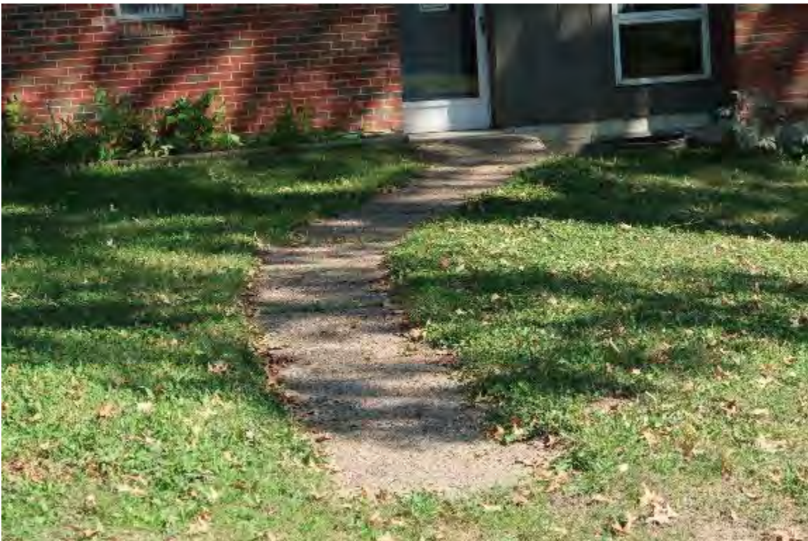
Deteriorating Sidewalk (Wood Hills)
