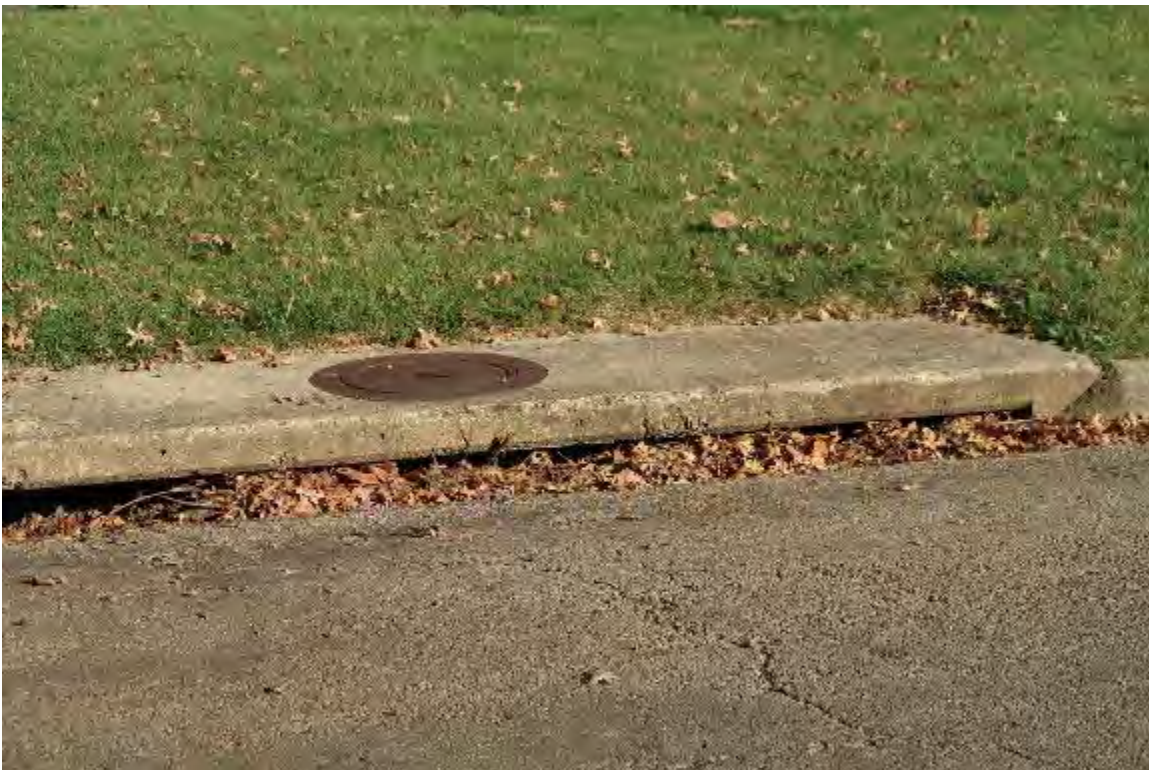
Sewer Inlet Clogged With Debris
