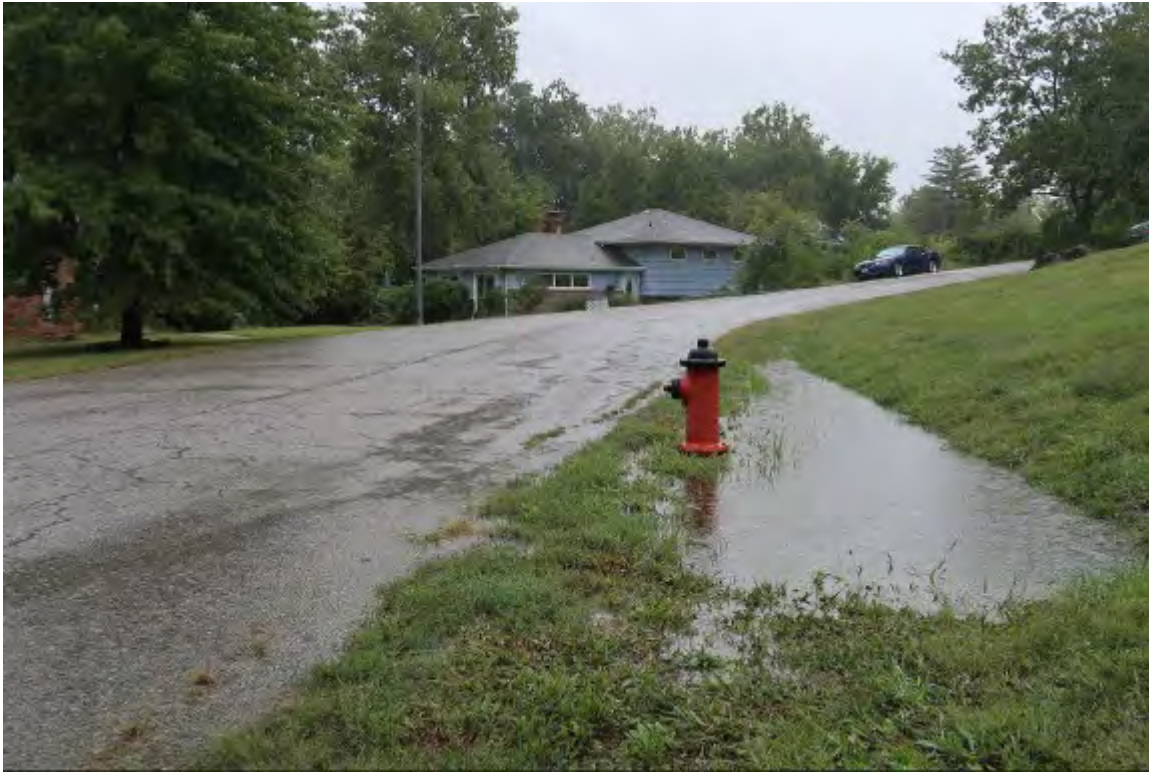
Poor Drainage In Fox Woods Subdivision
