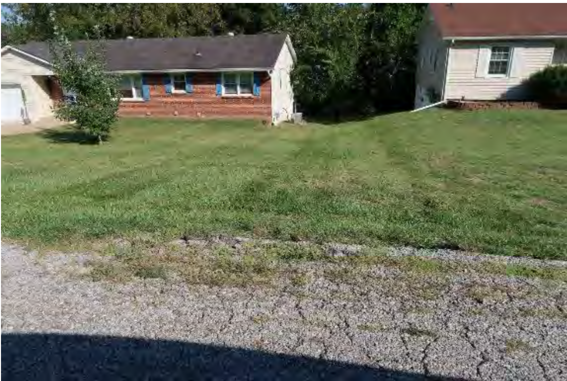
Damaged Roadway (Fox Woods)
