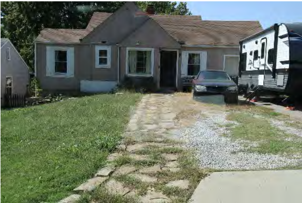
Deteriorating Sidewalk (Golden Oaks)
