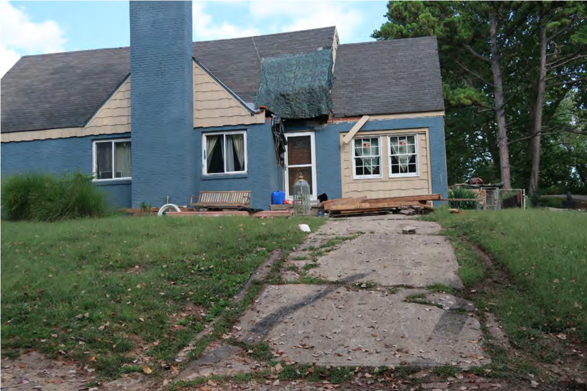
Dilapidation (Wood Hills)
