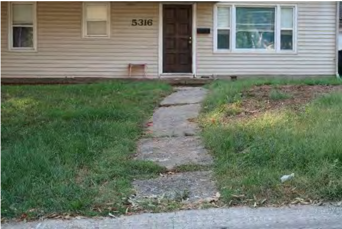
Deteriorating Sidewalk (Edgewood Acres)
