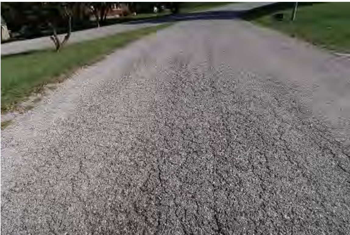
Damaged Roadway (Fox Woods)
