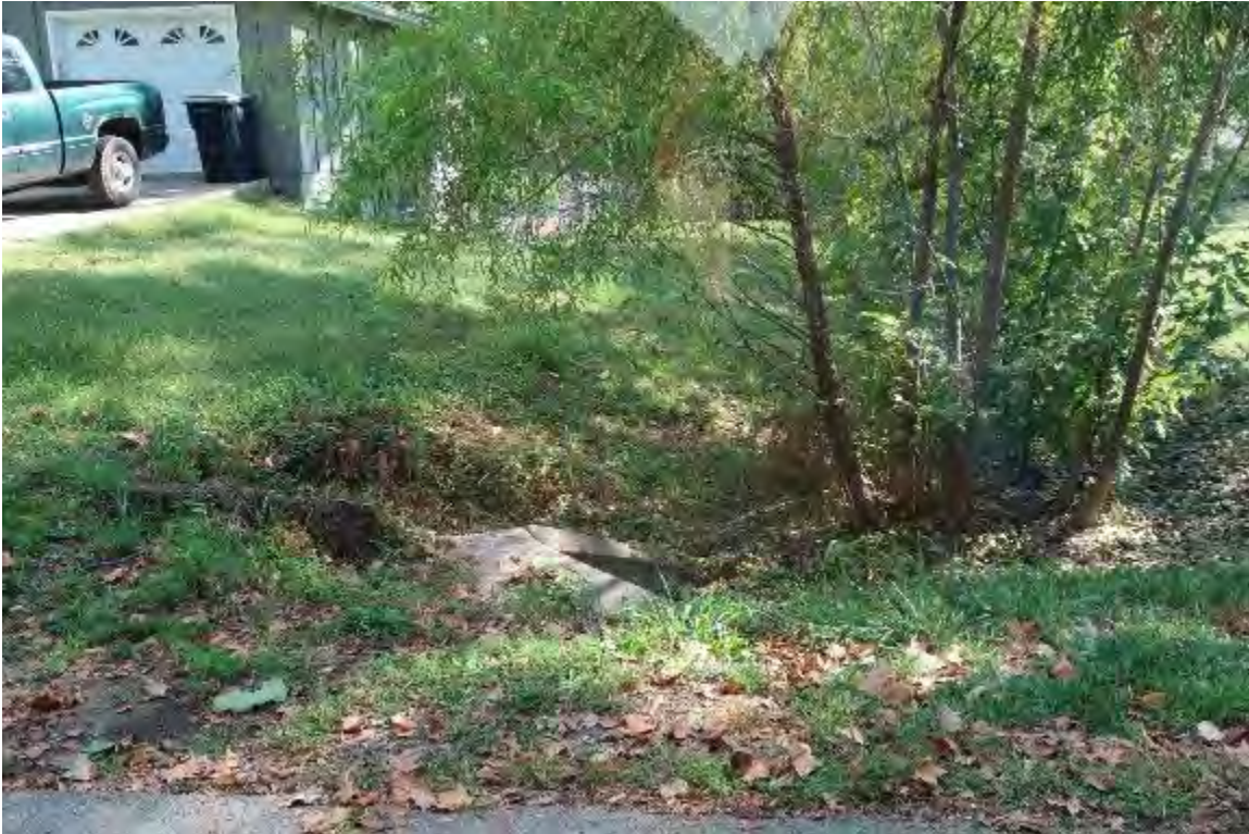
Open Drainage In Brookwood Extension
