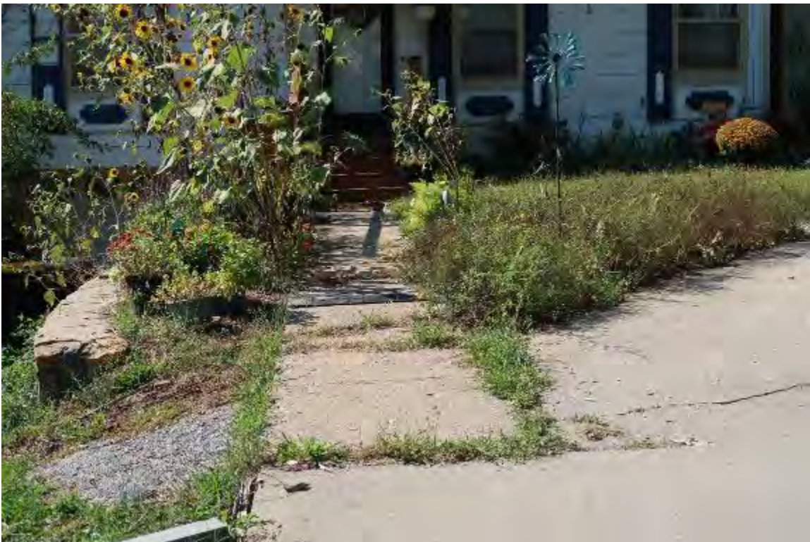
Deteriorating Sidewalk & Unkept Landscaping (Golden Oaks)
