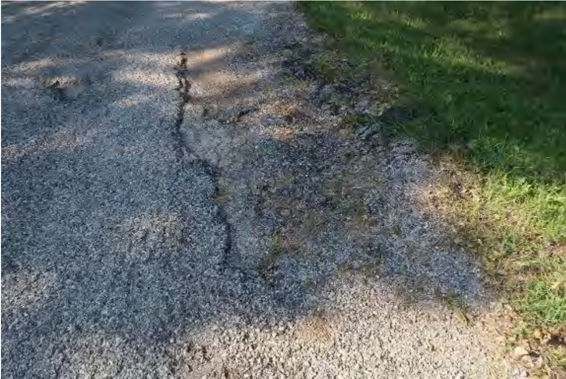
Damaged Roadway (Fox Woods)
