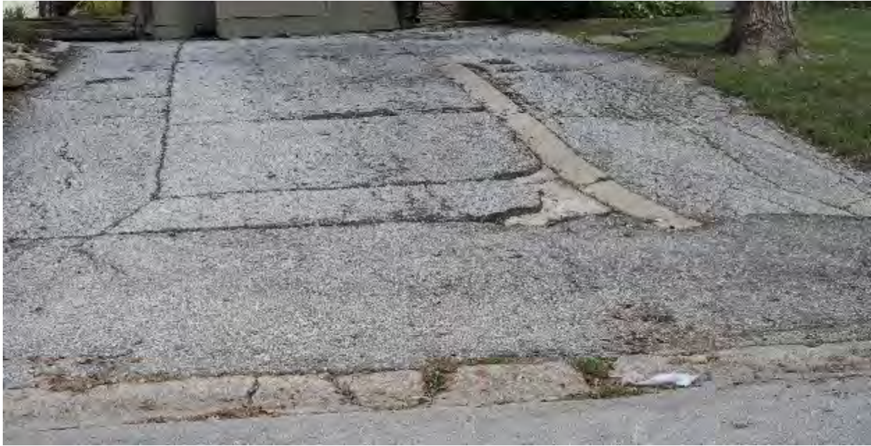
Damaged Gutters (Golden Oaks)
