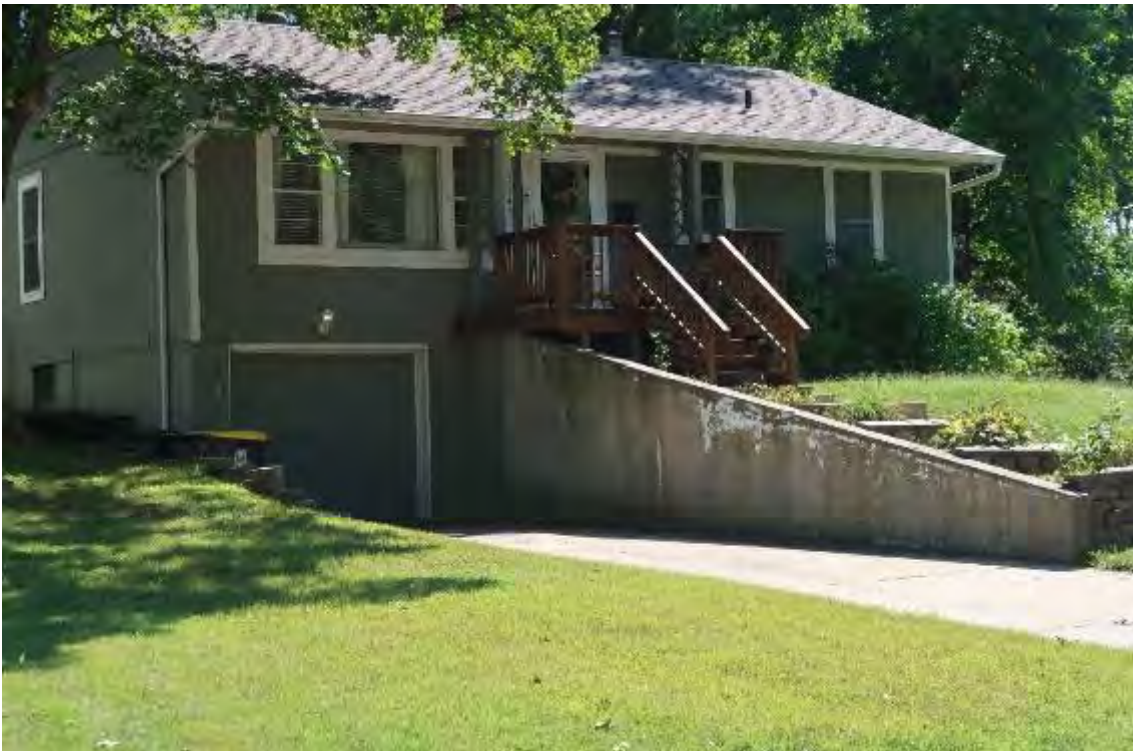
Unsecured Retaining Wall
