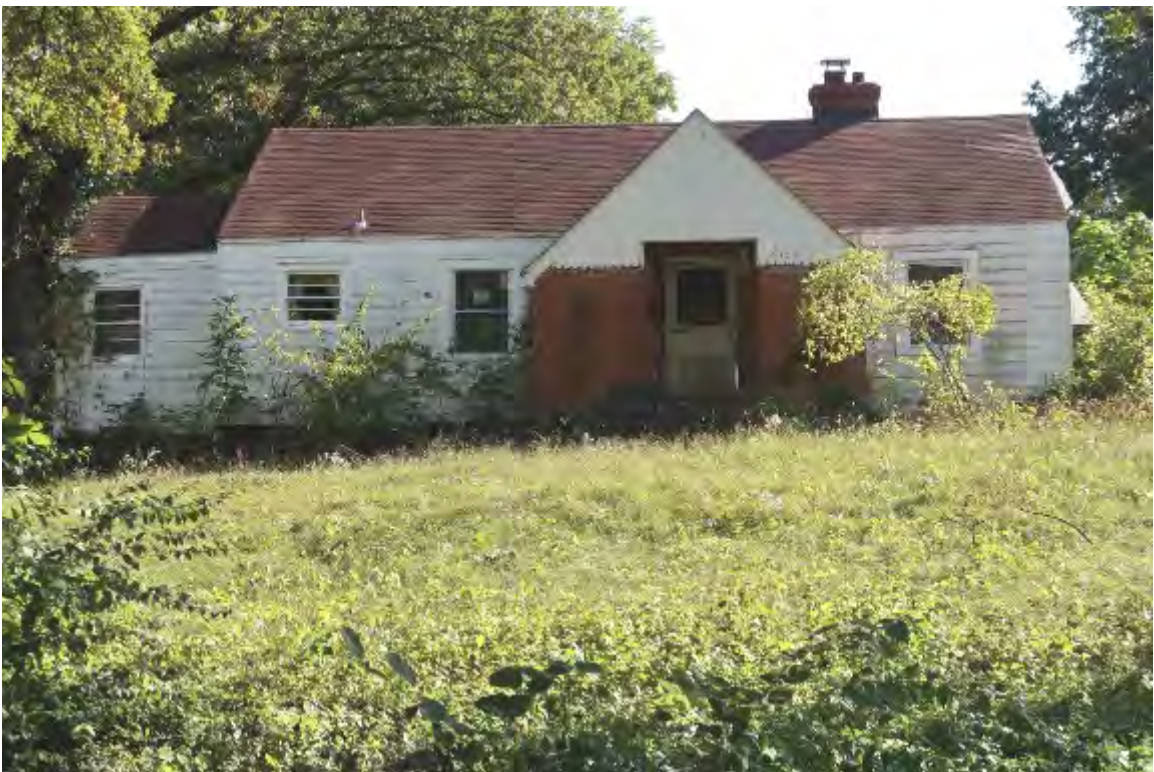
Dilapidation (Fox Woods)
