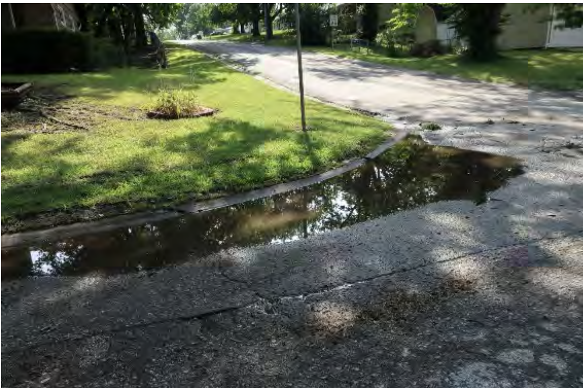
Standing Water Due To Lack Of Sewer Inlet
