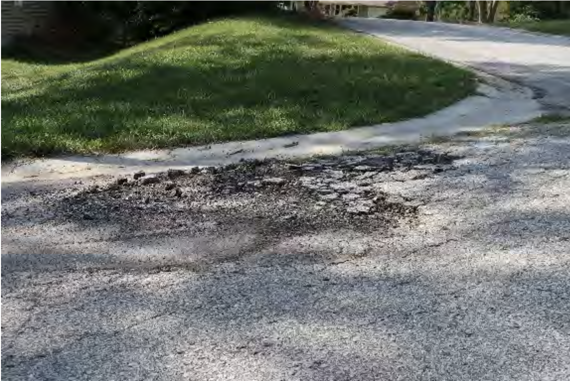
Damaged Roadway (Antioch Gardens)
