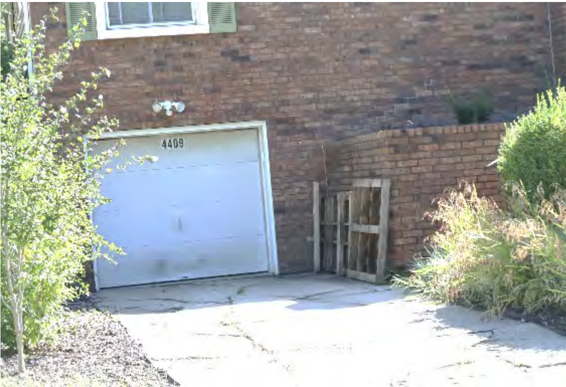
Unsecured Retaining Wall
