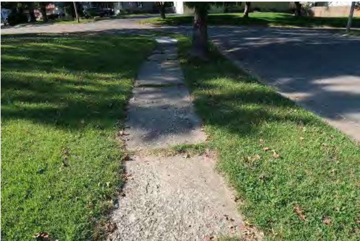
Deteriorating Public Sidewalk (Glenhaven)
