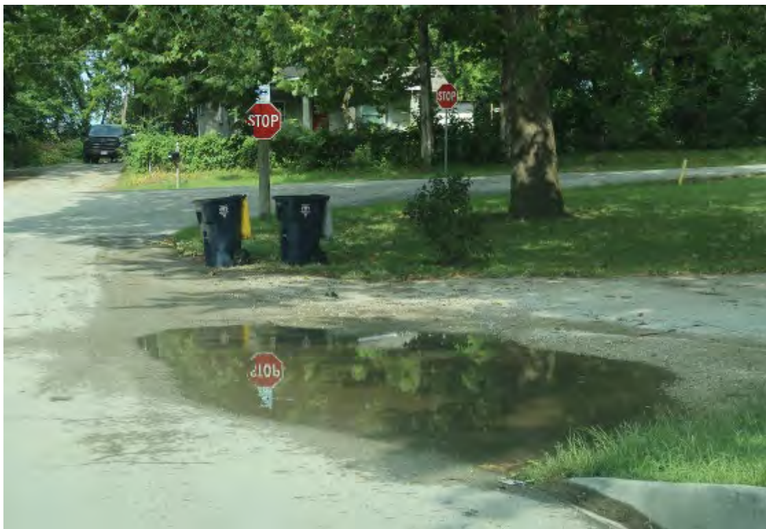
Poor Drainage – Golden Oaks Subdivision
