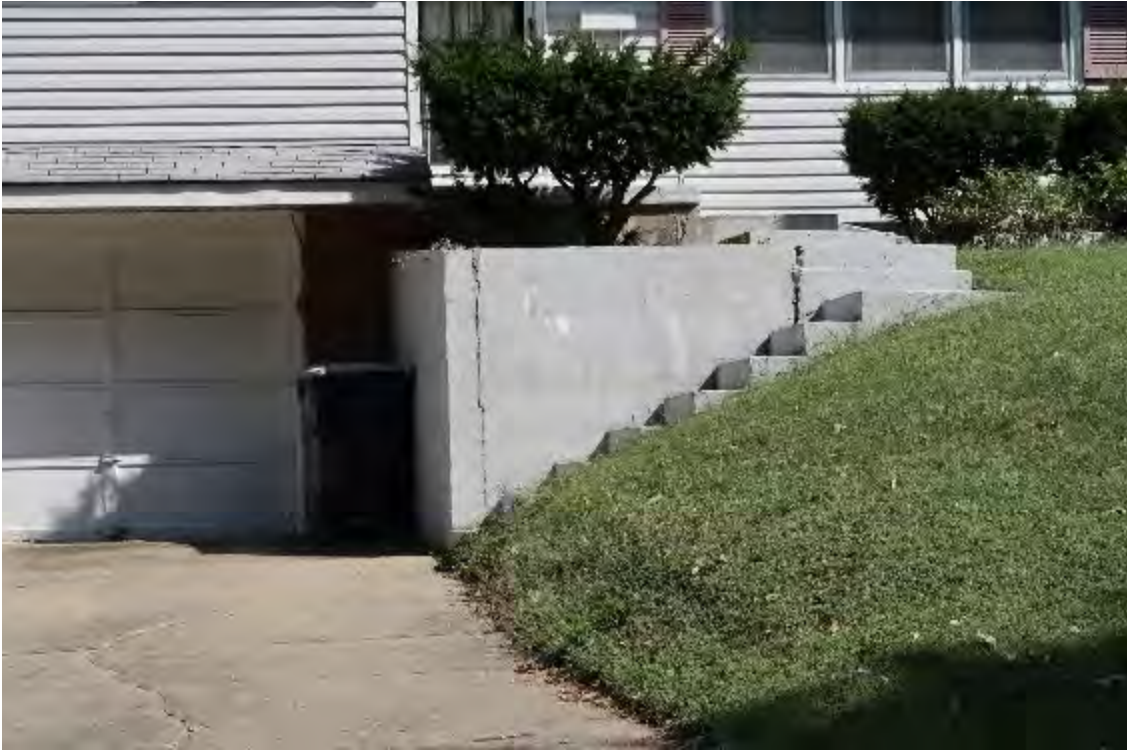
Failing / Unsecured Retaining Wall
