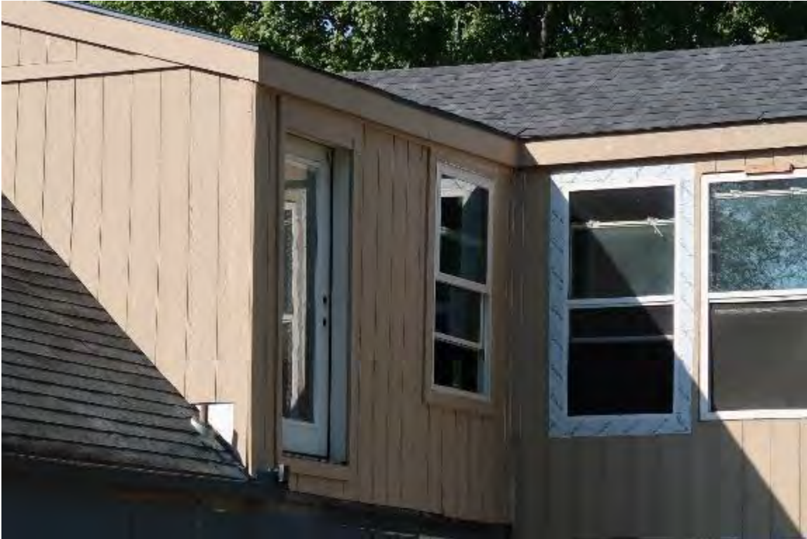
Code Violations (Unsecured Second Level Door; Wood Hills)
