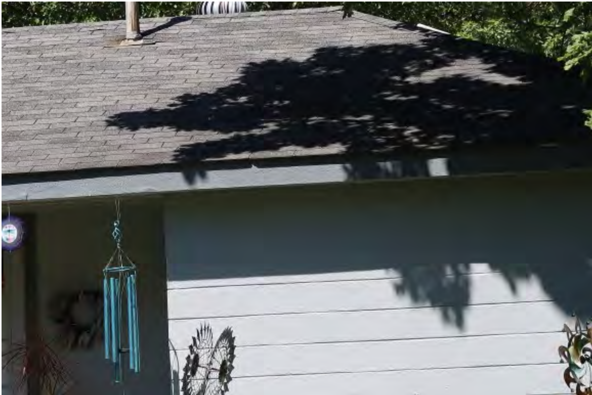
Lack Of Roof Gutters
