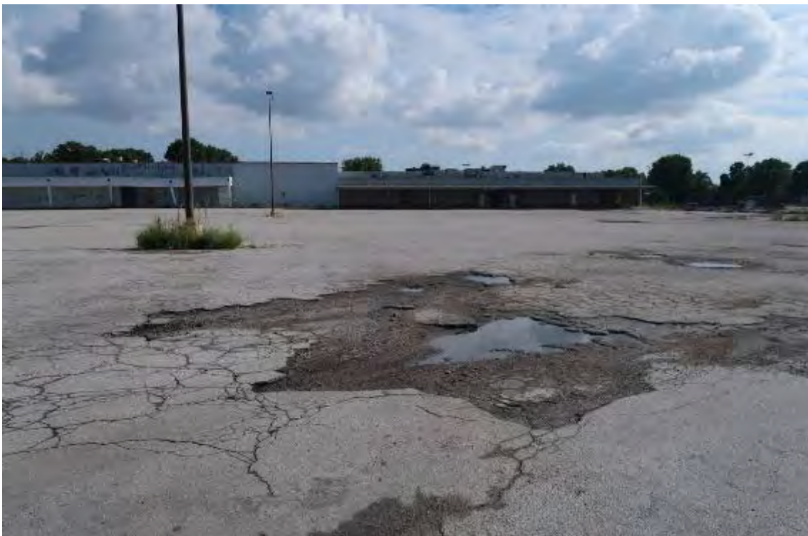
Poor Condition Of Parking Lot (2811 & 2821 N Chouteau Trafficway)
