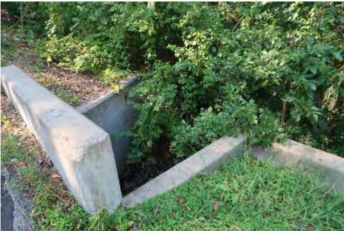
Unsecured Drop Off In Drainage Culvert In Fox Woods
