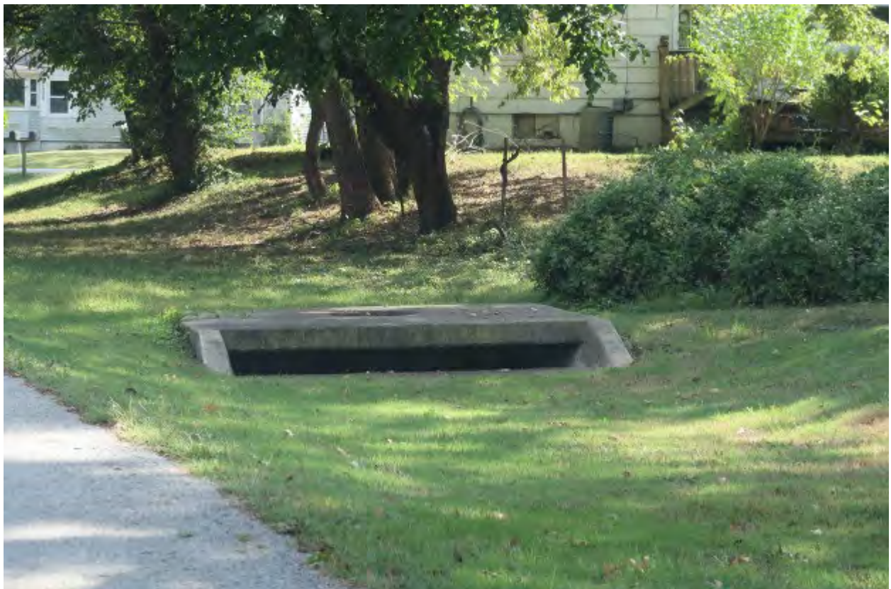
Unsightly Drainage Inlets In Front Yard Lacking Guards – Antioch Acres Subdivision
