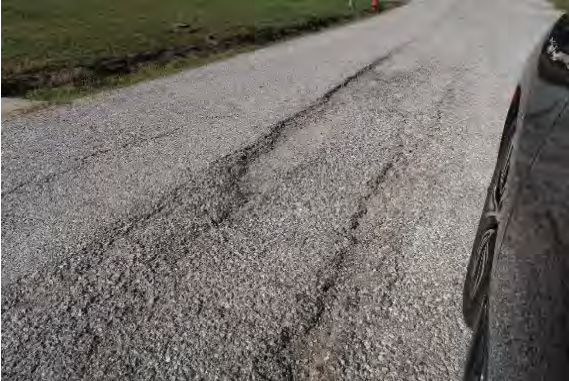
Damaged Roadway (Brookwood Extension)
