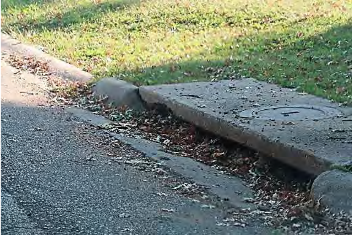
Sewer Inlet Clogged With Debris
