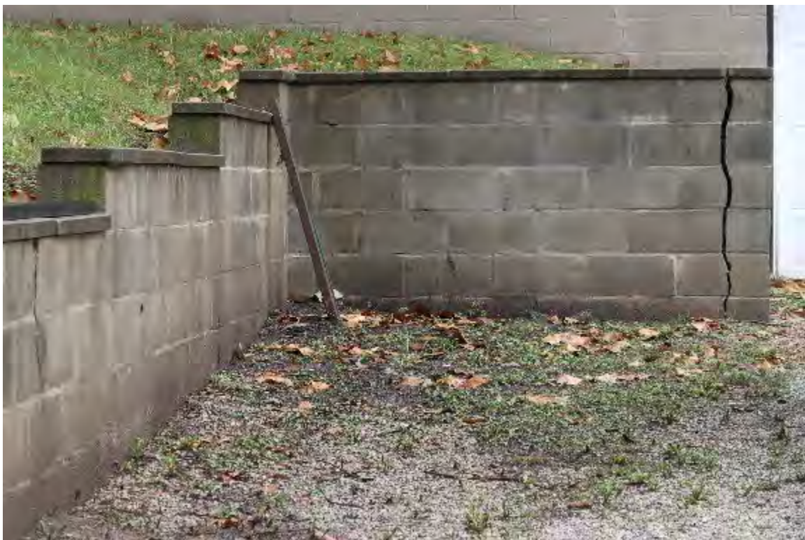
Failing / Deteriorating Retaining Wall (Fox Woods)
