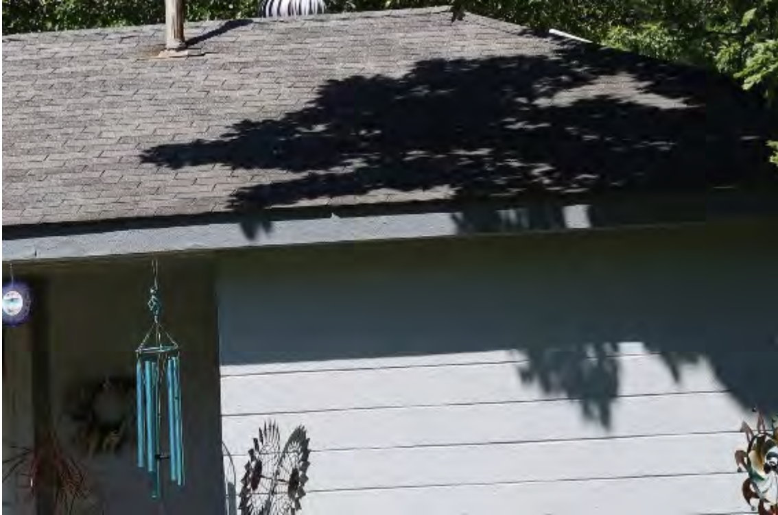
Lack Of Roof Drainage
