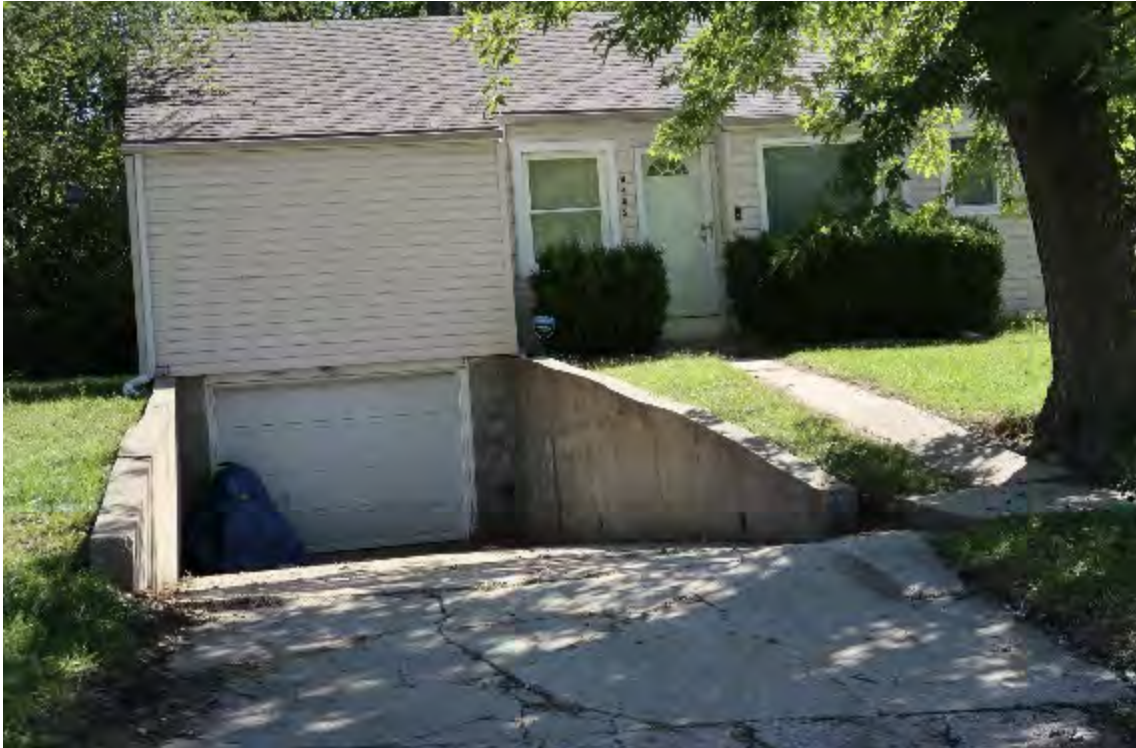
Unsecured Retaining Wall
