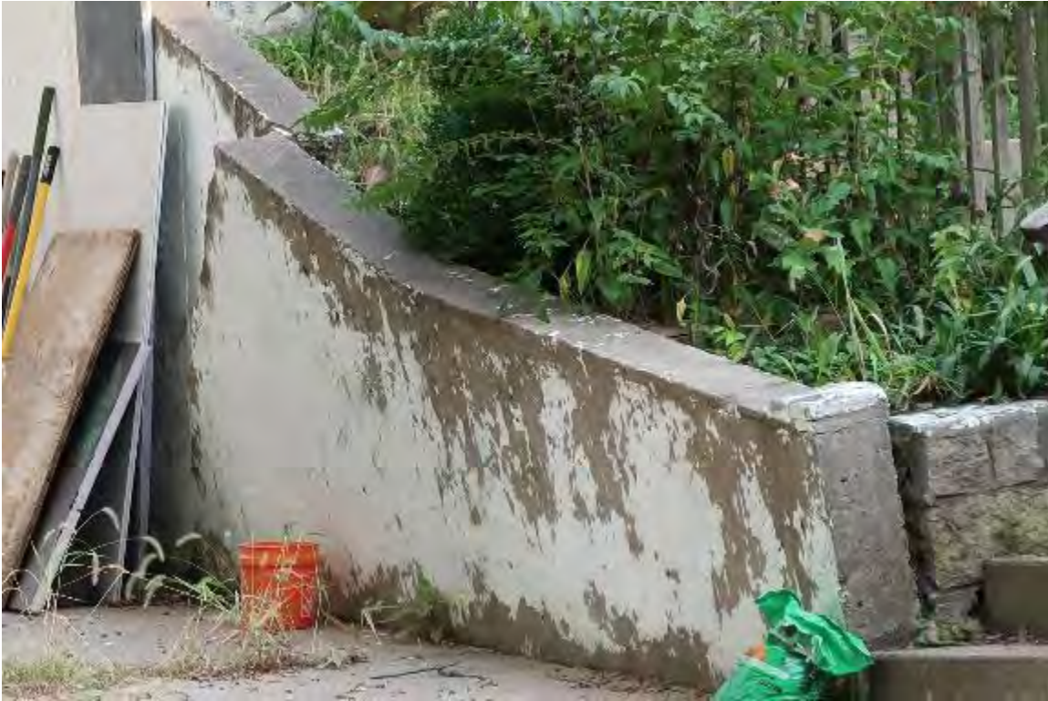
Failing / Unsecured Retaining Wall
