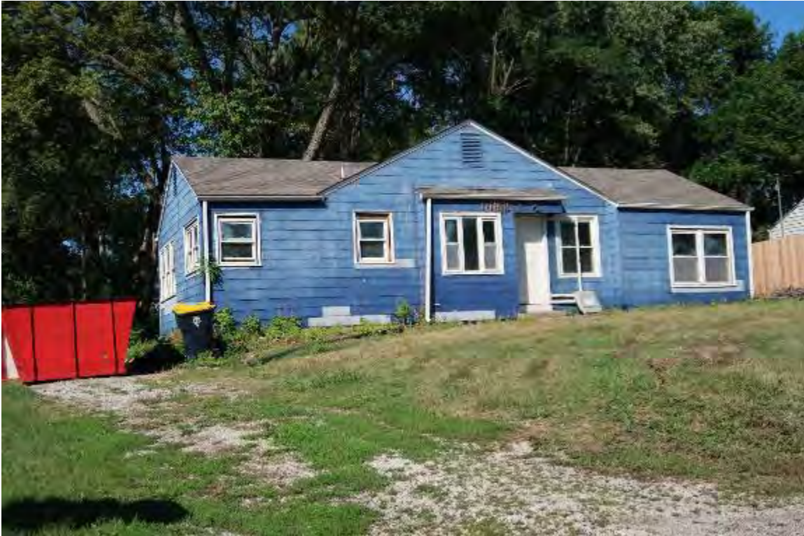
Potential Environmental Issue – Asbestos Shingle Siding
