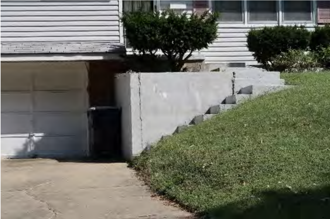
Failing / Unsecured Retaining Wall
