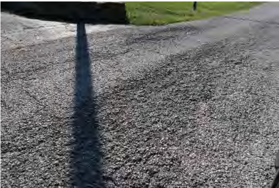
Damaged Roadway (Fox Woods)
