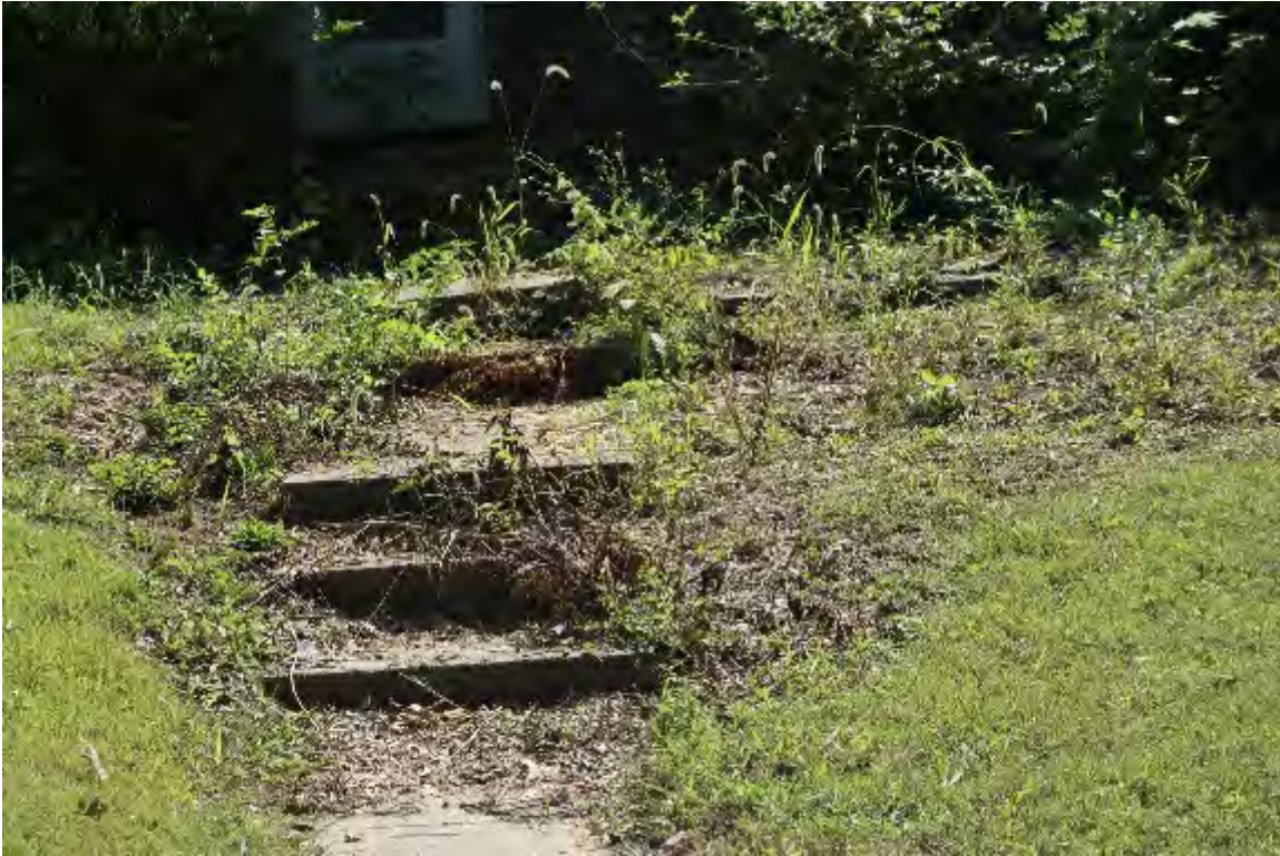
Deteriorating Steps (Fox Woods)
