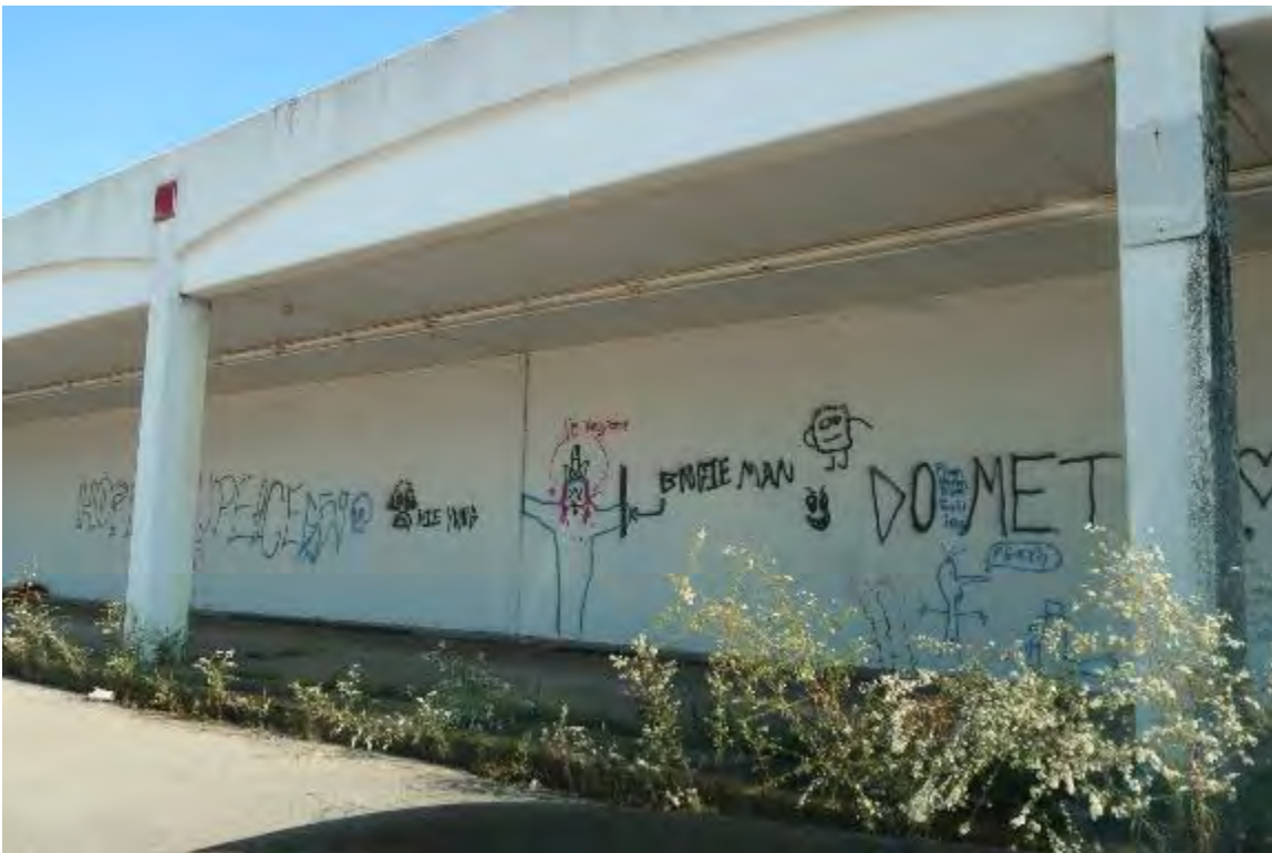
Graffiti On The Kmart Exterior
