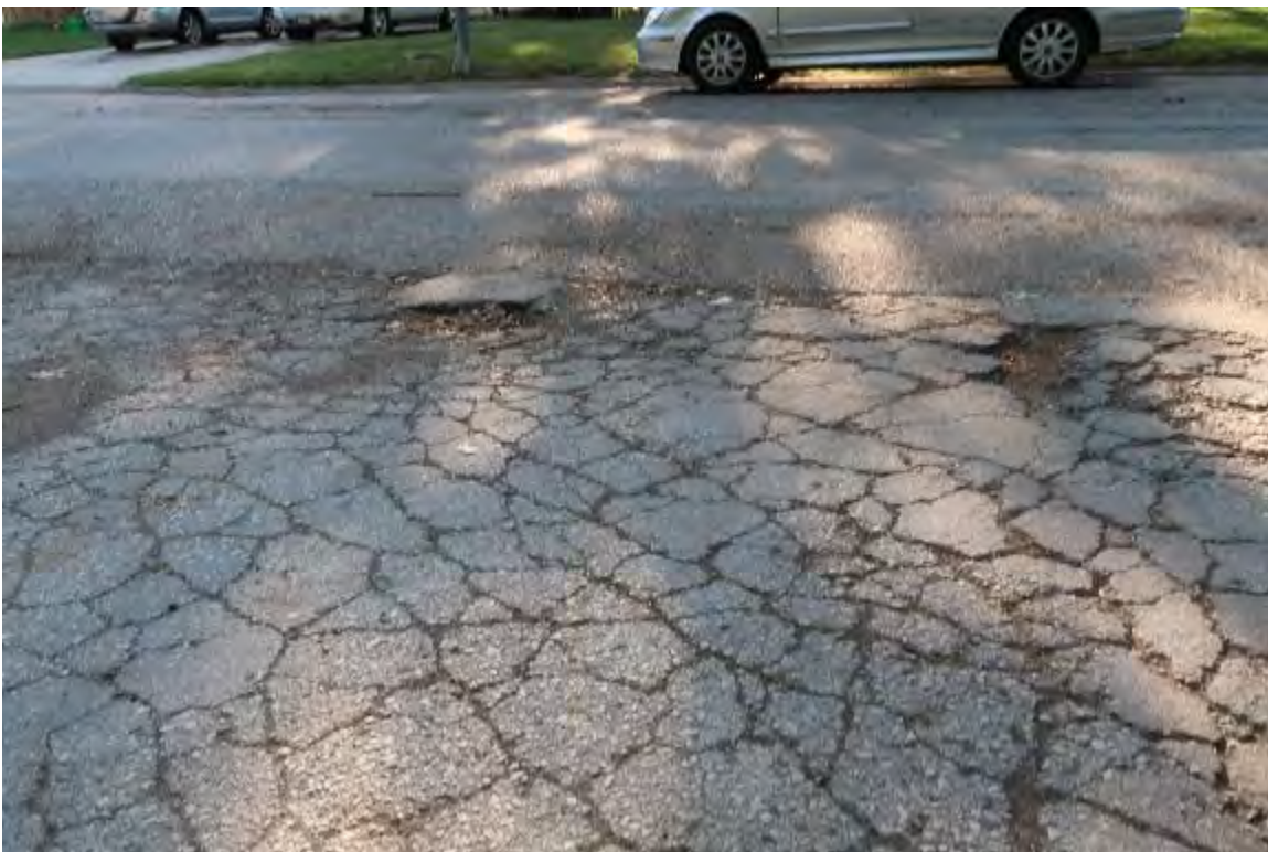
Damaged Roadway (Edgewood Acres)
