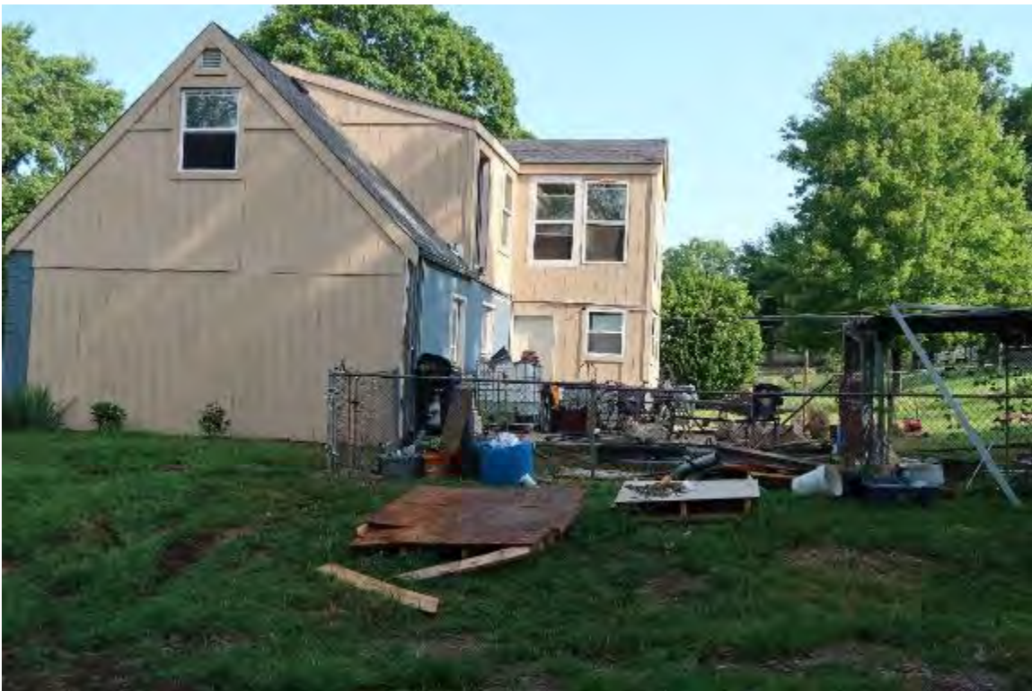
Code Violations (Wood Hills)
