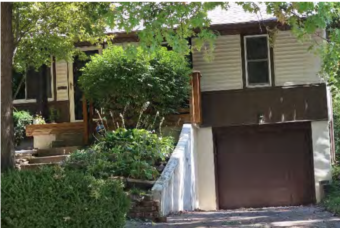
Leaning Retaining Walls & Deteriorated Driveway (Edgewood Acres)
