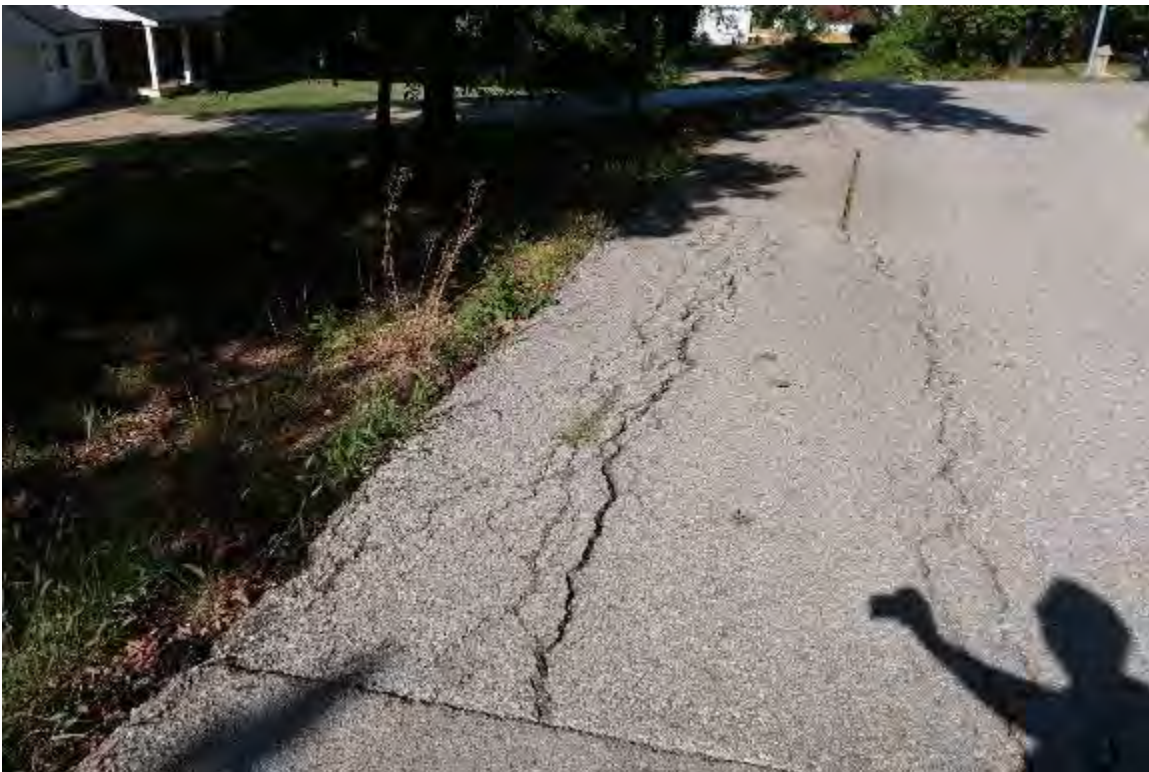
Failing Roadway Due To Erosion From Lack Of Curbs & Gutters (Fox Woods)
