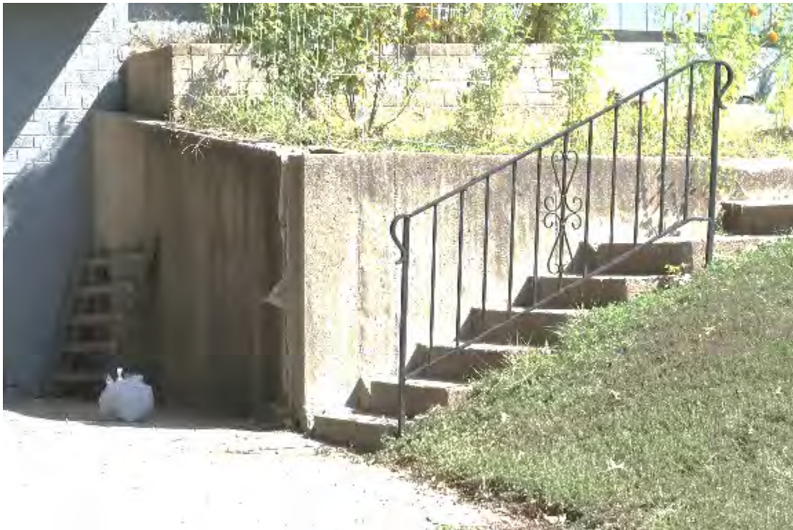
Deteriorating Retaining Wall & Steps (Edgewood Acres)
