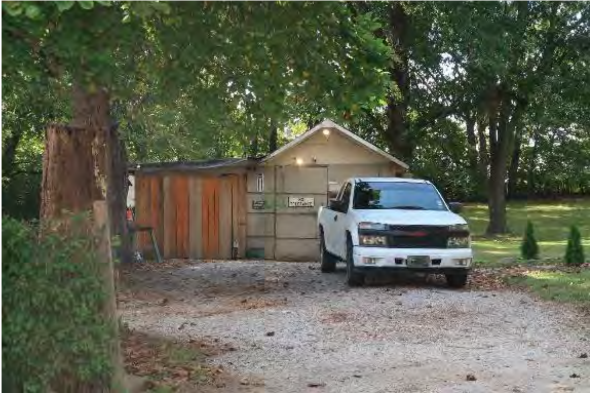
Dilapidation (Brookwood Extension)
