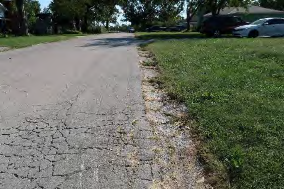
Damaged Roadway & Gutters (Wood Hills)
