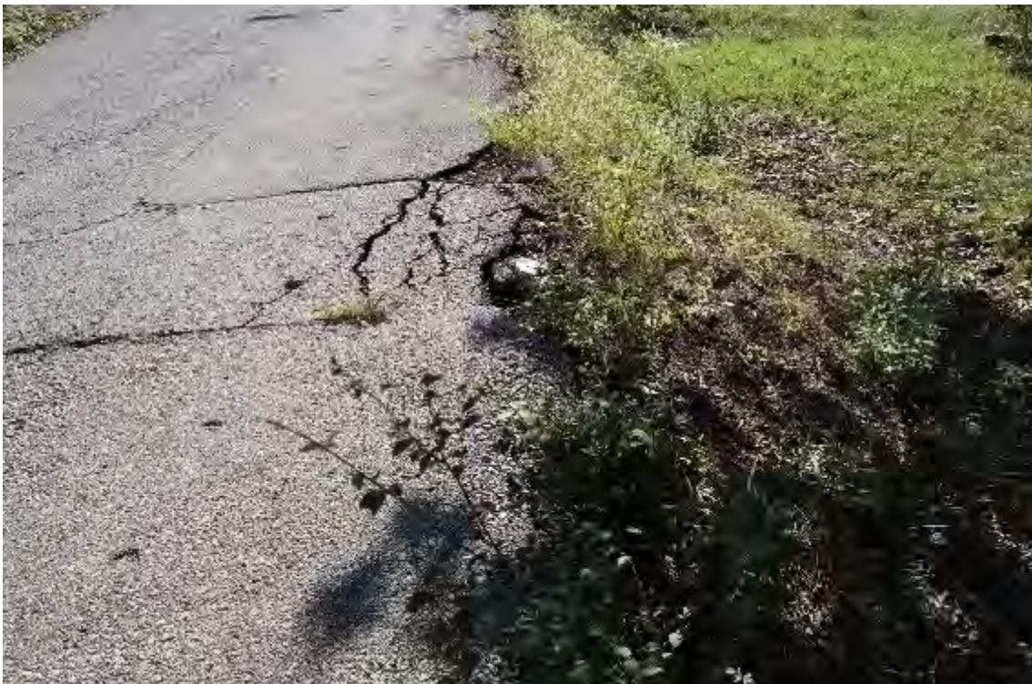
Erosion Adjoining Failing Roadway In Fox Woods Due To Lack Of Curbs & Gutters
