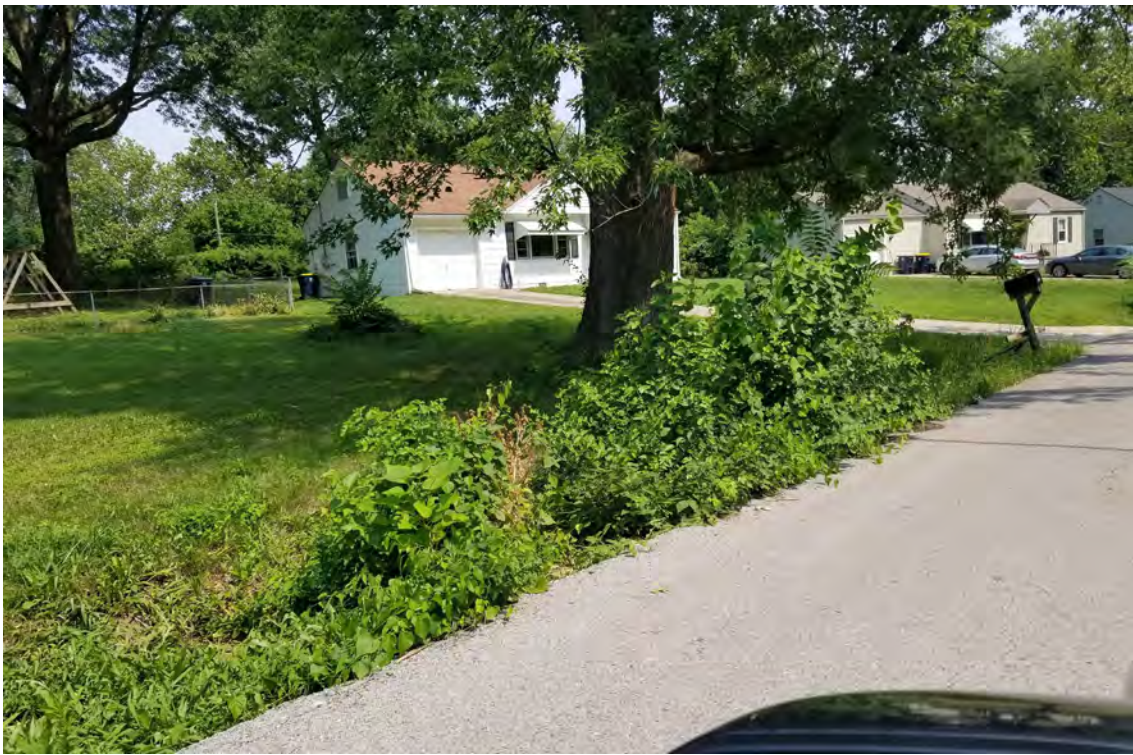
Excessive Weeds In Drainage Ditches (Antioch Acres)
