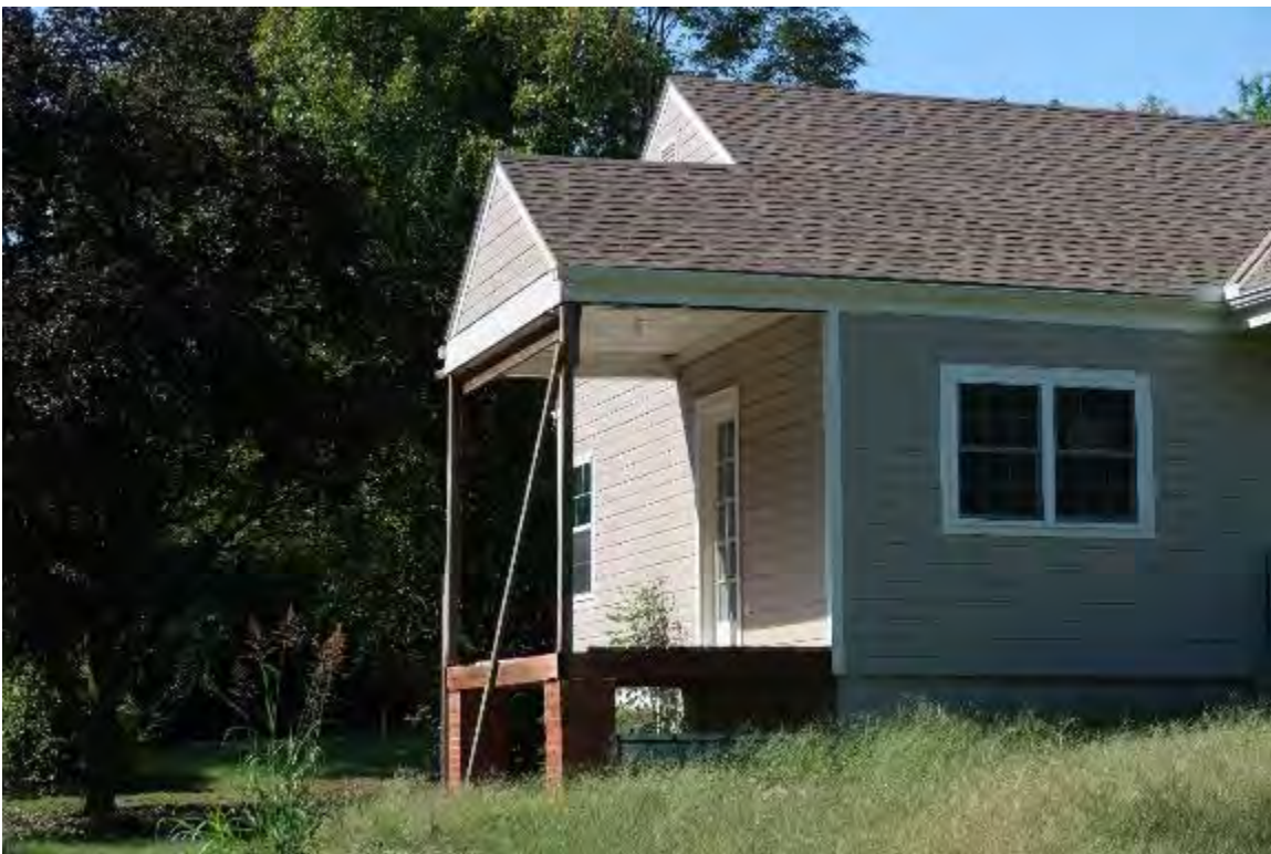
Unsafe Decking (Golden Oaks)
