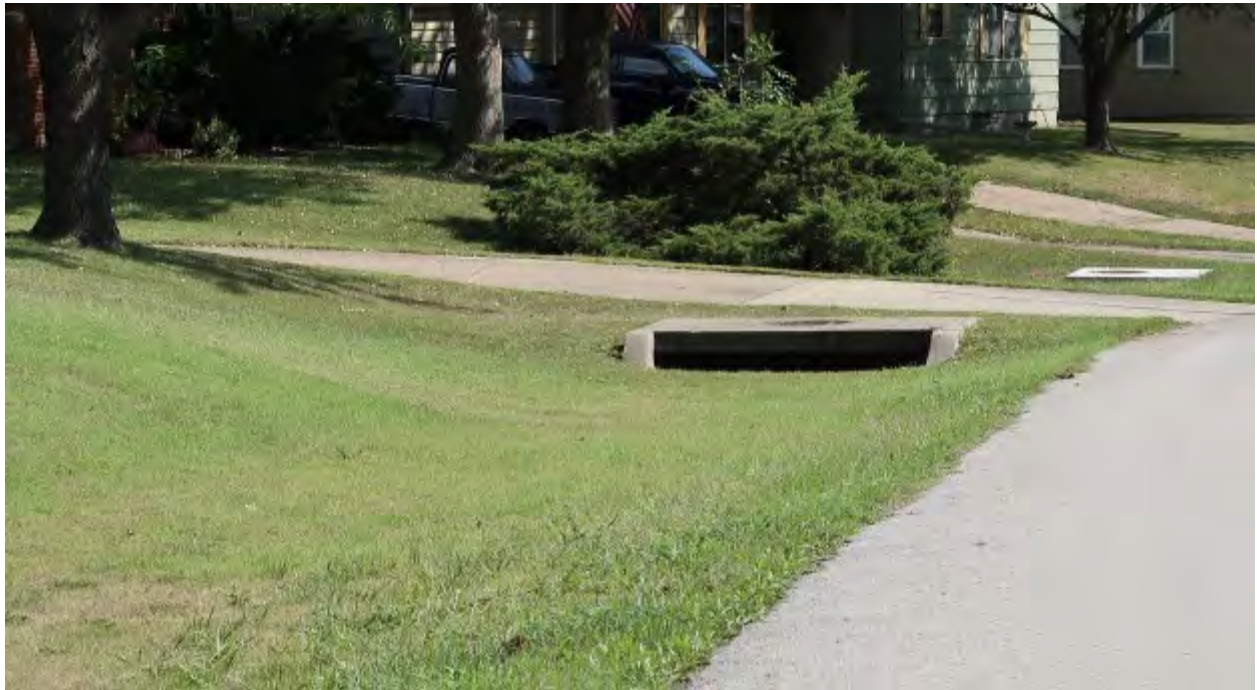
Unsightly Drainage Inlets In Front Yard Lacking Guards – Antioch Acres Subdivision
