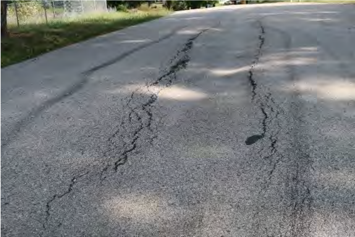
Narrow & Damaged Roadway (Cave In) Lacking Curbs, Gutters, & Pedestrian Sidewalks (Antioch Acres)
