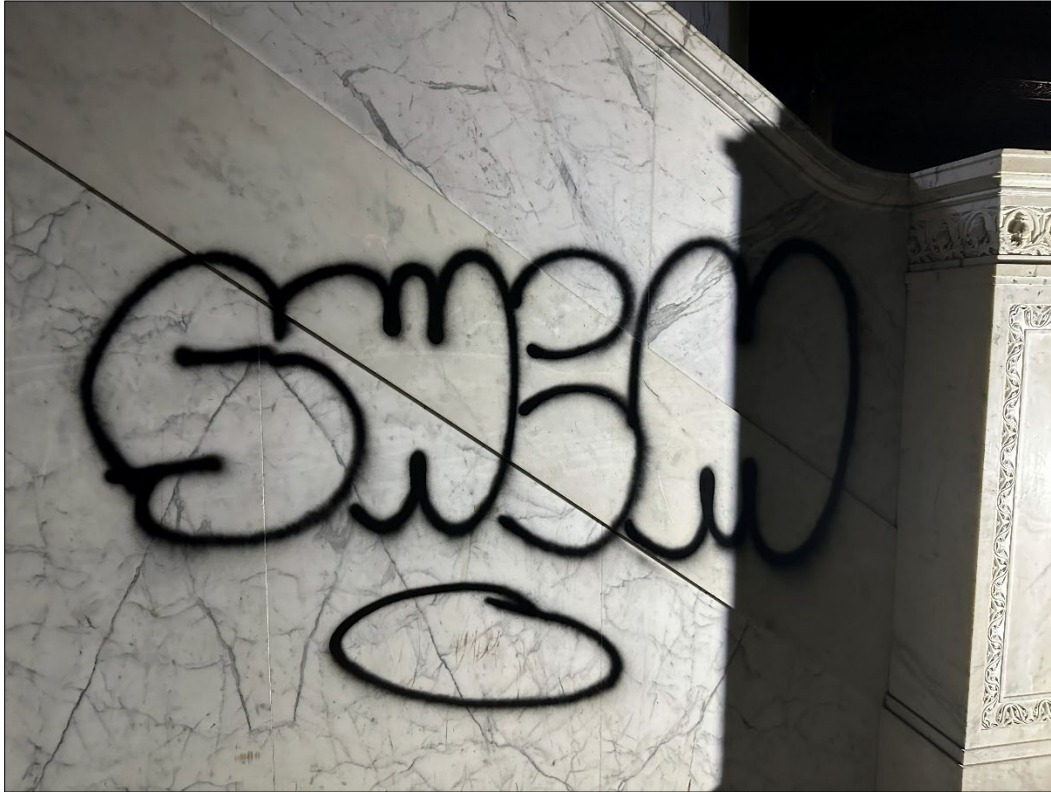
818 Grand Blvd – interior – graffiti
