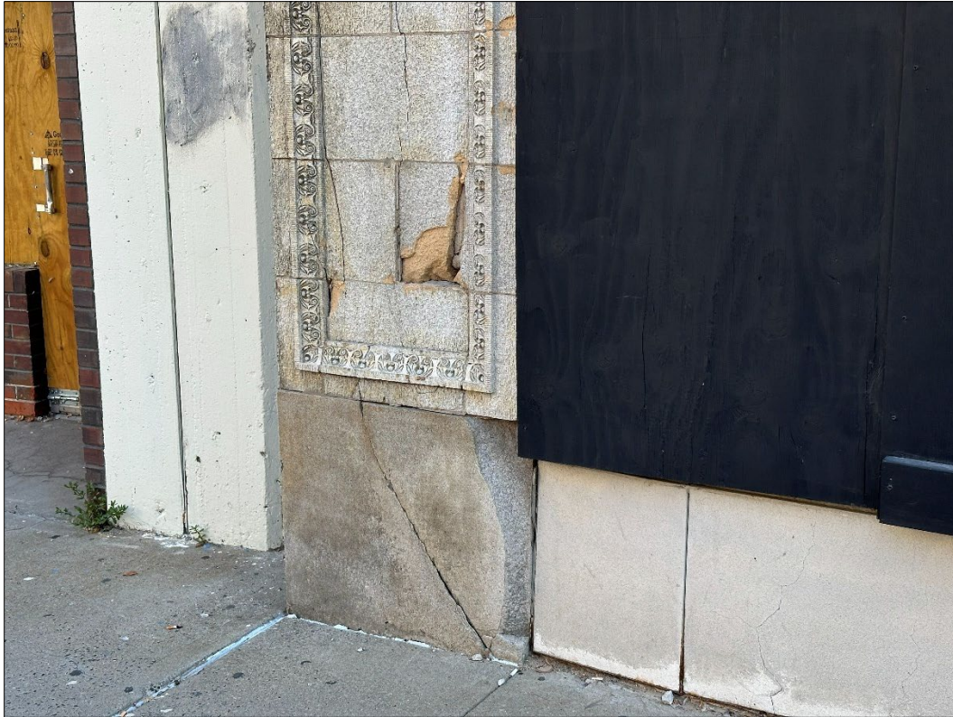
819 Walnut St – looking east – deterioration of terra cotta
