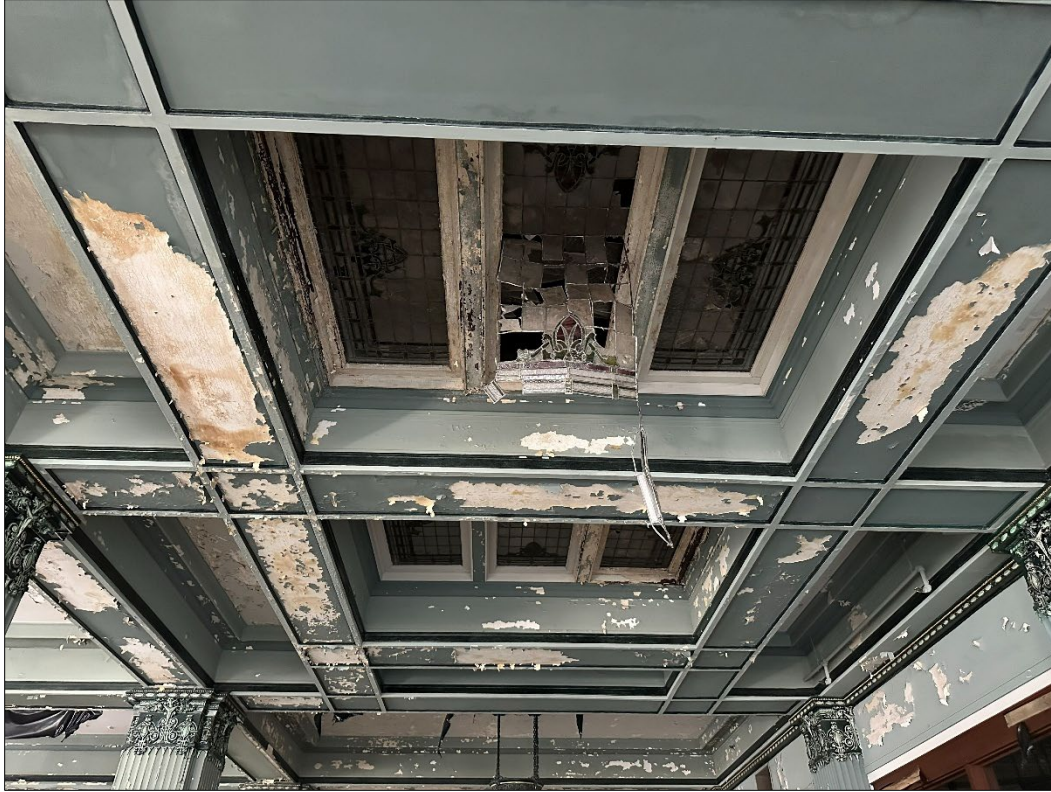
818 Grand Blvd – interior – failure of finishes; deterioration of fixtures
