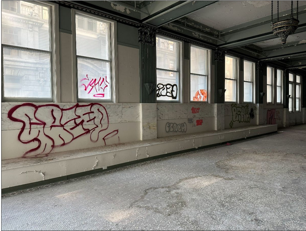
818 Grand Blvd – interior – graffiti; failure of finishes
