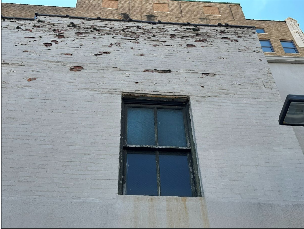
819 Walnut St – looking south – deterioration of window frame, masonry, lintel
