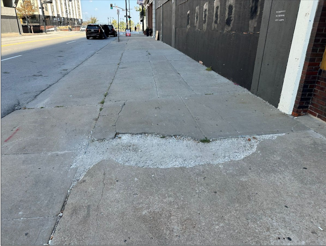
800 Grand Blvd – looking north – uneven sidewalk
