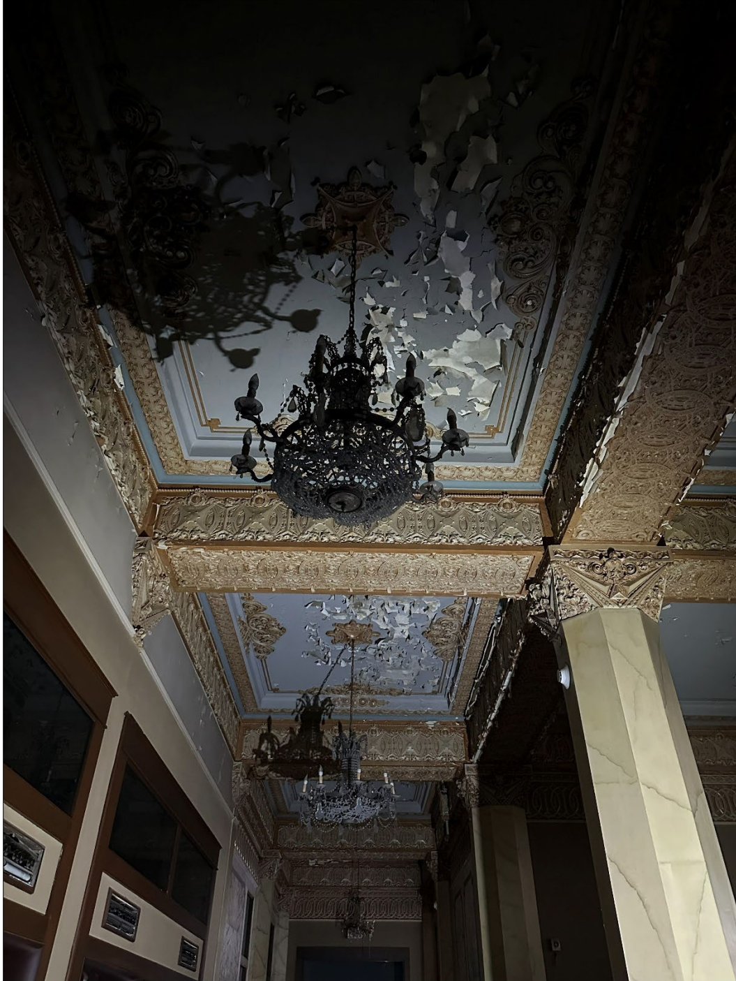
818 Grand Blvd – interior – failure of finishes
