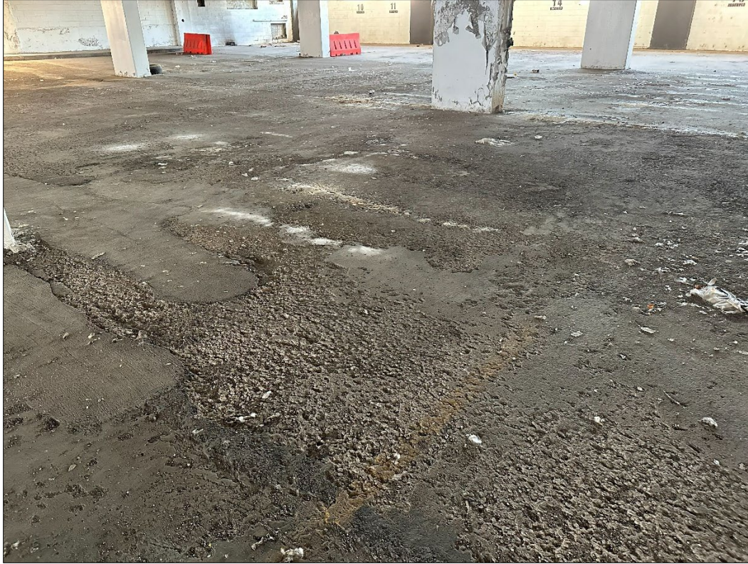
800 Grand Blvd – looking southwest – spalled concrete; failure of finishes
