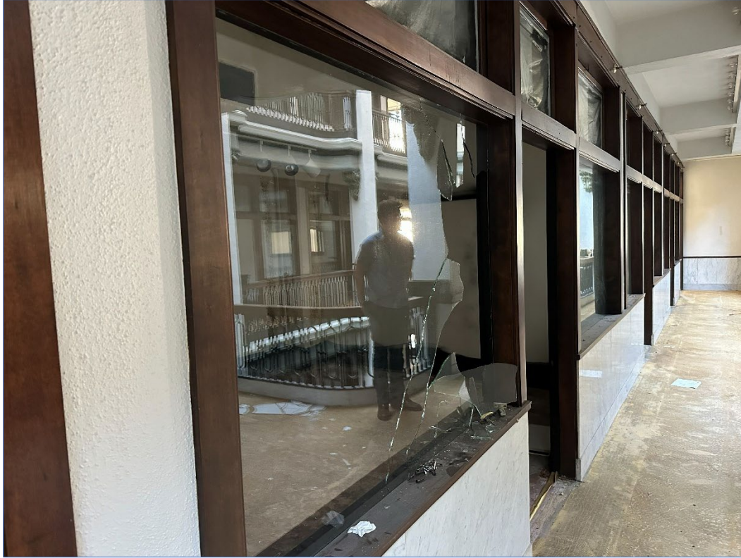
819 Walnut St – interior – broken window (vandalism)
