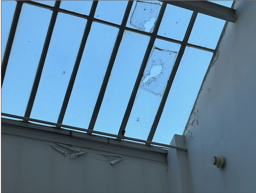
819 Walnut St – looking north – damaged glass panels in roof; failure of finishes
