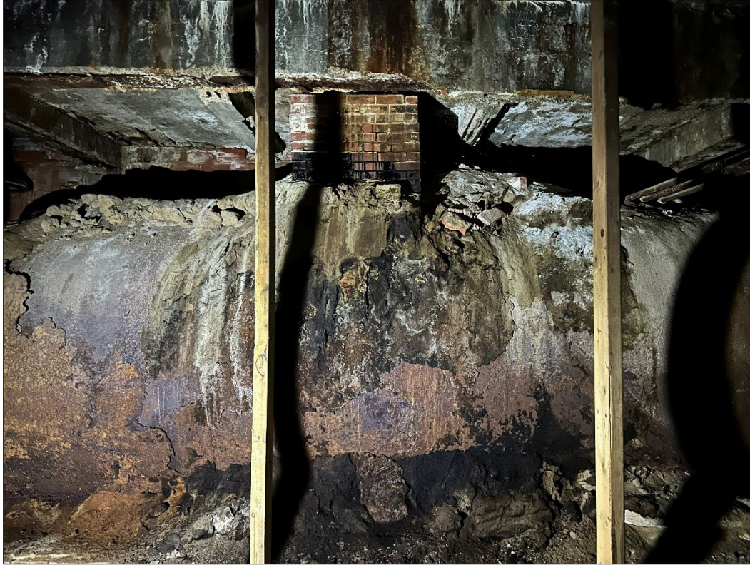
818 Grand Blvd – interior – deterioration of basement, foundation, underneath side of sidewalk
