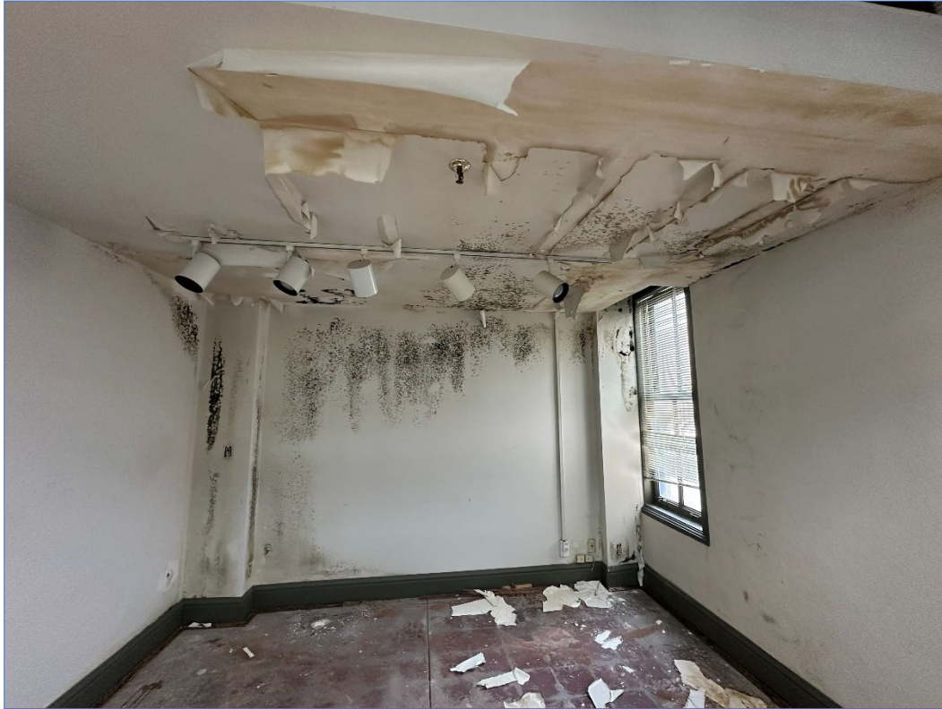
819 Walnut St – interior – mold; failure of finishes
