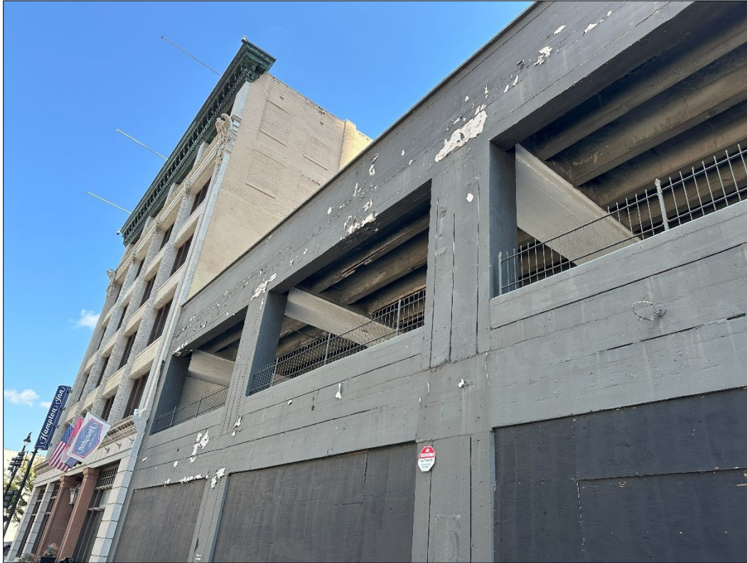
800 Grand Blvd – looking northeast – failure of finishes
