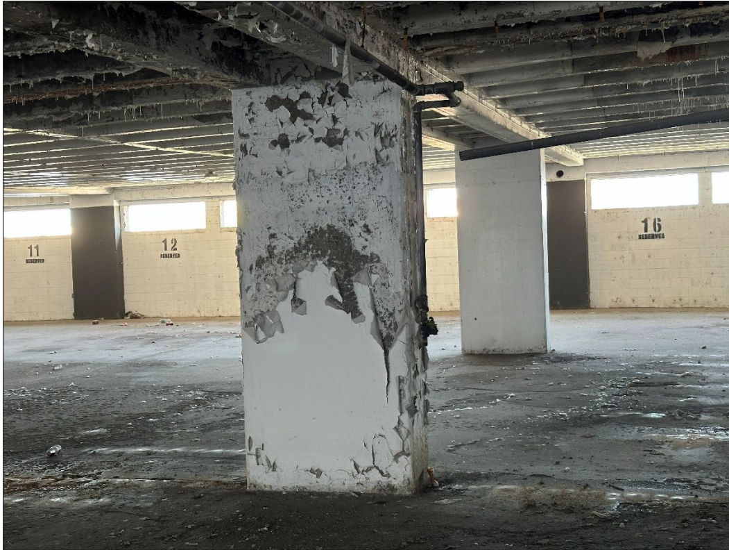
800 Grand Blvd – failure of finishes; deterioration of garage floor
