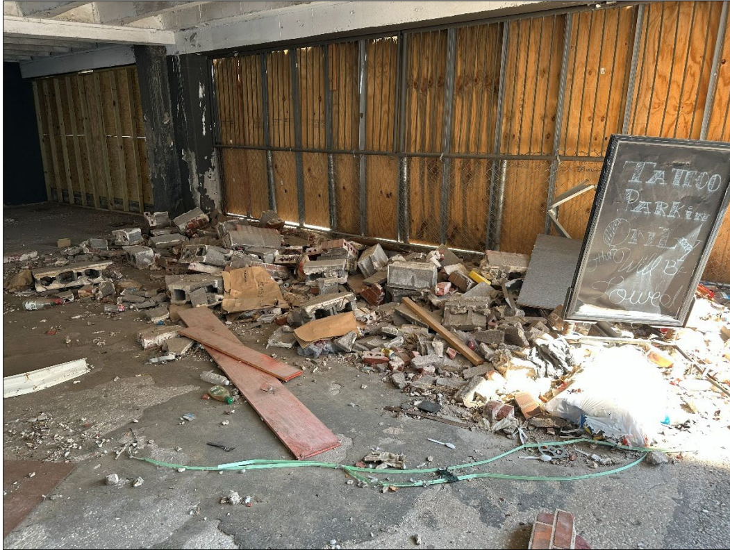
800 Grand Blvd – looking east – trash/debris; failure of finishes
