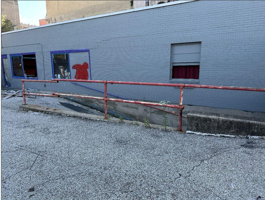
800 Blvd – looking south – deterioration of pavement, railing; broken windows; trash/debris
