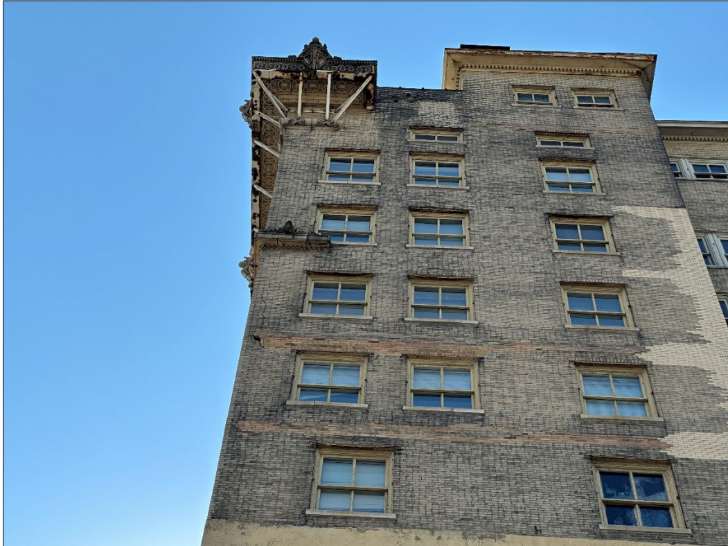
818 Grand Blvd – deterioration of steel cornice supports, masonry, and windows
