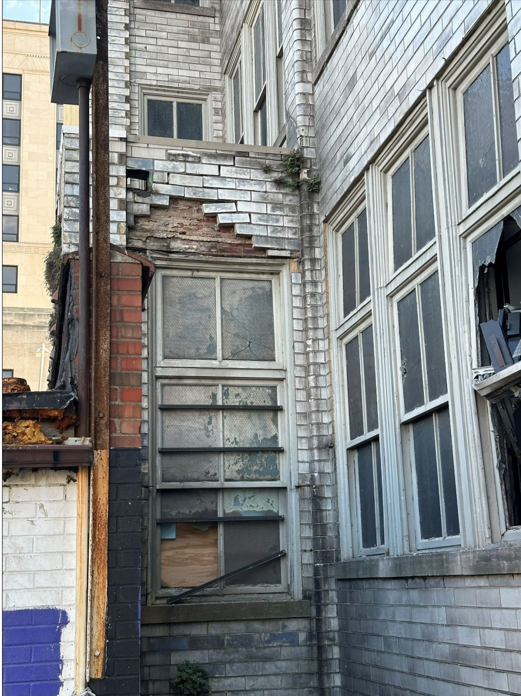
818 Grand Blvd – looking east – deterioration of brick veneer, windows, equipment
