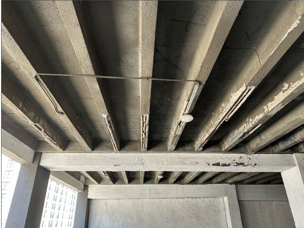
800 Grand Blvd – deterioration of garage structure; failure of finishes
