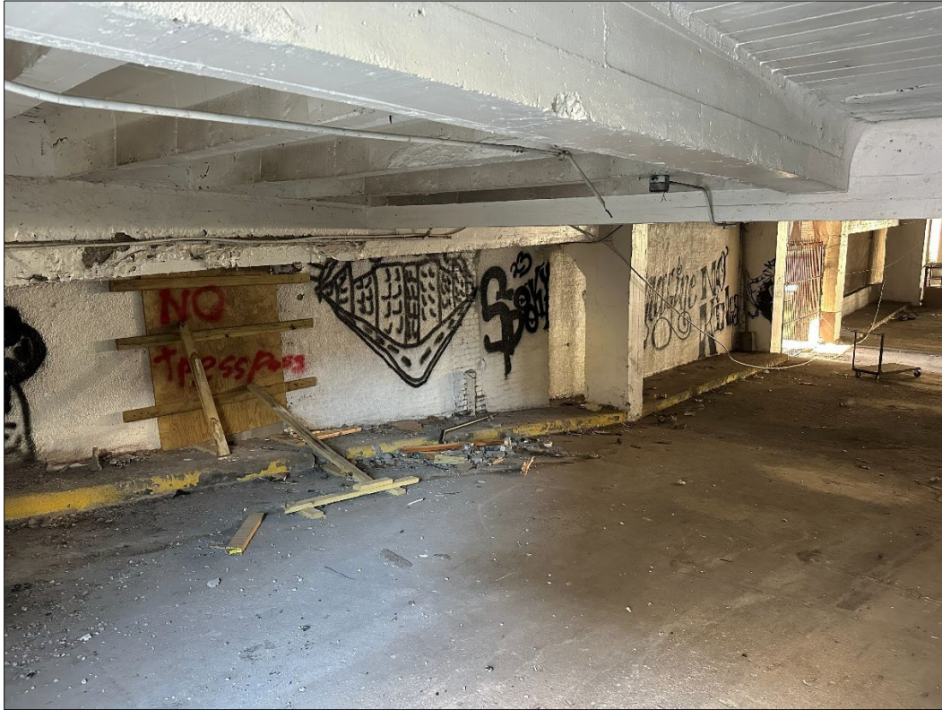
800 Grand Blvd – looking west – graffiti; trash/debris
