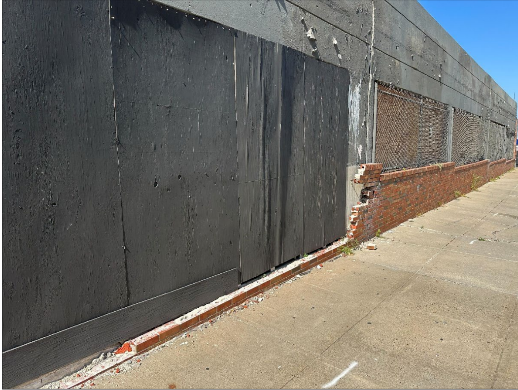
800 Grand Blvd – deterioration of brick veneer, fence
