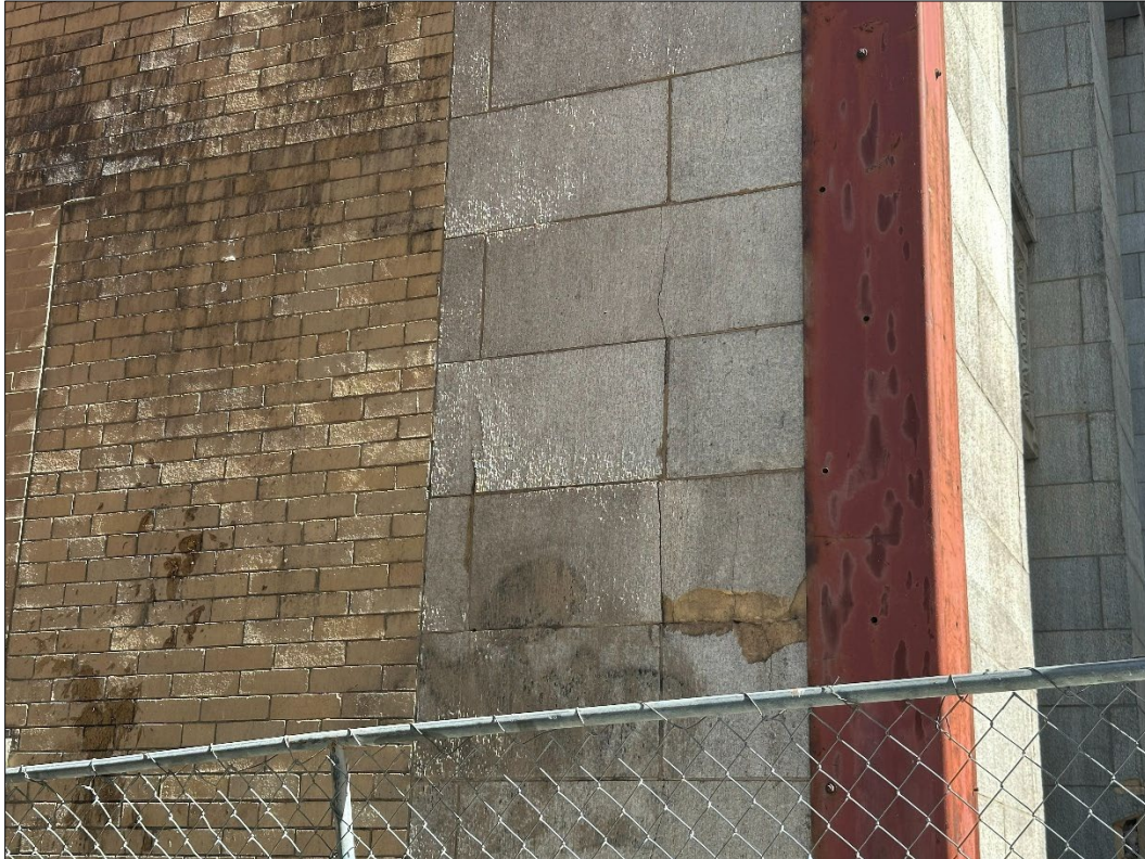
818 Grand Blvd – looking east – deterioration of brick veneer, terra cotta, and mortar joints
