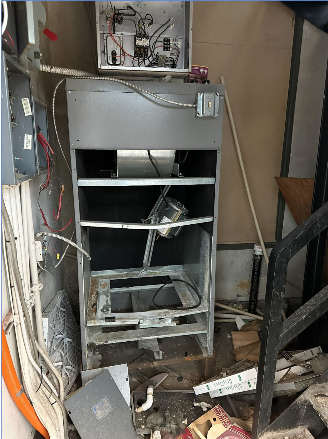
819 Walnut St – interior – missing HVAC equipment components
