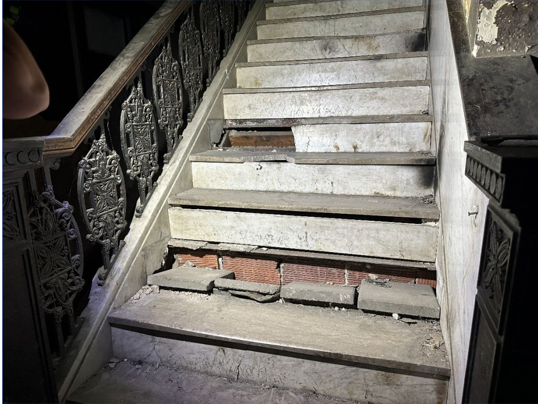
818 Grand Blvd – interior – deteriorated/broken stairs
