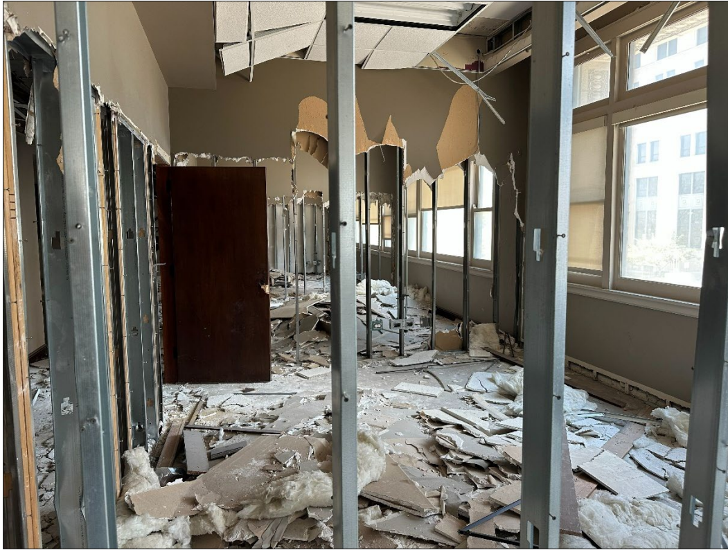
818 Grand Blvd – interior – trash/debris
