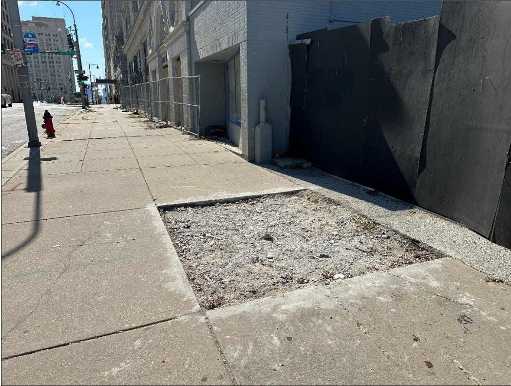
800 Grand Blvd – looking south – uneven sidewalk
