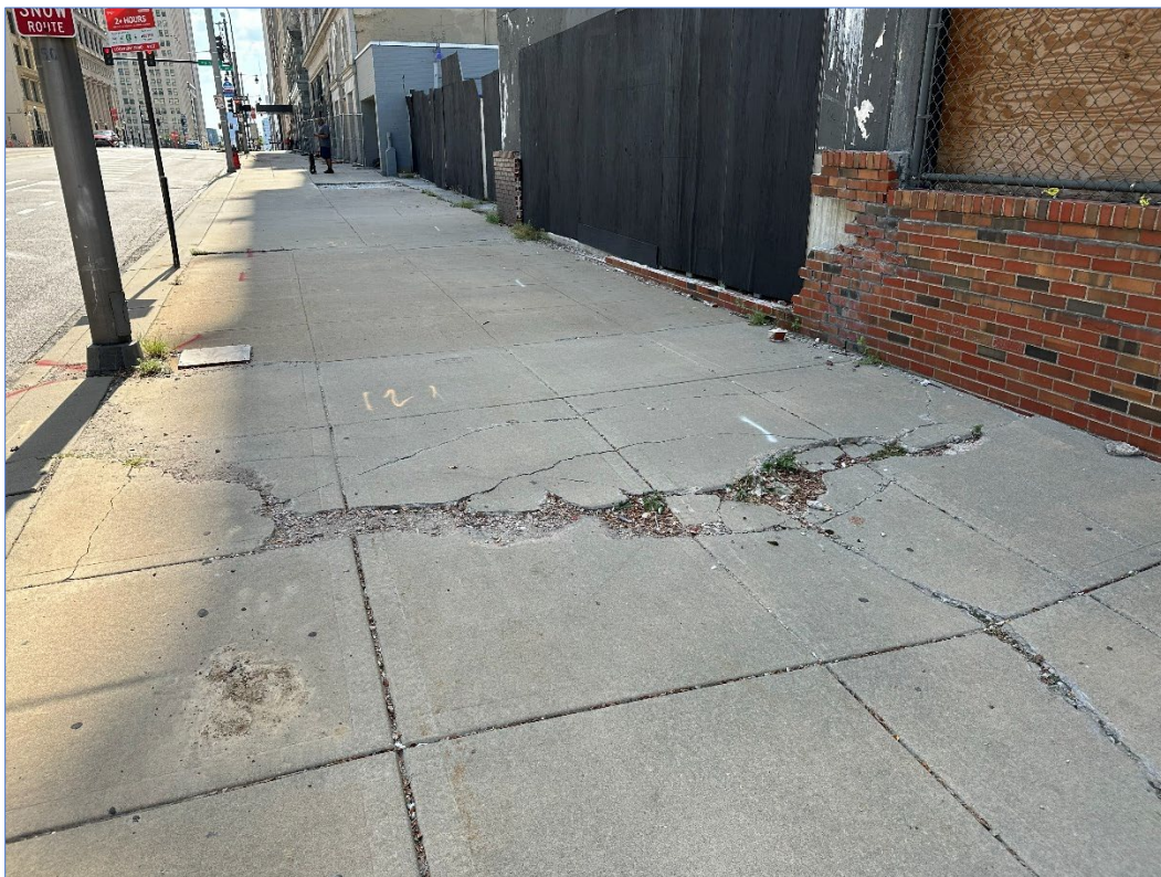
800 Grand Blvd – looking south – deterioration of sidewalk/uneven pavement
