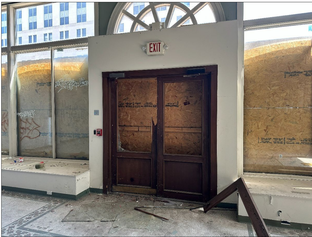
818 Grand Blvd – interior – broken glass; debris
