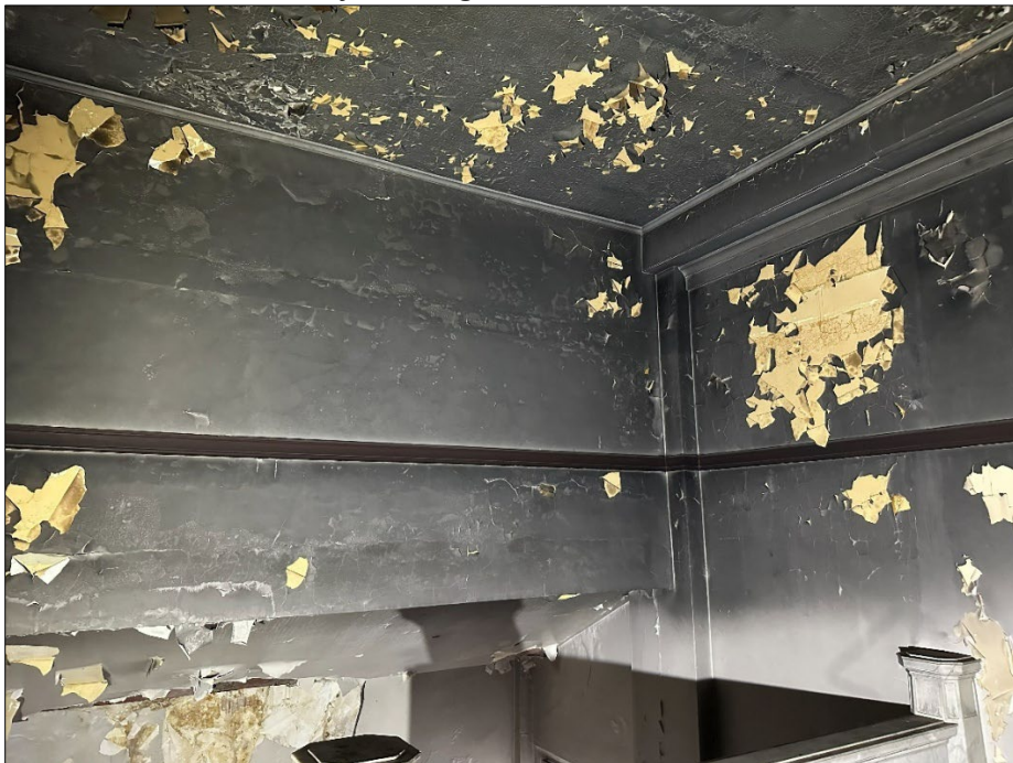
800 Grand Blvd – interior – fire damage
