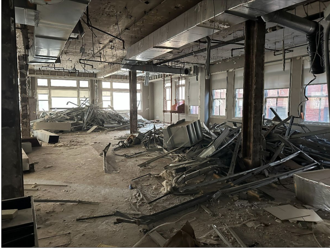
818 Grand Blvd – interior – trash/debris; disconnected and nonfunctioning building systems
