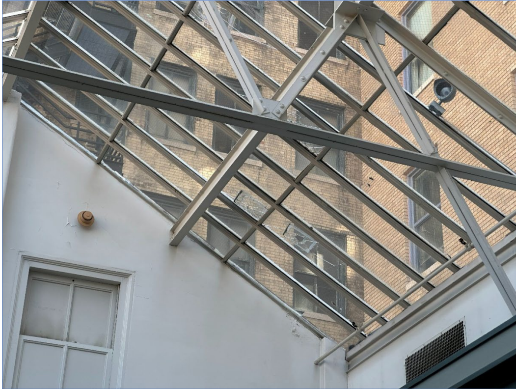
819 Walnut St – interior – broken glass panels in roof
