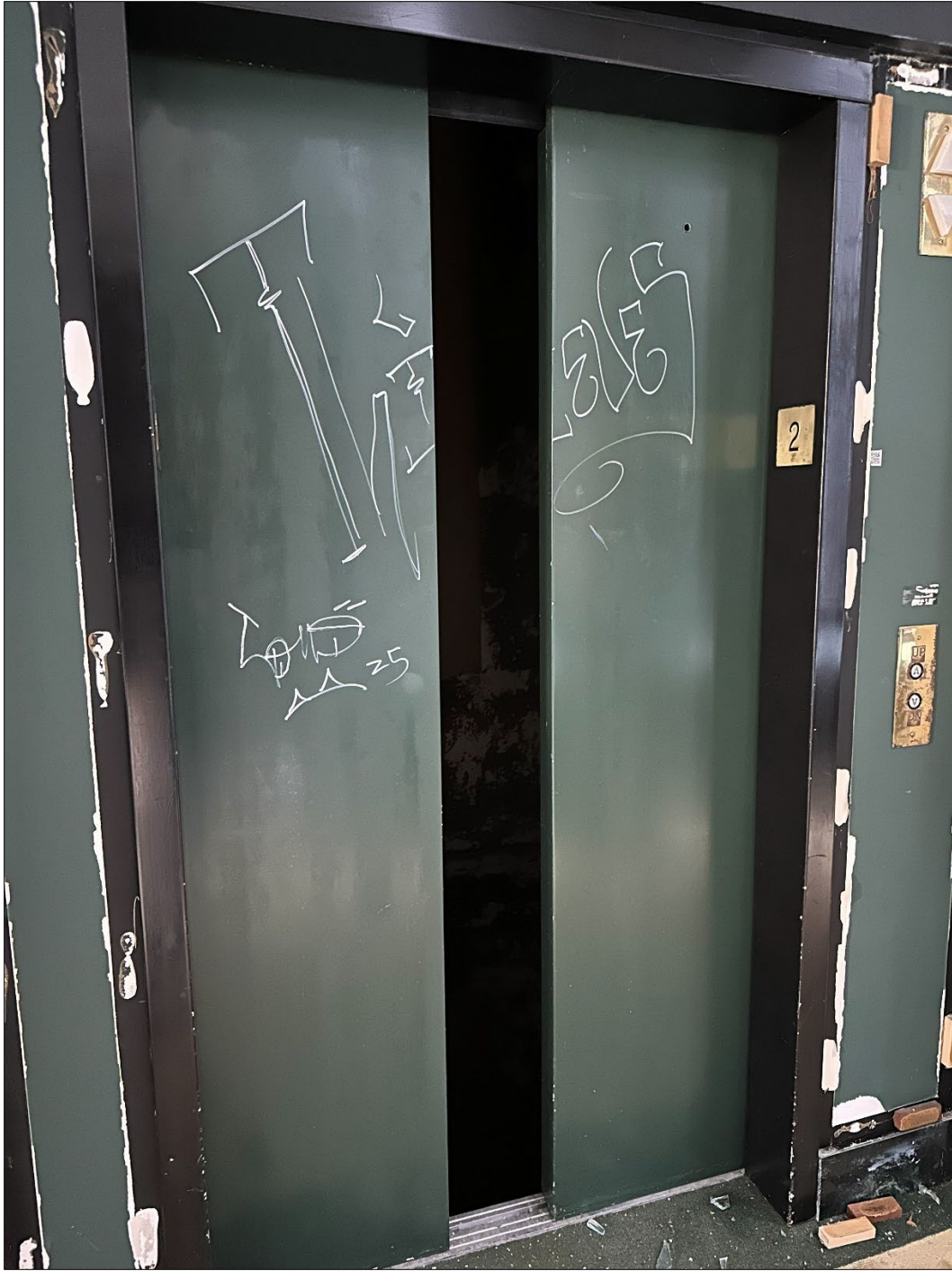
819 Walnut St – interior – open elevator; graffiti
