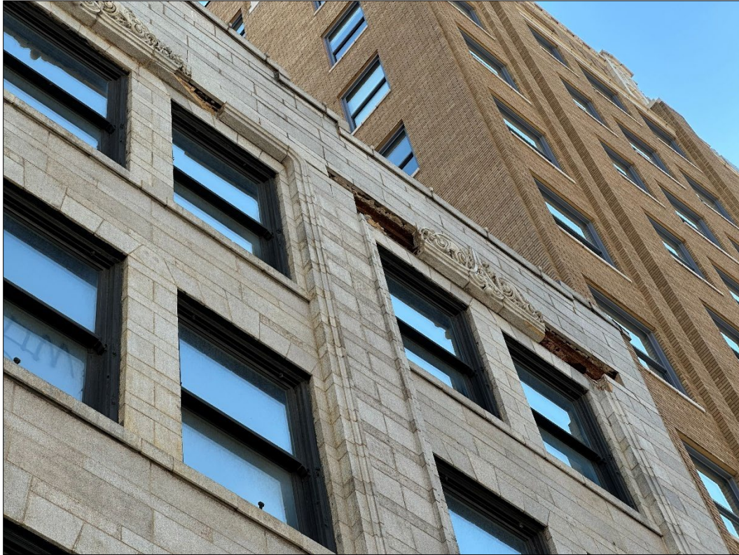
819 Walnut St – looking east – deterioration of terra cotta mouldings
