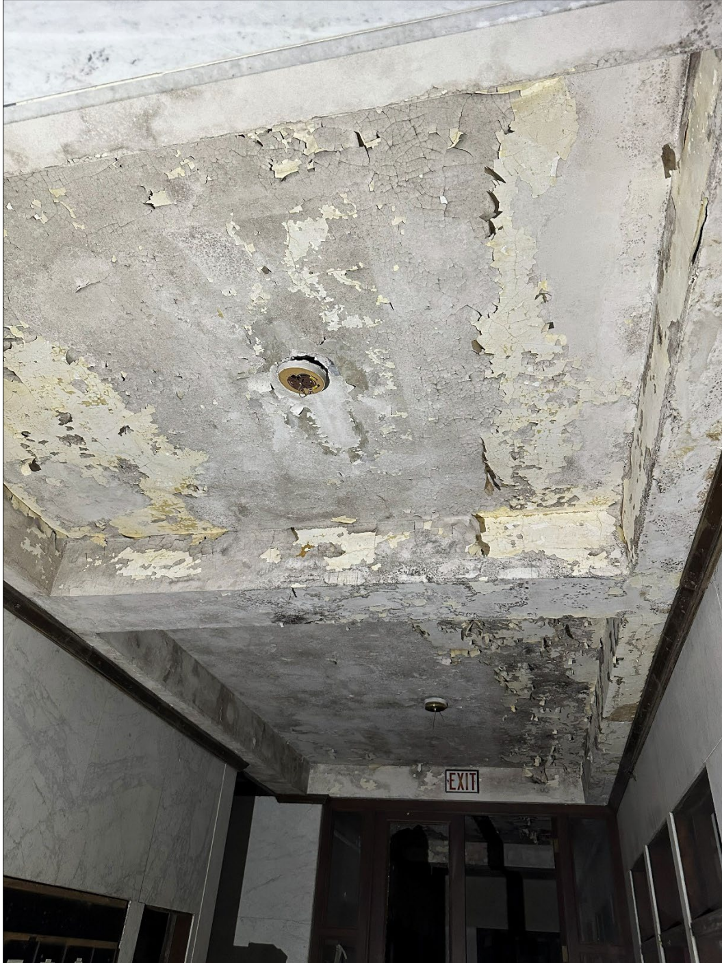
818 Grand Blvd – interior – failure of finishes
