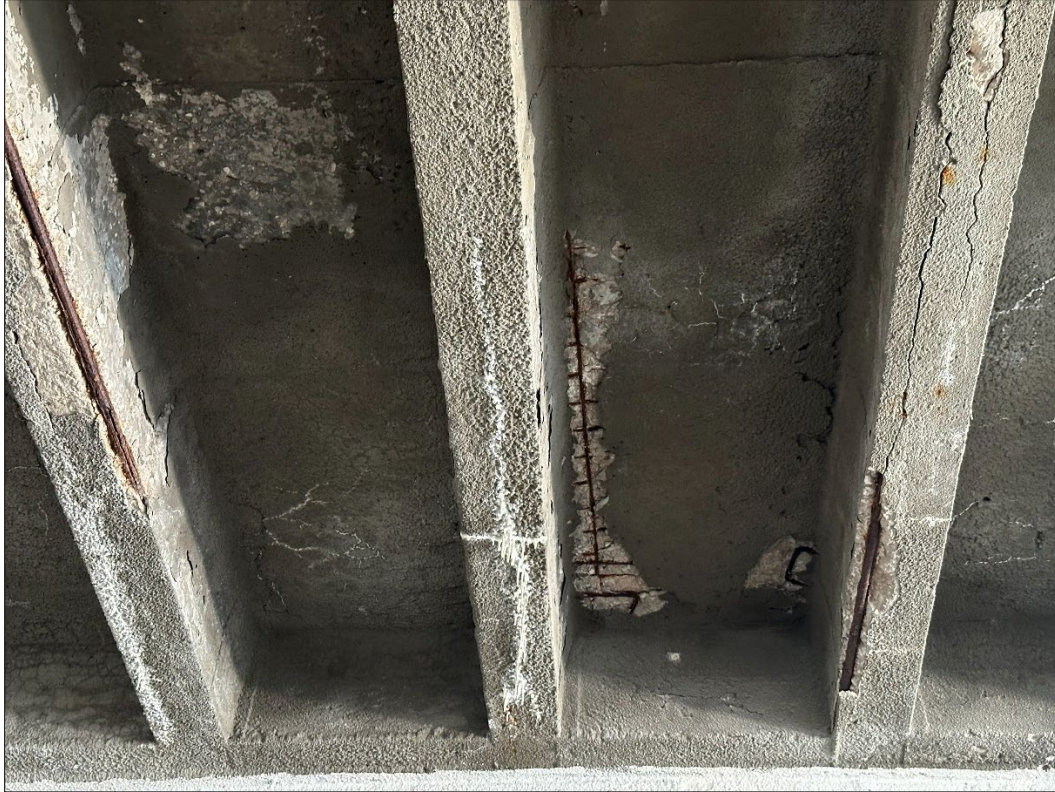
800 Grand Blvd – deterioration of garage structure
