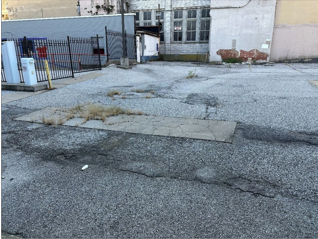
800 Grand Blvd – looking south – deterioration of pavement
