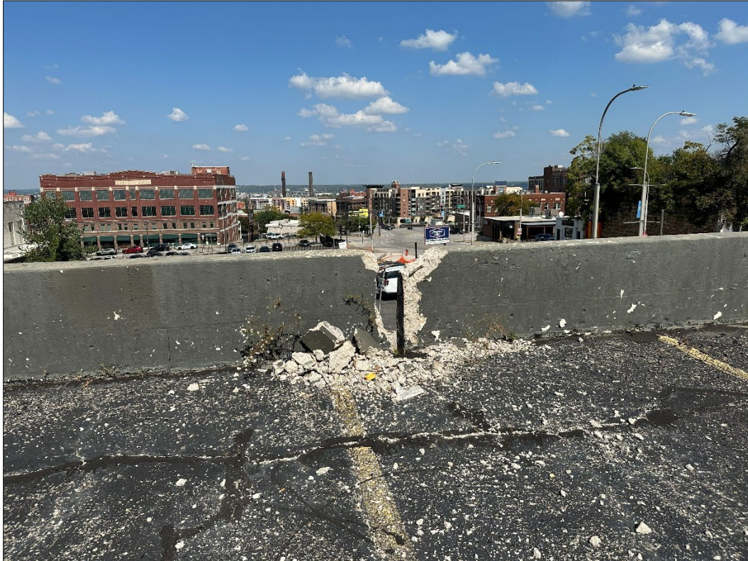
800 Grand Blvd – looking north – deterioration of pavement, wall
