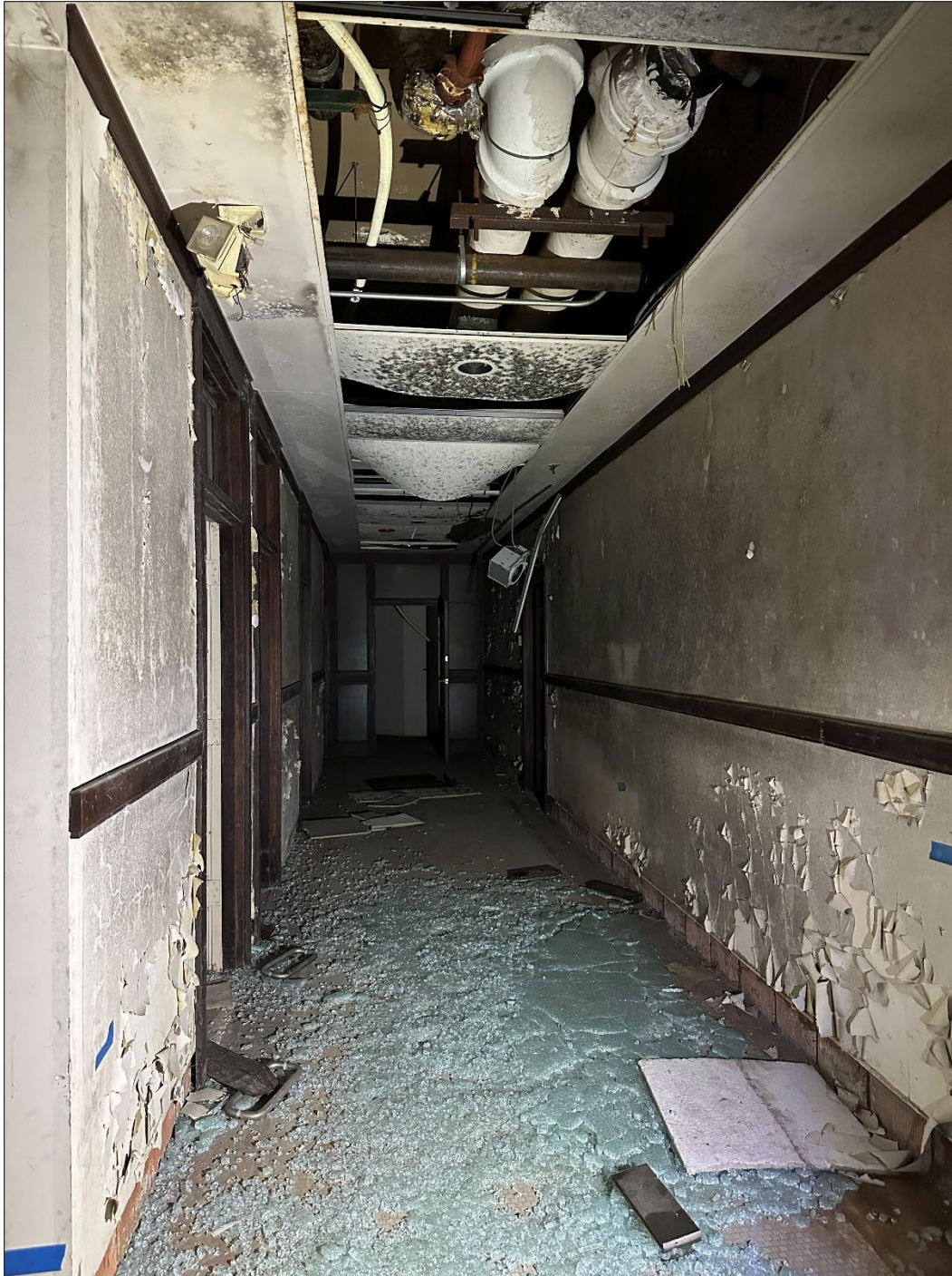
818 Grand Blvd – interior – broken glass on floor; failure of finishes
