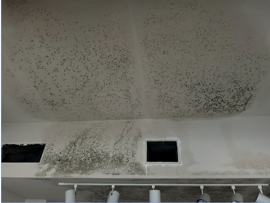
819 Walnut St – interior – mold; failure of finishes
