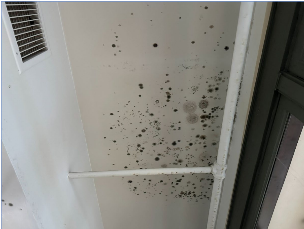
819 Walnut St – interior – mold
