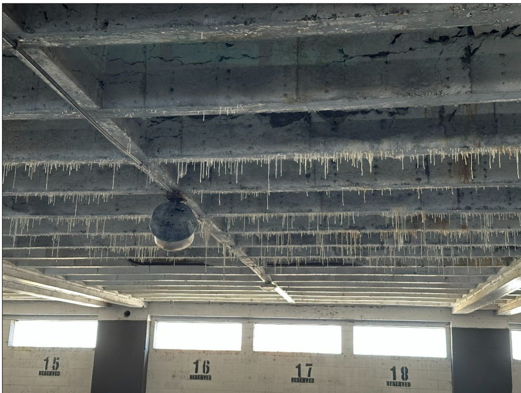
800 Grand Blvd – looking north – presence of calthemites due to water seeping through concrete beams
