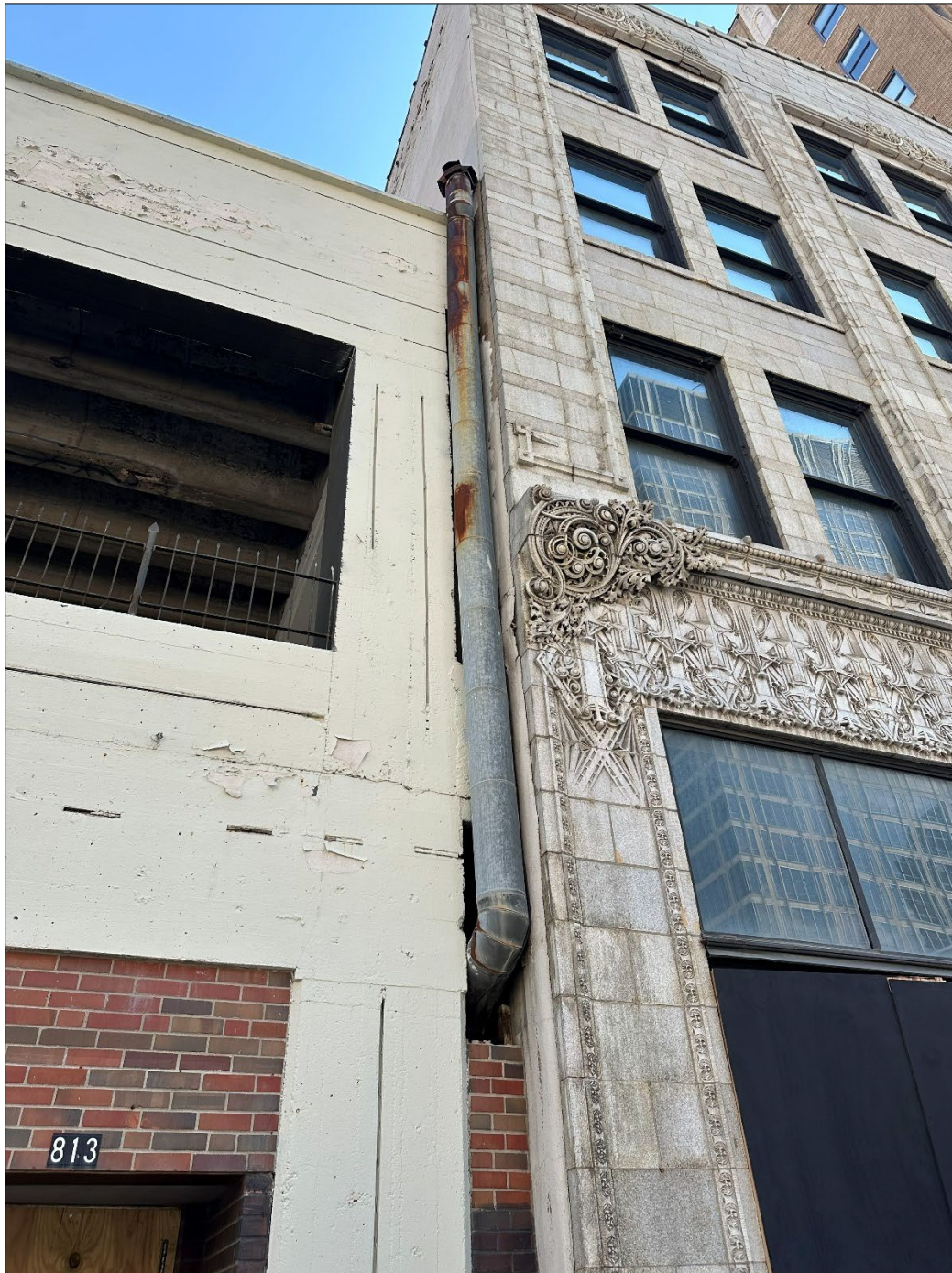
800 Grand Blvd – looking east – rusting mechanical equipment
