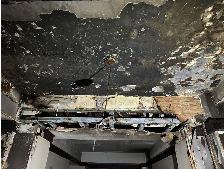
800 Grand Blvd – interior – fire damage
