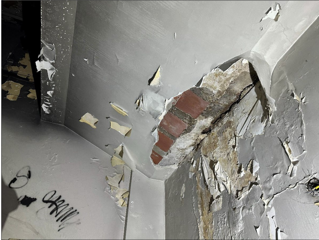
818 Grand Blvd – interior – failure of finishes; graffiti
