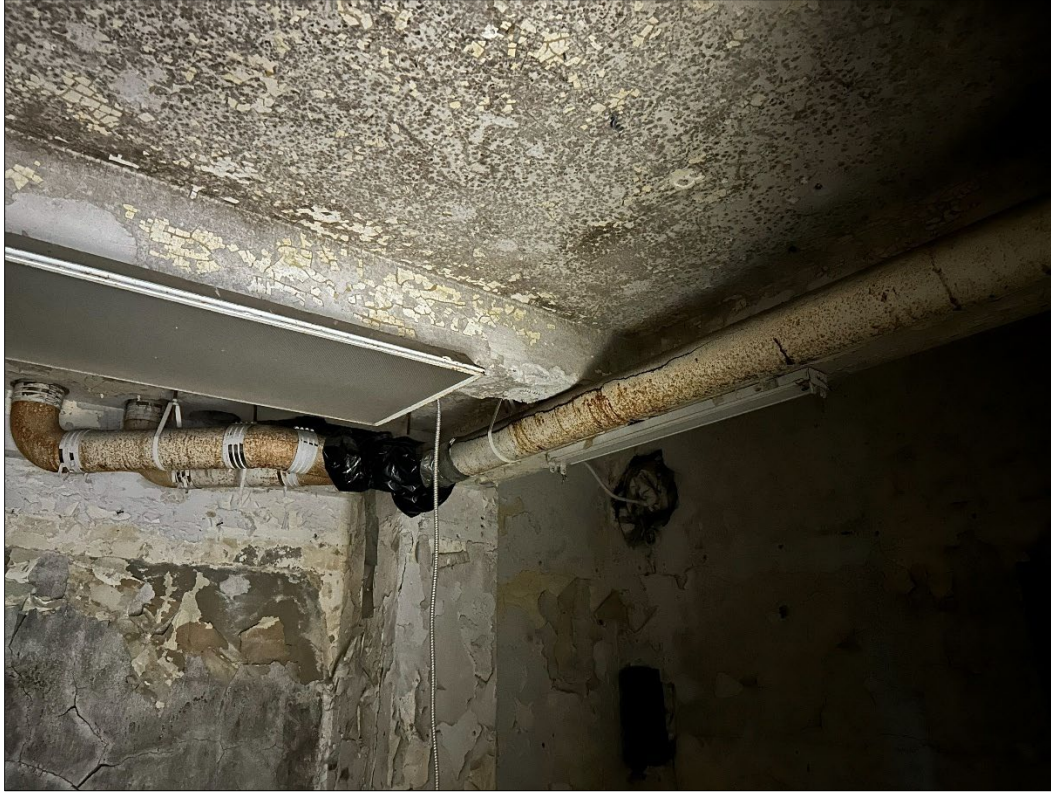
818 Grand Blvd – interior – failure of finishes; suspect pipe wrap
