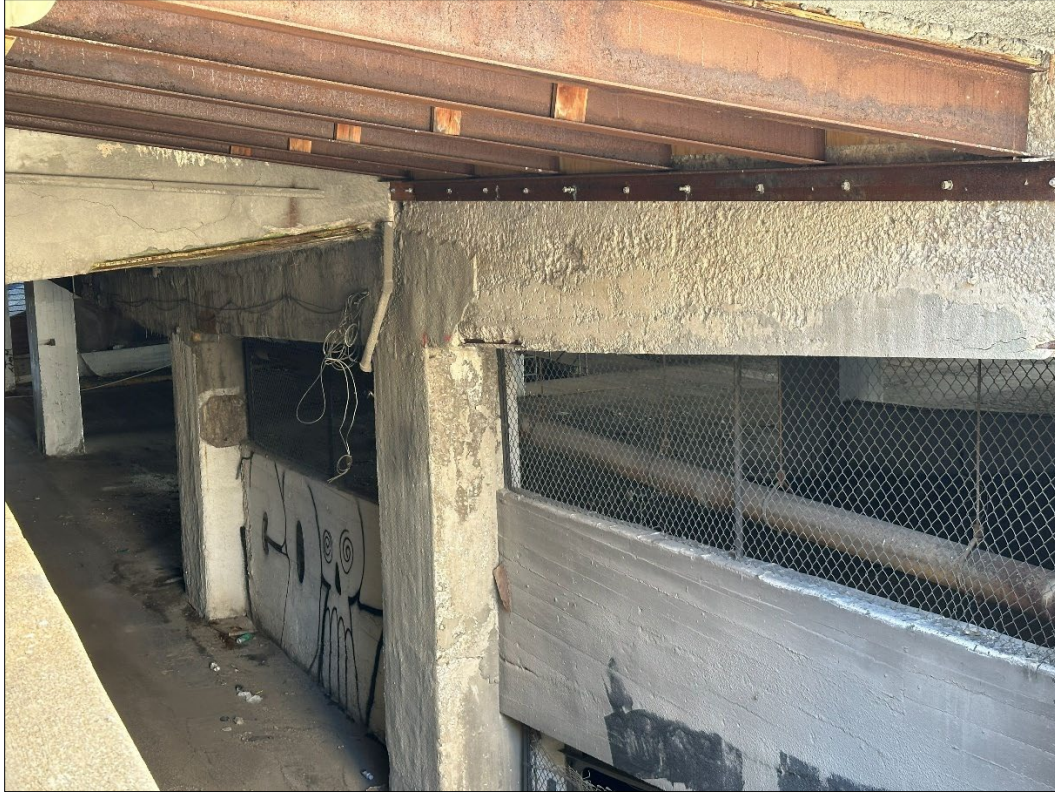
800 Grand Blvd – looking west – spalling concrete; graffiti
