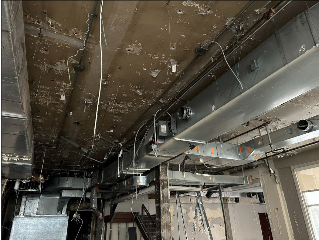
818 Grand Blvd – interior – disconnected, nonfunctioning building systems
