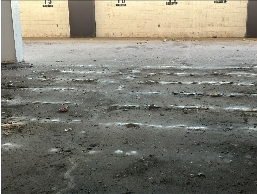
800 Grand Blvd – looking north – deterioration of parking garage floor
