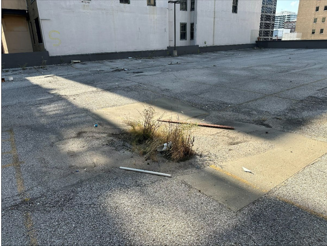
800 Grand Blvd – looking southwest – deterioration of pavement
