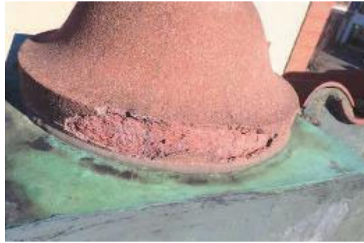
Crumbled cornice Building 18/Block L
