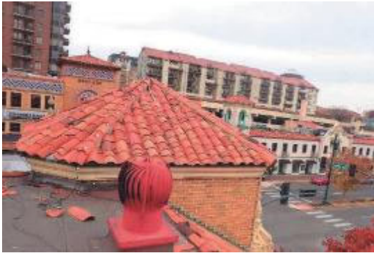
Broken and fallen tile Building 9/Block H
