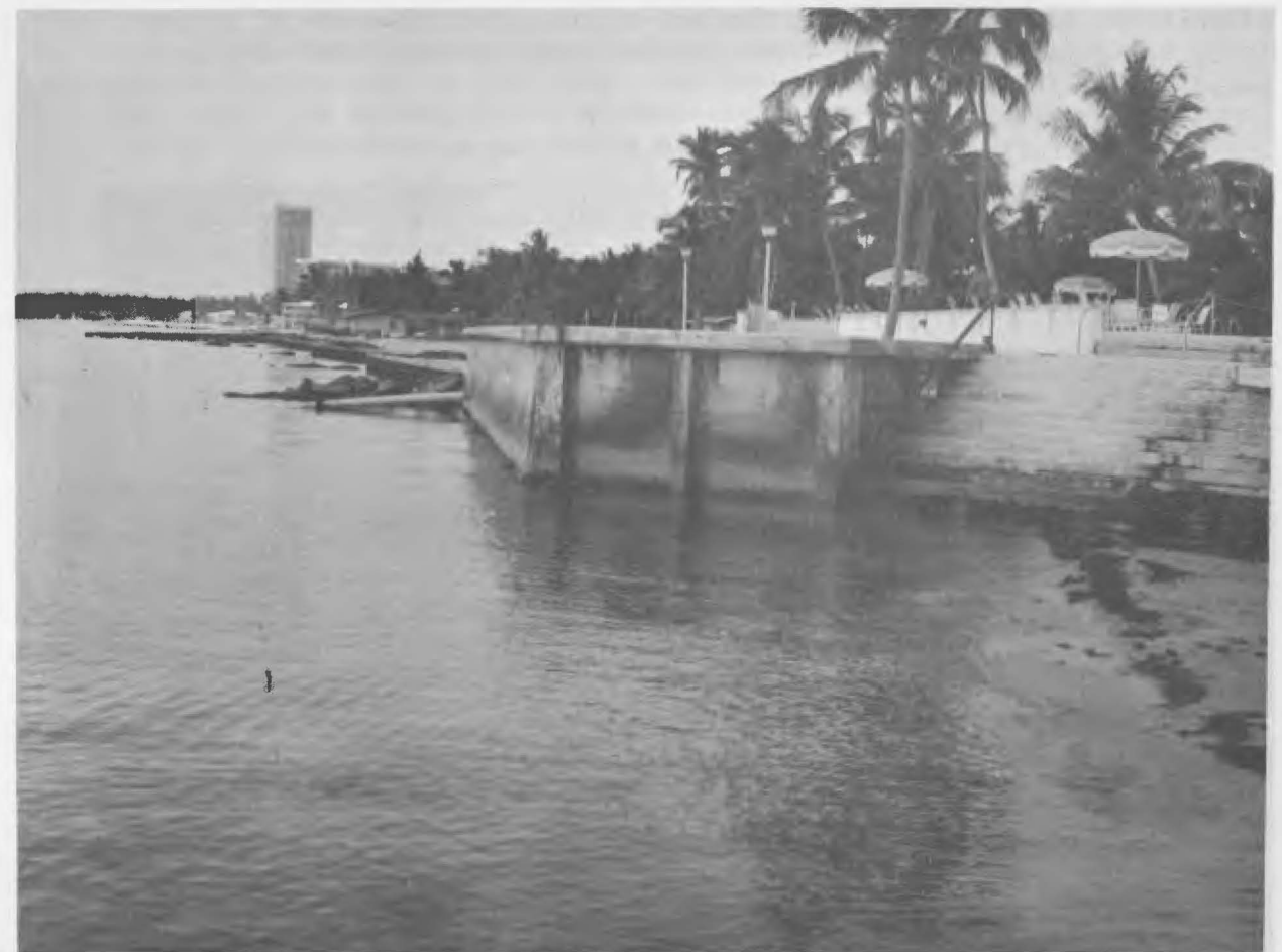
Key Biscayne (Dade County) - Problem area north of Cape Florida State Park (1971)
