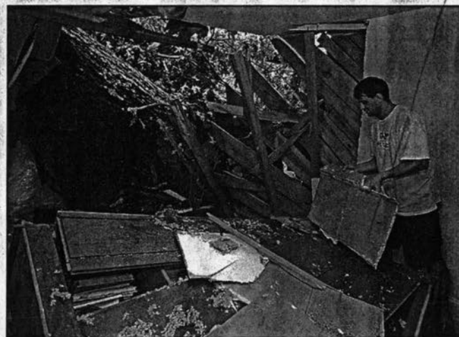
Raleigh, Friday: The storm brought nature into people's lives in a very personal and frightening way. Etienne Volat removed broken plaster from a bedroom in his home on Kenmore Drive after a large oak tree smashed through the roof.
