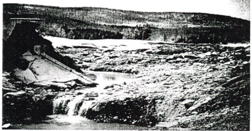
Dam failure at Meadow Pond in Alton, NH
