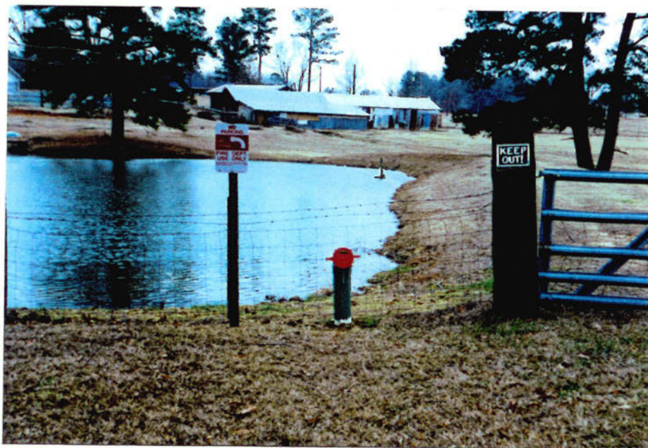
A dry fire hydrant.
