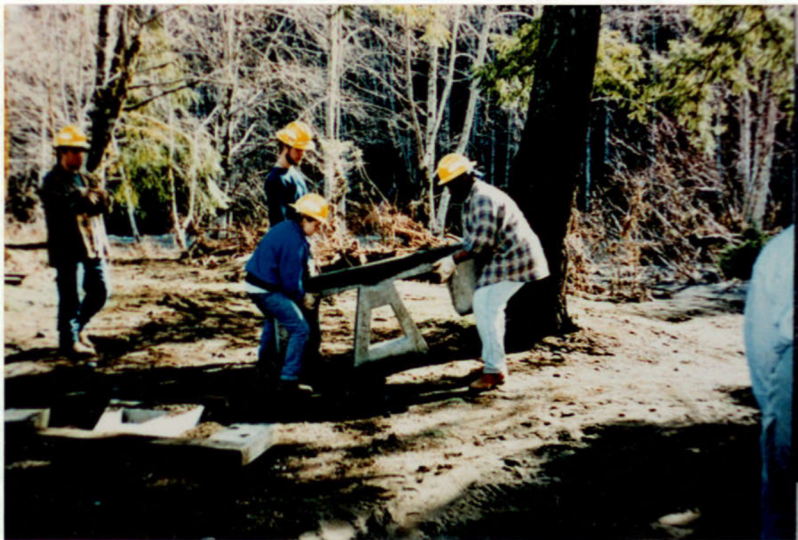
Campground maintenance and preparation is necessary before peak camping season begins. Here Members set in durable concrete picnic tables at Hamma Hamma Campground, Hood Canal Ranger District, Olympic National Forest.
