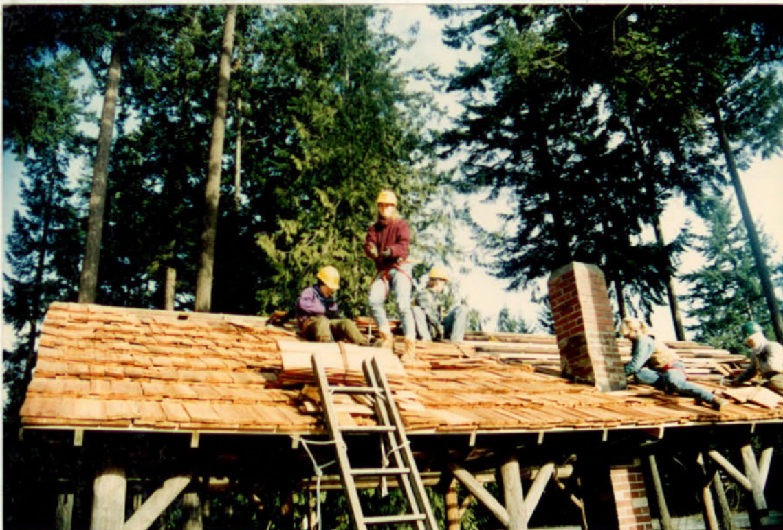
AmeriCorps members have participated in many Jefferson and Clallam County projects. Here members are re-roofing the Chimacum Community Center picnic shelter.
