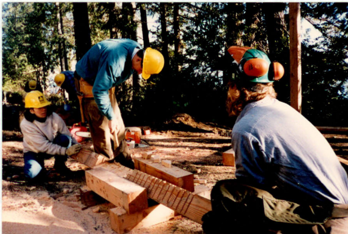
Interpretive trails are constructed near popular campgrounds to educate campers about watersheds, wildlife, and ecosystem dynamics. Members construct kiosk (information boards) at Seal Rock Campground, Quilcene Ranger District, Olympic National Forest.
