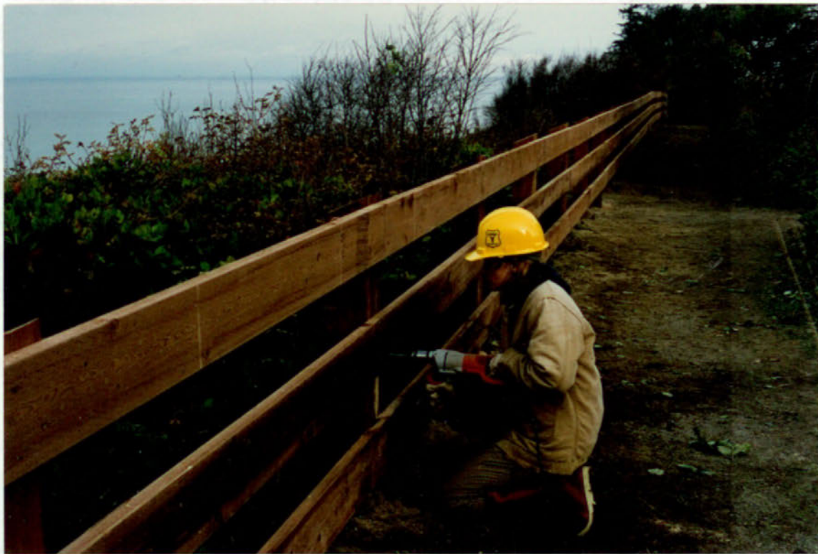
Fences along critical bluffs have been constructed as an erosion control method. This 1200 foot fence was built in the Dungeness Campground, a Clallam County Park.
