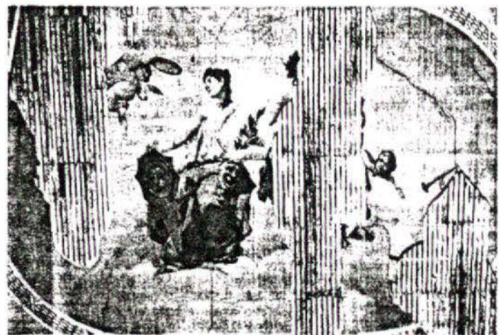
Painting on the Colonial Theater ceiling was damaged by a roof leak.
