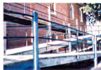
Retrofitting can be inadequate.
